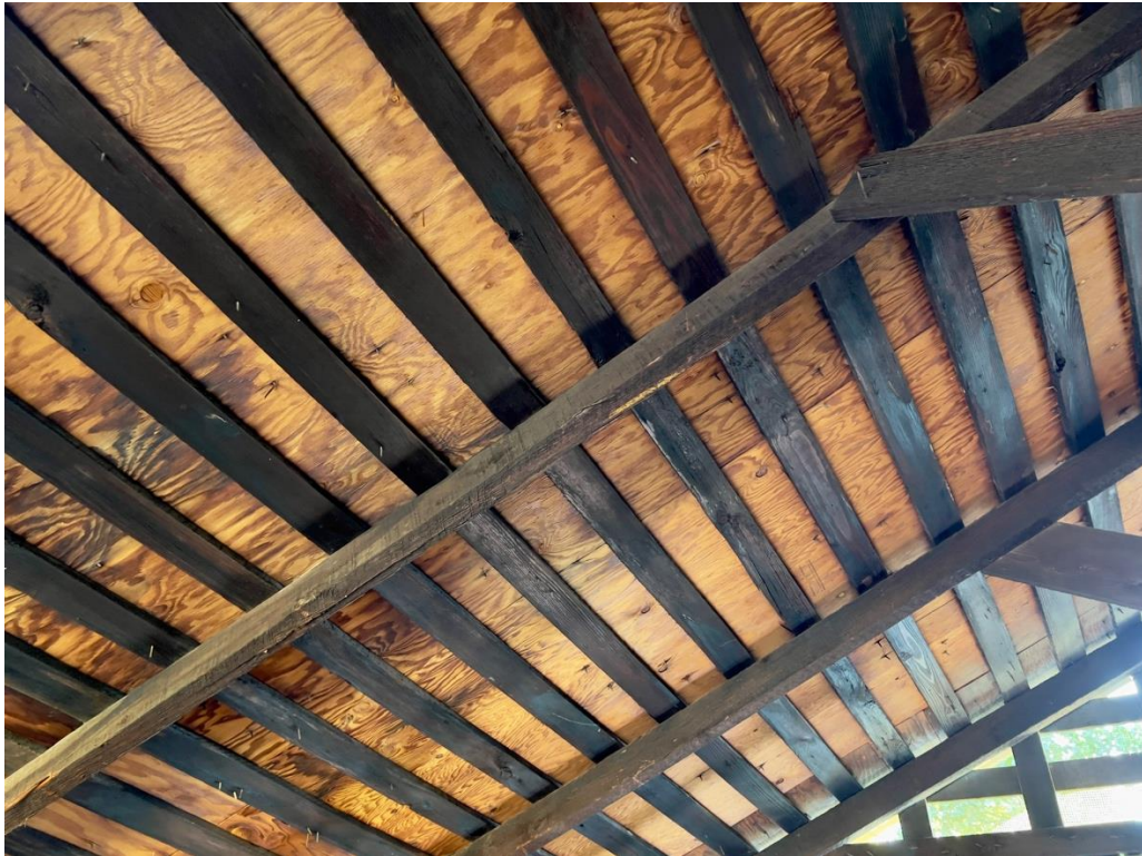
Broken joists and widely spaced rafters
