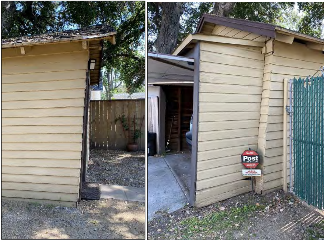
Original garage structure needs to be straightened and the frame needs to be strengthened with additional bracing.
