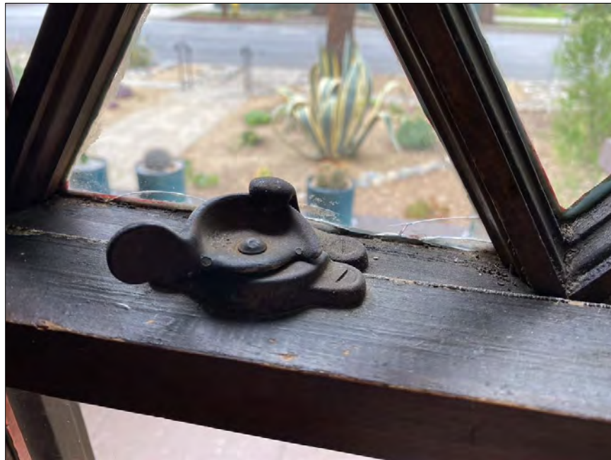
Double hung windows need to replace missing sash cords and repair broken/cracked glass.
