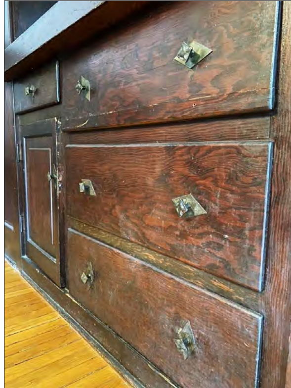
Built-in cabinetry in the dining room needs to be repaired and refinished.
