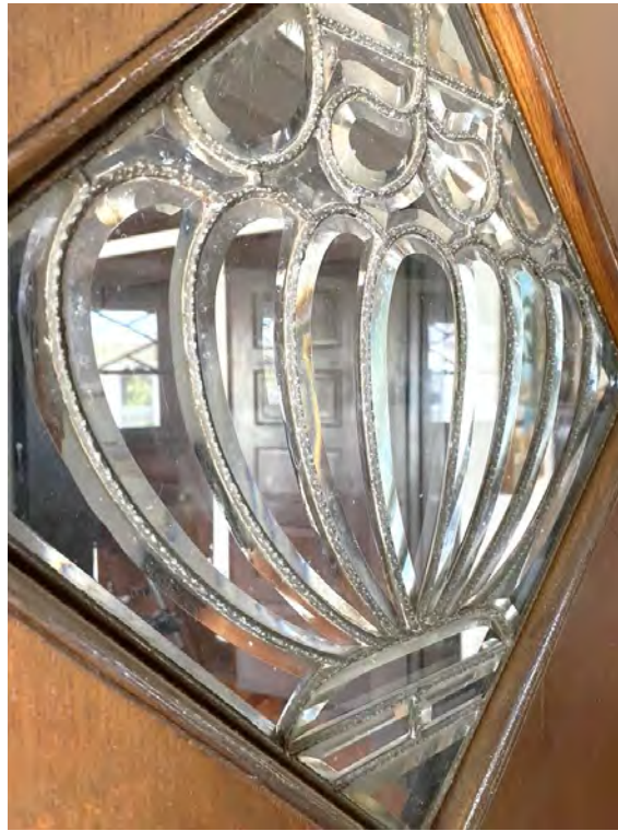
Corrosion to the leaded glass window on the front door and hardware needs to be restored.
