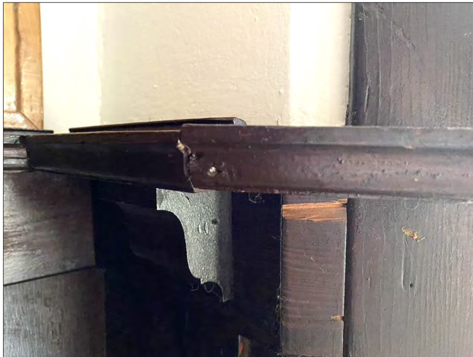
Broken pieces of wall galley shelves in the dining room to be restored.
