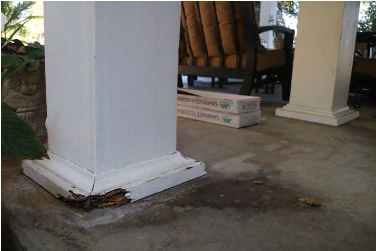
Figure 5 Detail of porch column and deterioration at base, 335 Monterey Road
