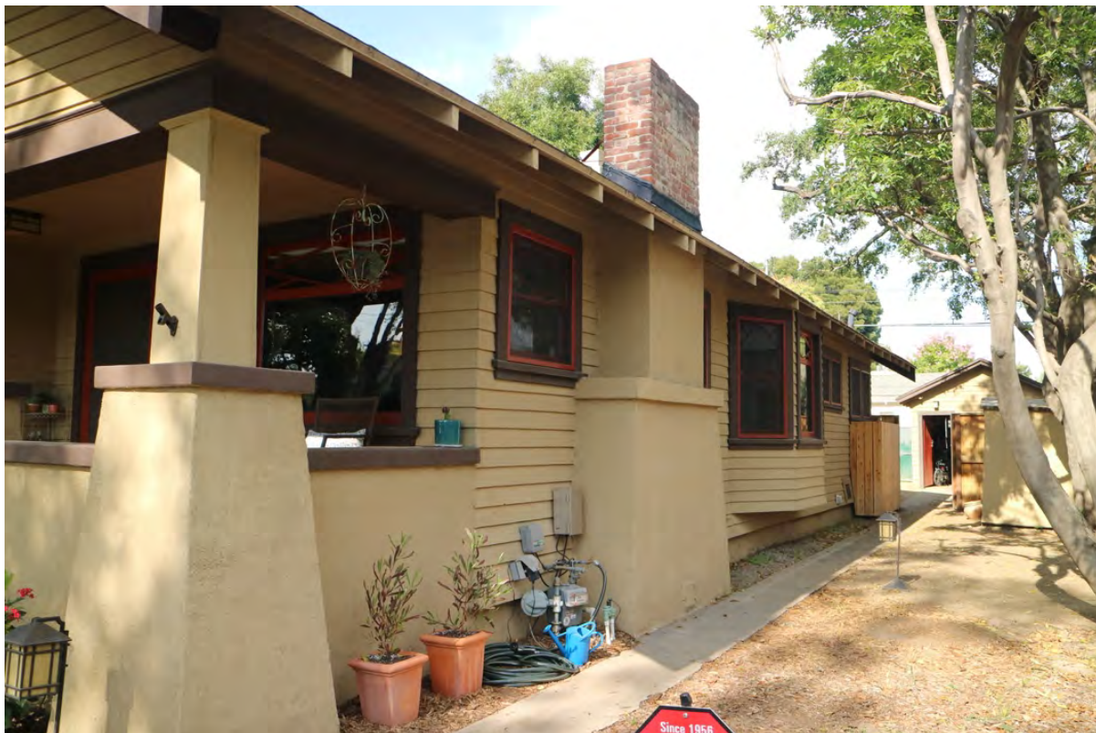
Figure 14 Overview of roof and chimney, condition and repair issues, south elevation
