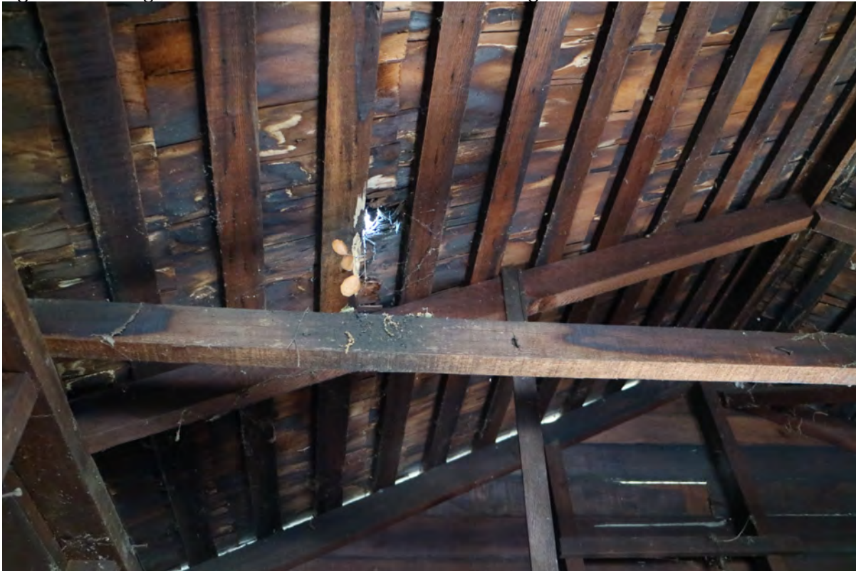
Figure 9 Garage roof, detail, shows hole in roof sheathing
