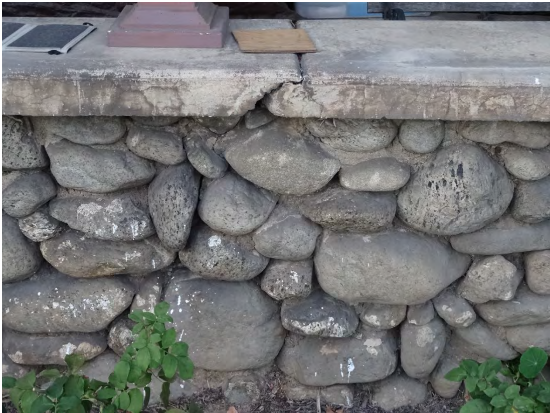
Multiple cracks in the stone porch wall
