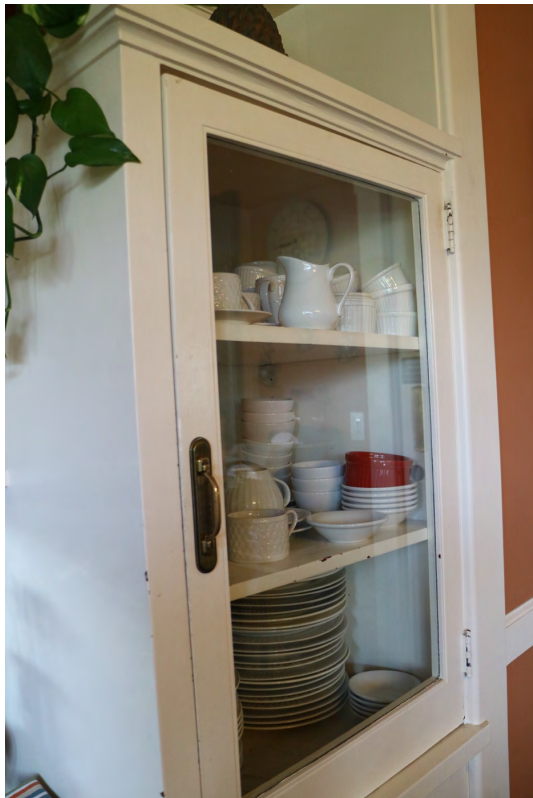
Figure 29 Interior cabinetry; overpainting has led to poorly fastening cabinets
