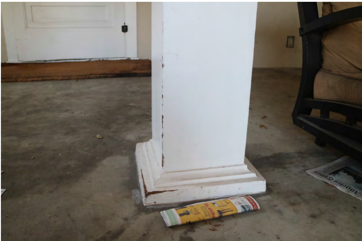
Figure 4 Detail of porch column and deterioration at base, 335 Monterey Road
