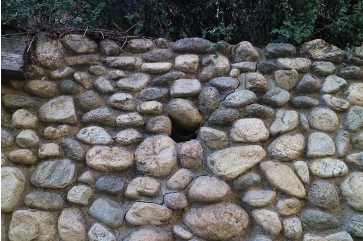
Figure 9 Detail, cracking mortar of arroyo stone wall (north perspective)
