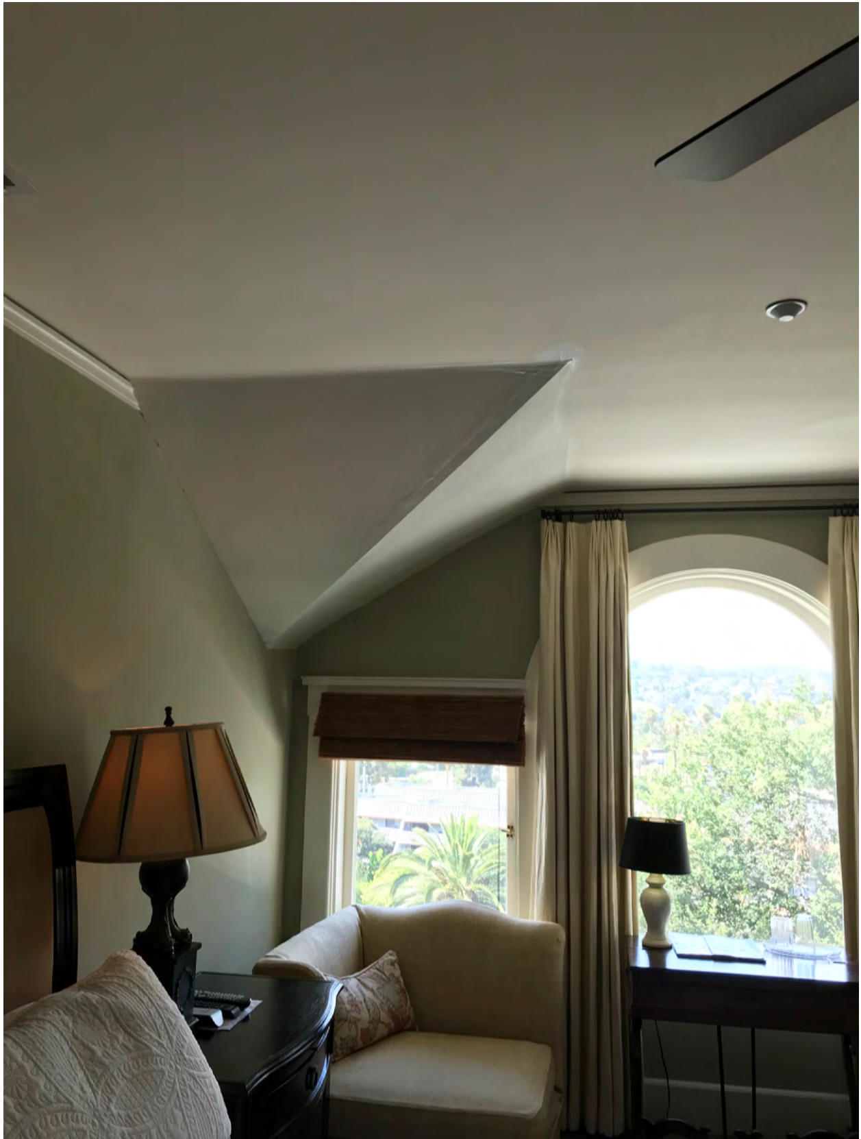
Figure 27 Interior, guestroom with leaking ceiling during rains
