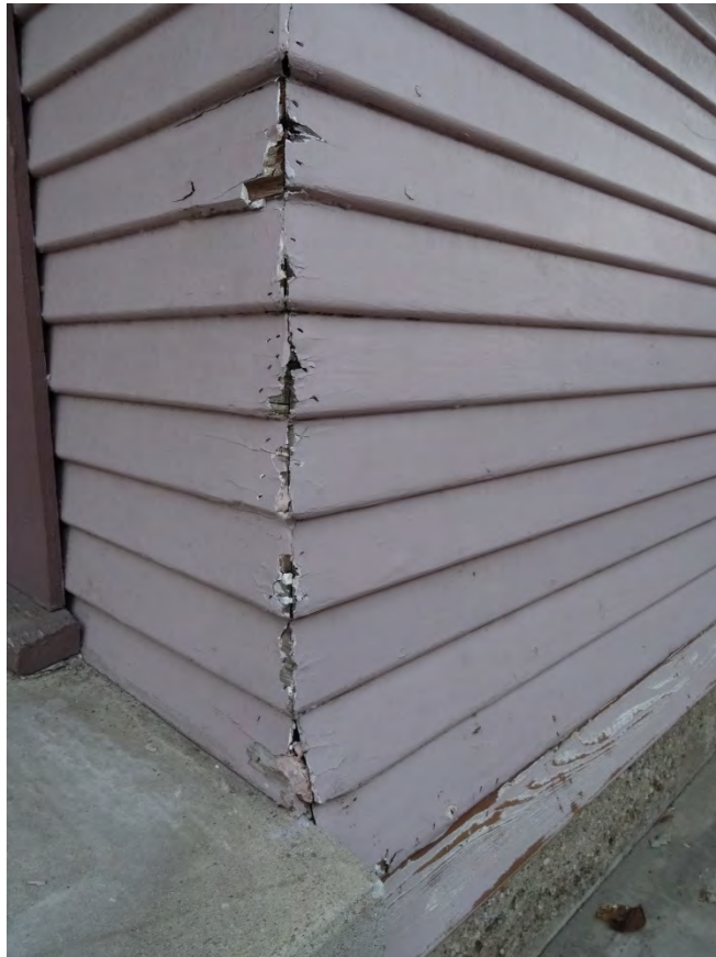
Deteriorating front gable fascia and wood siding
