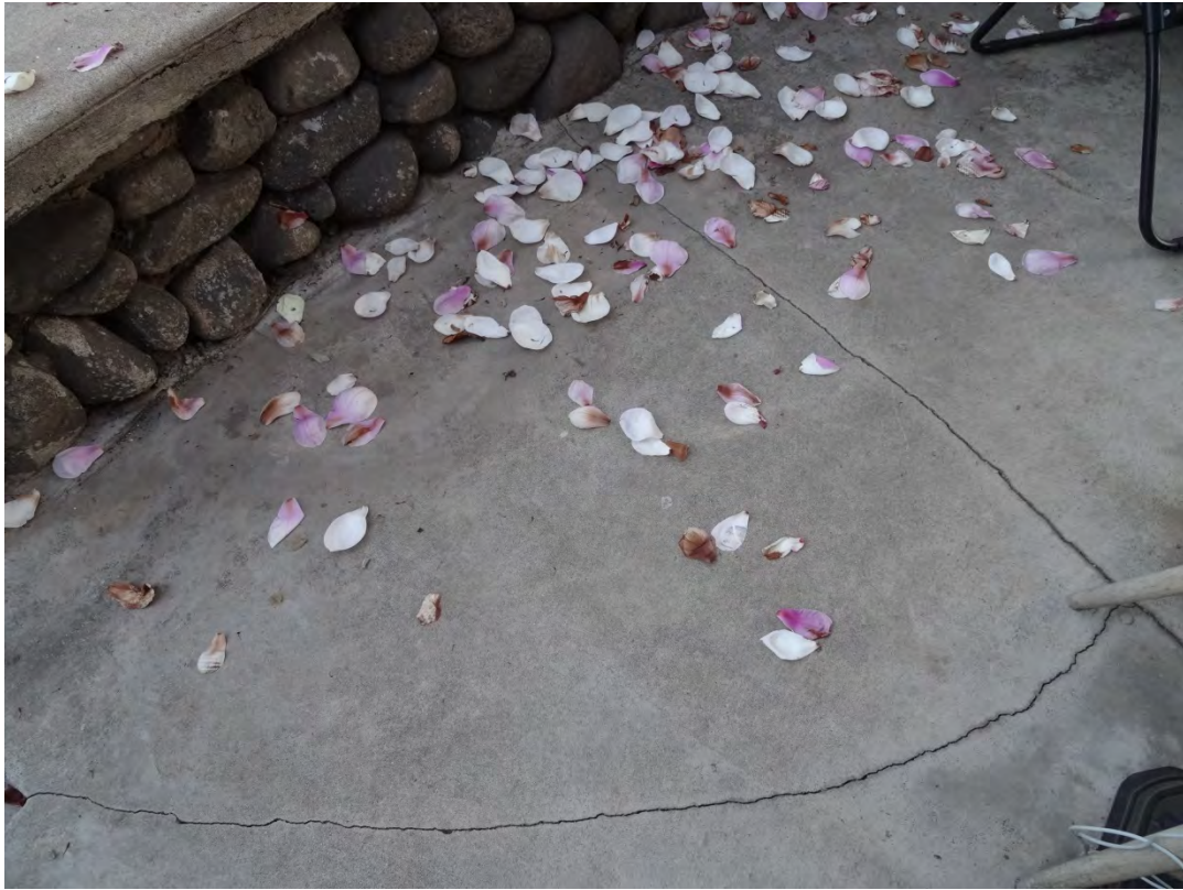
Cracks on the concrete porch floor
