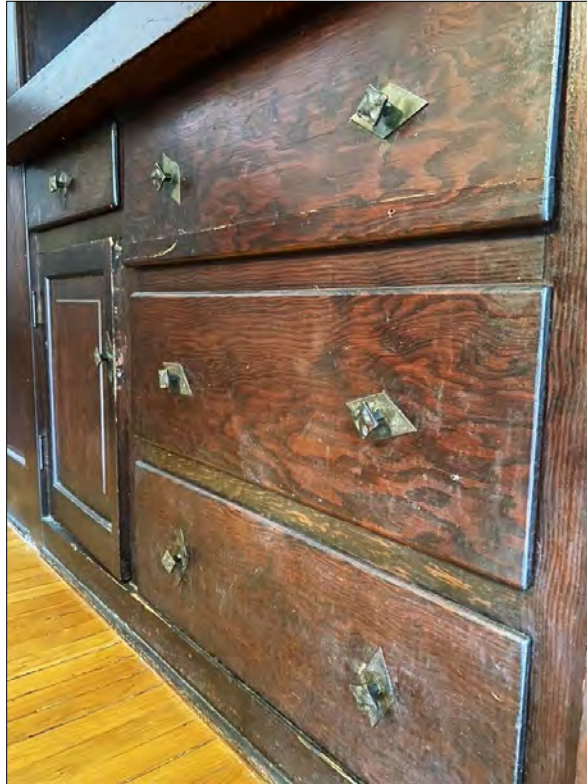
Built-in cabinetry in the dining room needs to be repaired and refinished.
