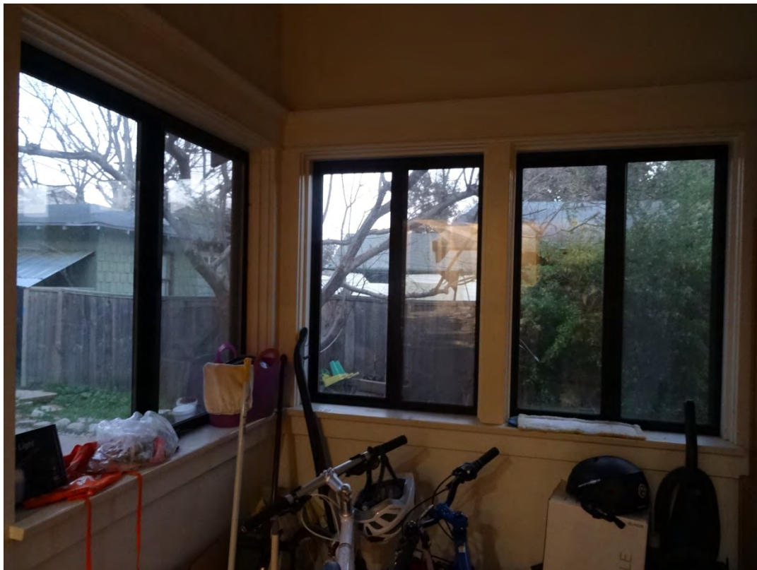
Non-original aluminum windows (to be replaced)
