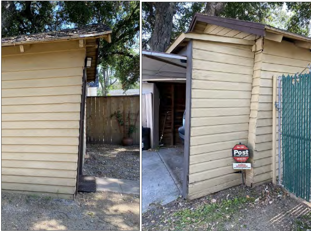
Original garage structure needs to be straightened and the frame needs to be strengthened with additional bracing.
