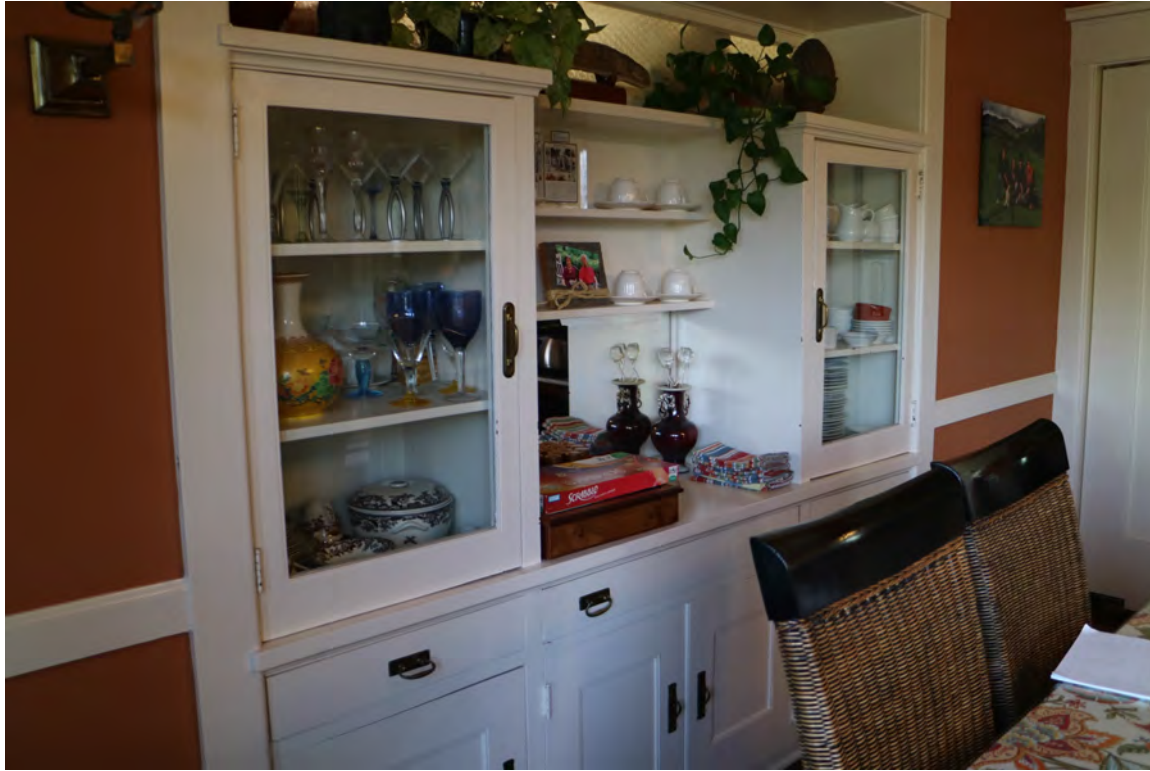
Figure 28 Interior cabinetry; overpainting has led to poorly fastening cabinet doors
