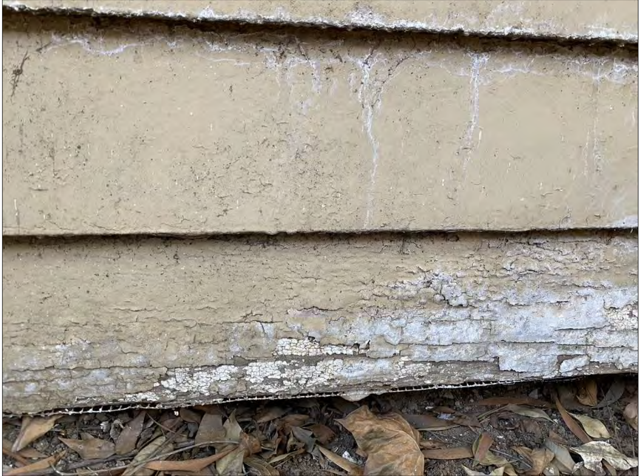
Some of the wood siding along the bottom edge of the house is showing water damage and will need to be repaired.
