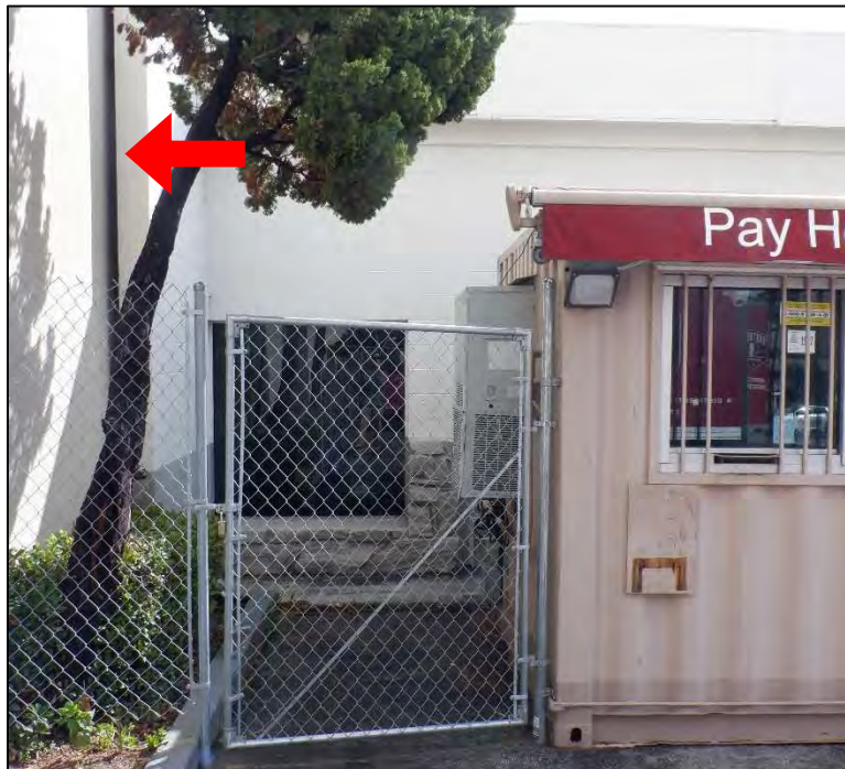
Photograph 10: Detail view showing the narrow separation between the garage building at 1400 Mission Street and the neighboring building at 812 Fremont Avenue (denoted by the red arrow). Camera facing east, March 23, 2023.
