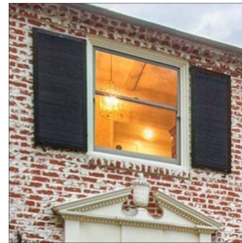
WIDNOWS & DOORS EXTERIR WOOD WINDOWS & DOORS (SIERRA PACIFICA WOOD WINDOWS) PAINTED WHITE TO MATCH EXISTING w/ BLACK WOOD SHUTTER WHERE OCCURS
