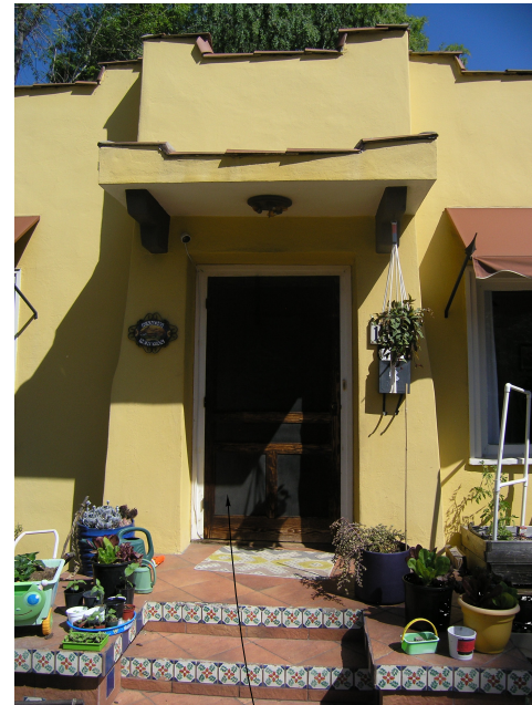
FRONT DOOR NEW WOOD PLANK DOOR STAINED DEEP BROWN BLACK CABOT SOLID STAIN
