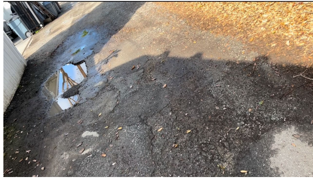
Large pothole on the way to home driveway gate entry
