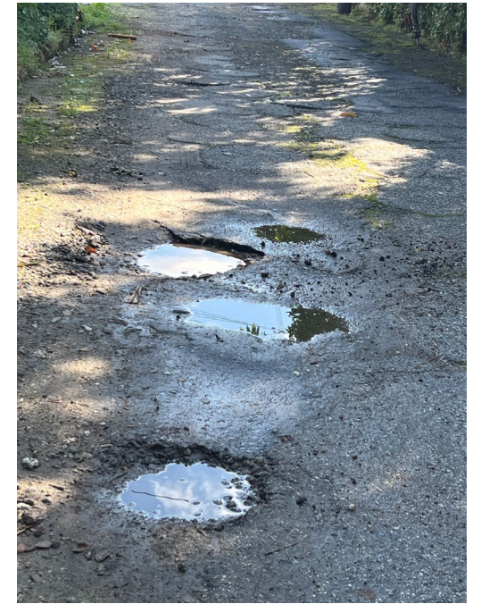
Multiple potholes all the way toward Milan
