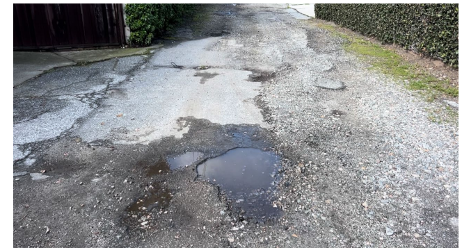
Pothole on North Alley at Montrose Lane
