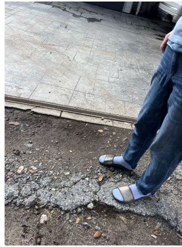
Erosion edge trip hazard at gate entry. Note mud tire tracks from North Alley and Gravel dragged onto driveway. Stamped Concrete driveway pattern flattened.
