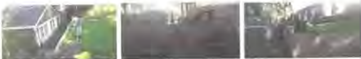
a) swale & retaining wall b) low and high retaining walls c) high retaining wall
