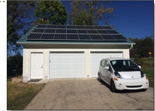
Solar installation to achieve net-zero carbon emissions
