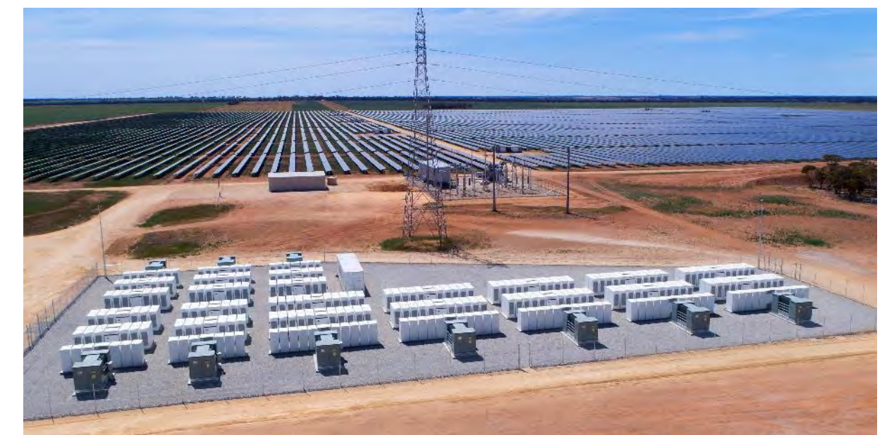
Commercial Solution: Solar and Storage
