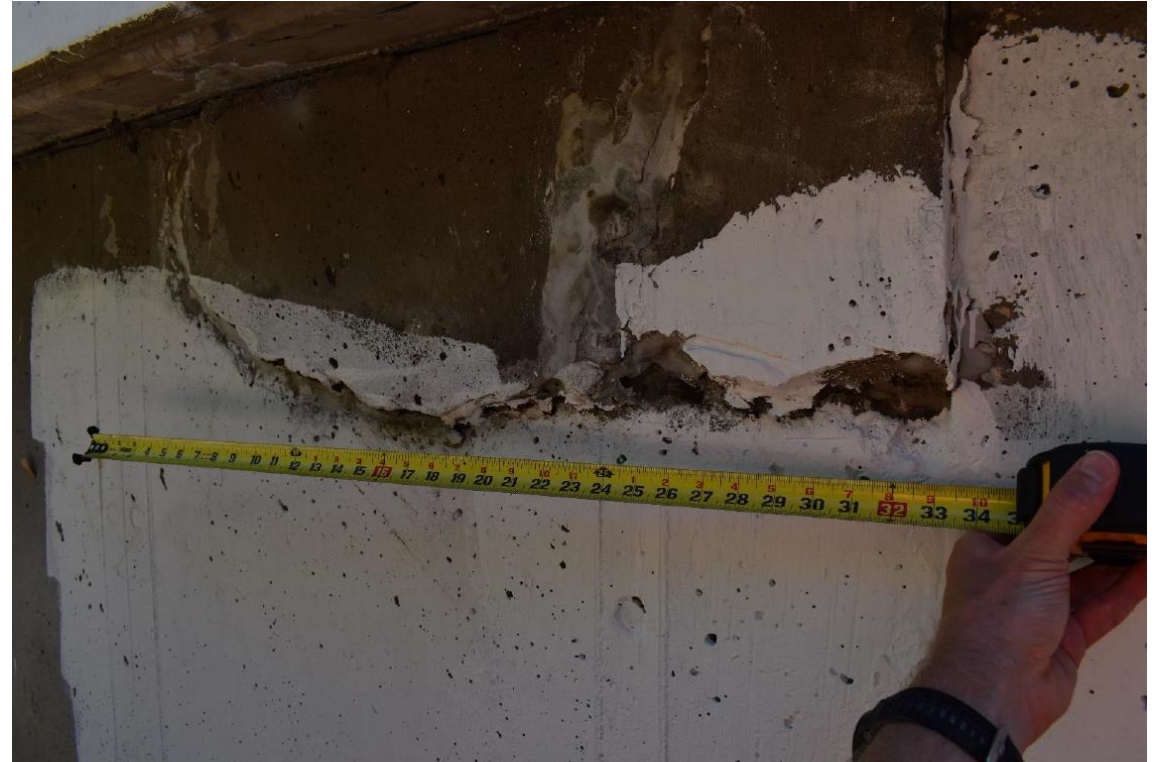
Photograph 7: 33-inch Wide Cracked Section Adjacent to Wall Joint at 210-degrees
