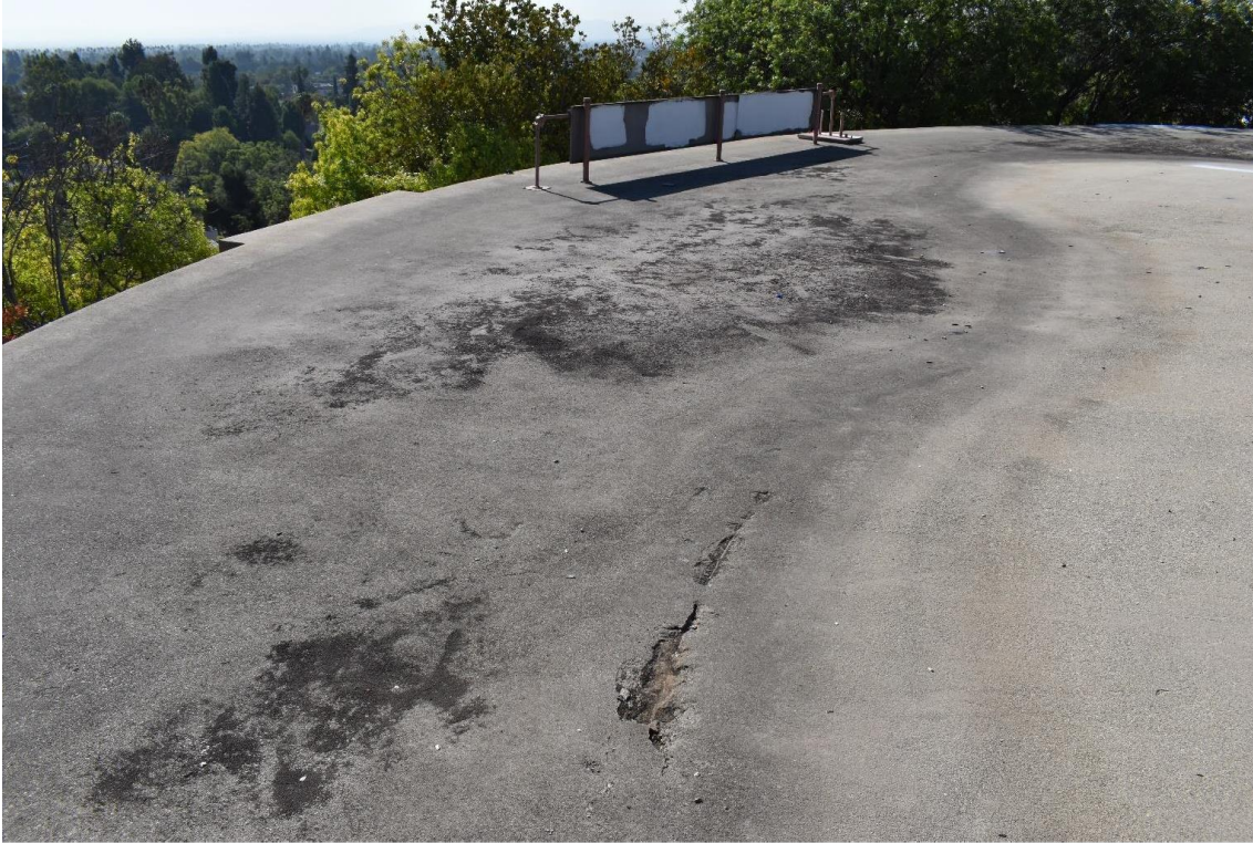
Photograph 3: Discoloration and Debris at Low Points in Roof Slab (PSE 8/17/2022)
