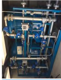
Stormwater Harvesting Unit
