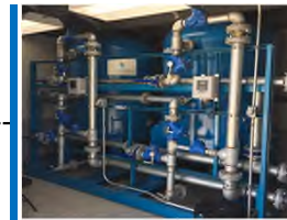
Stormwater Harvesting Unit
