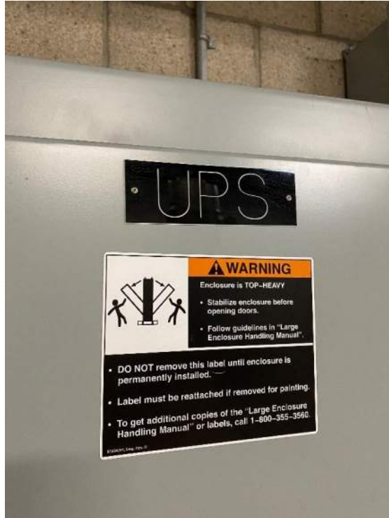
(Grand-23) UPS Panel
