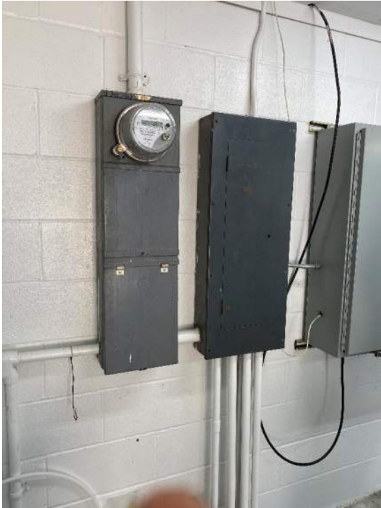
(Kol-17) Electrical Panel Inside Metering Building
