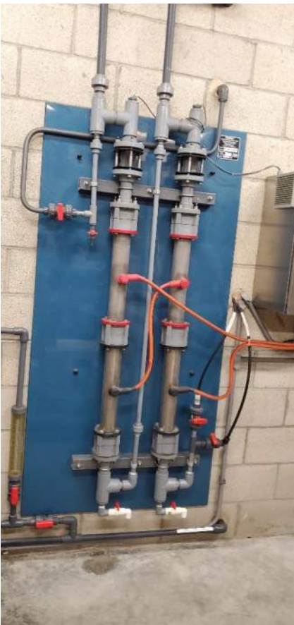
(Grand-10) Chemical Monitoring Equipment
