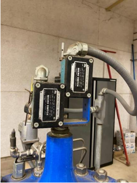
(Wil-19) Pump Monitoring Equipment
