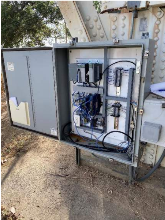
(Ray-15) Inside of Electrical Box
