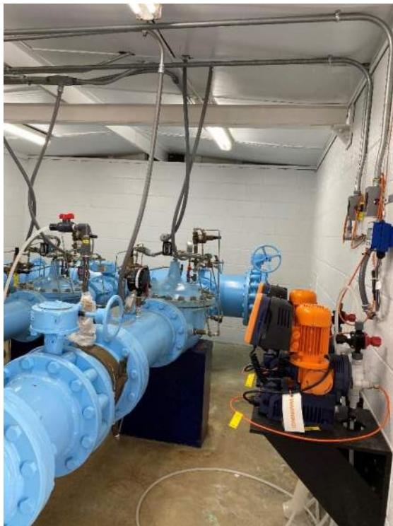
(Kol-20) Temporary Chemical Dosing Pumps
