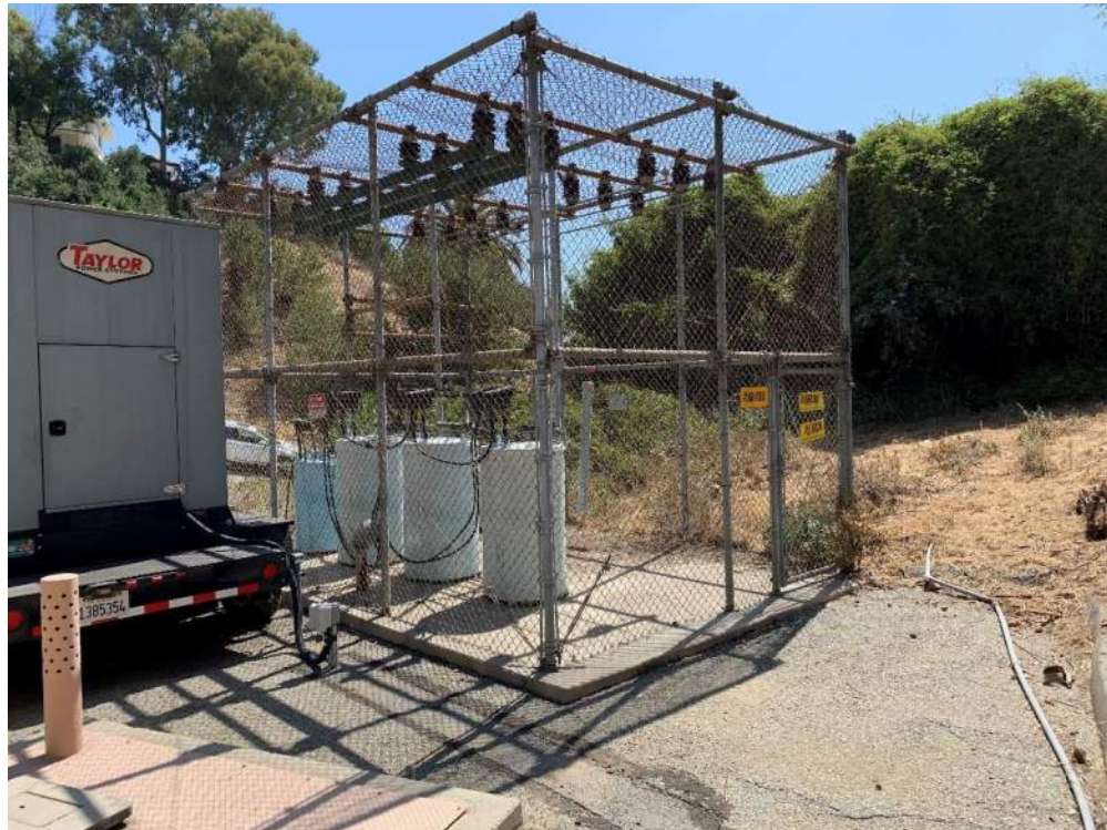
(West-14) Electrical Transformers and Mobile Backup Generator Outside Pump Room
