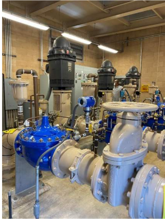
(Gar-17) Pumps and Motors
