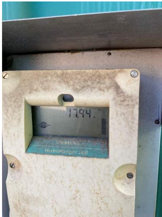
(Grand-32) Chemical Monitoring Equipment
