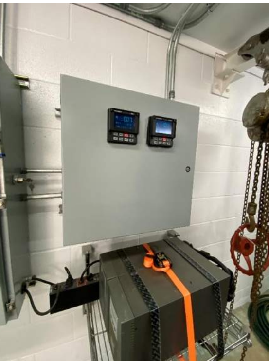
(Kol-14) Electrical Panel and Battery System Inside Metering Building
