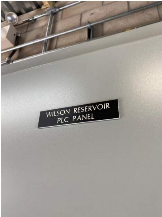
(Wil-14) Electrical Panel Inside Pump Room
