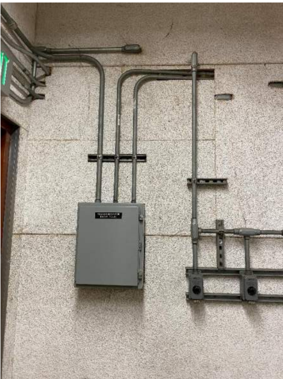
(Wil-16) Electrical Panel Inside Pump Room
