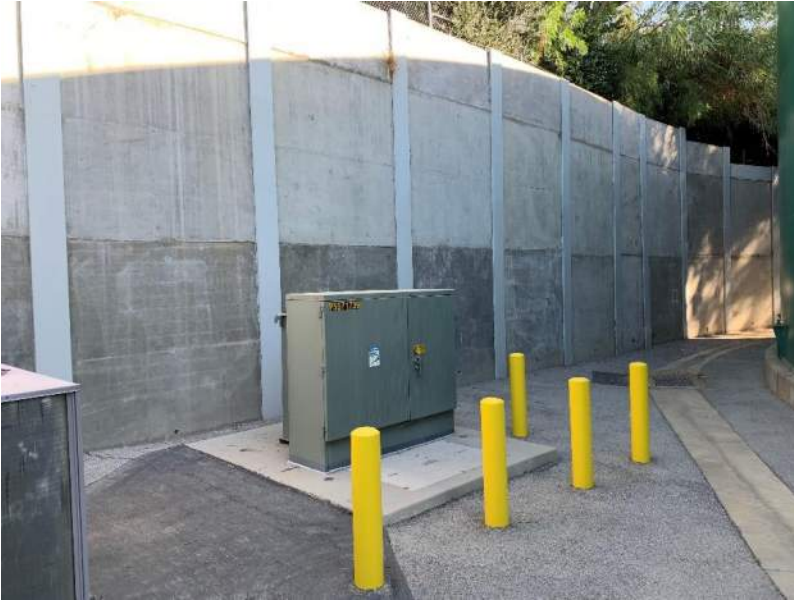
(Grand-9) Electrical Box
