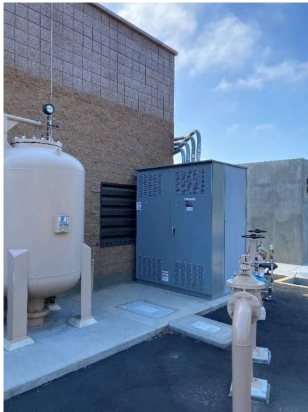
(Gar-10) Break Tank Outside Pump Room
