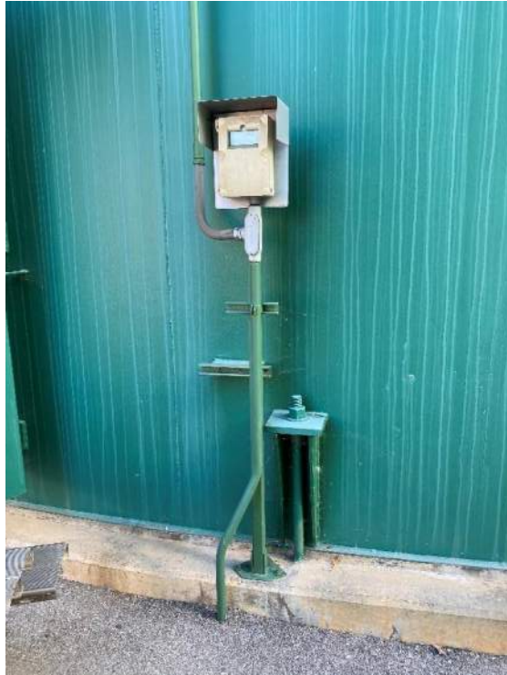
(Grand-31) Chemical Monitoring Equipment
