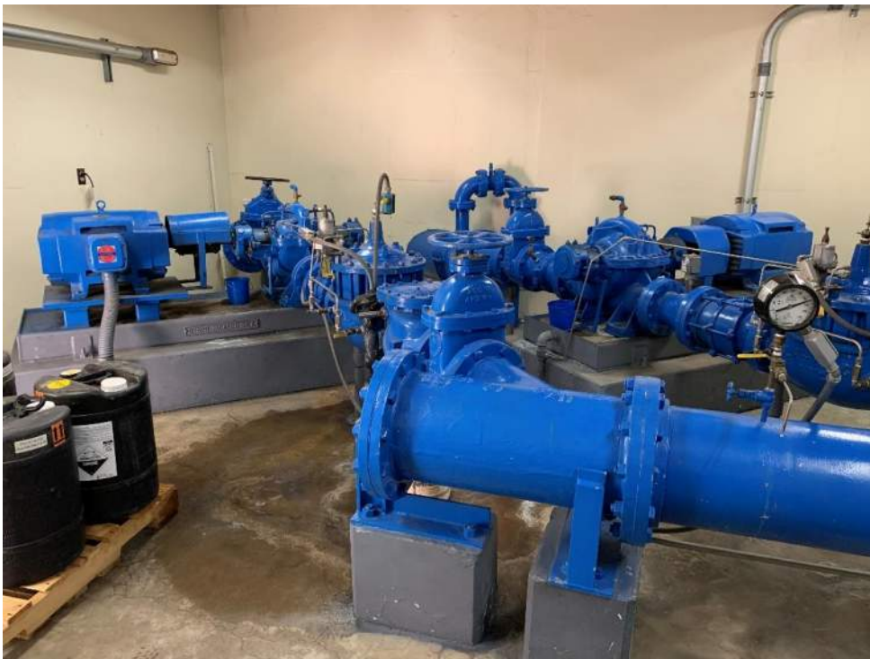
(West-12) Pumps, Motors, and Valve Assemblies Inside Pump Room
