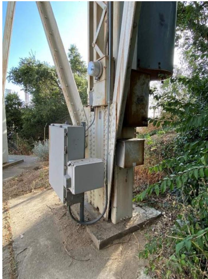
(Ray-14) Outside of Electrical Box
