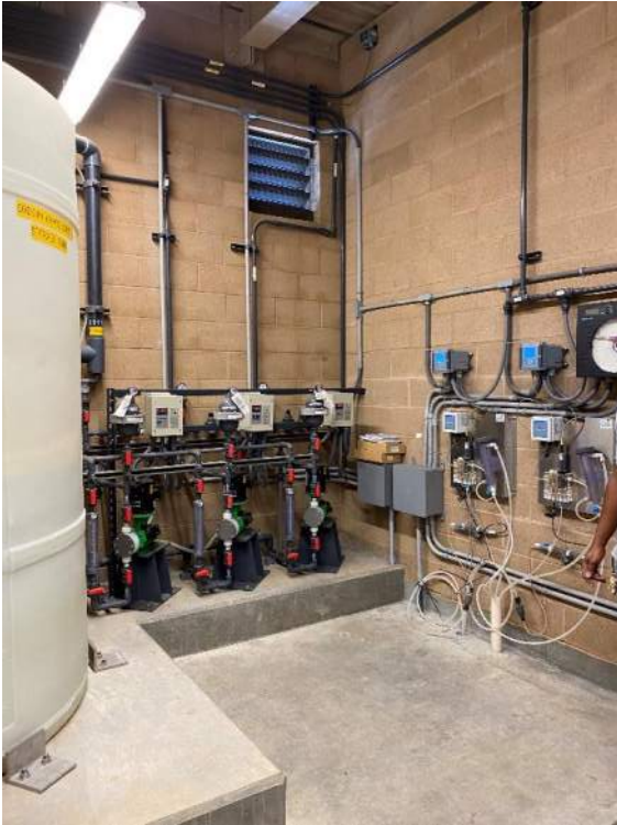
(Gar-19) MicroChlor System in Chemical Room
