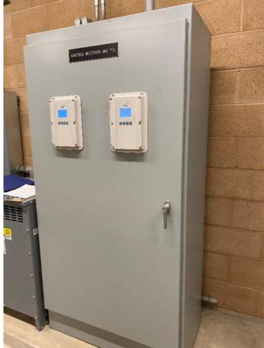
(Gar-14) Pump Controls Inside Pump Room
