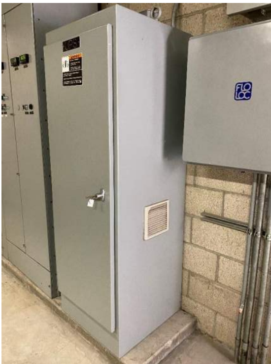
(Grand-26) Electrical Panel Inside Pump Room
