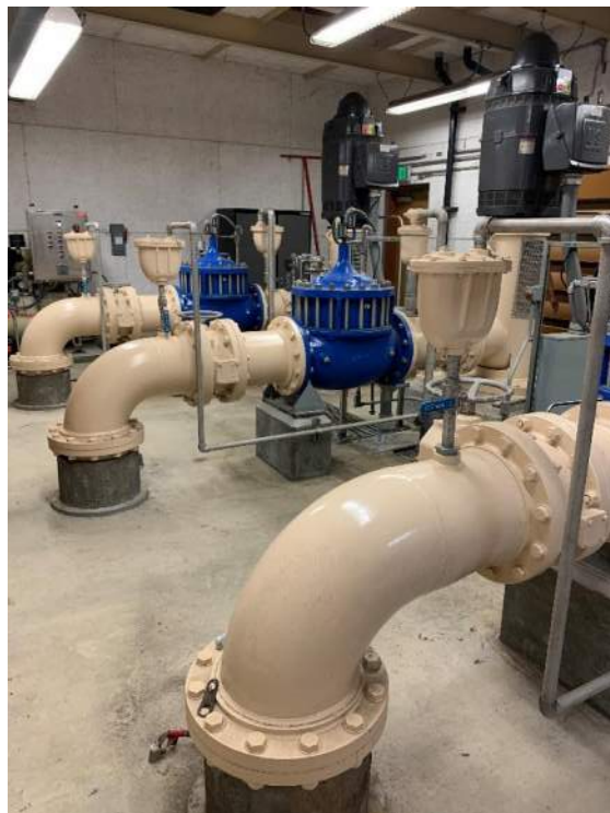
(Wil-10) Inside of Pump Room
