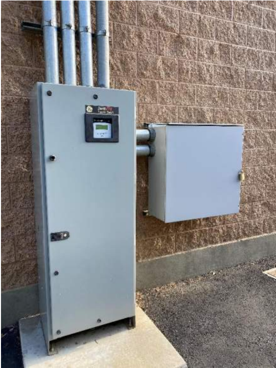
(Gar-11) Control Panel Outside Pump Room
