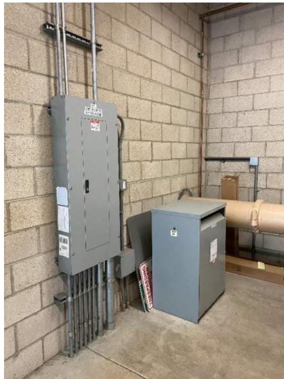
(Grand-24) Electrical Panel Inside Pump Room
