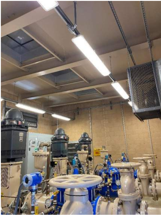
(Gar-15) Pumps and Motors
