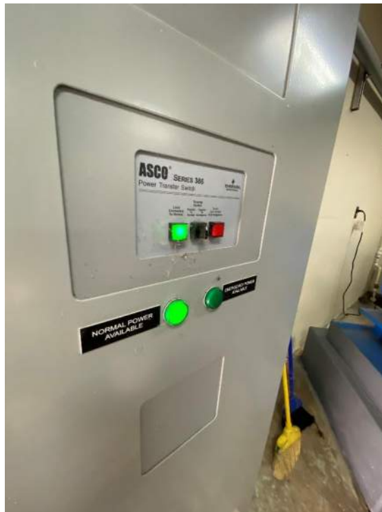
(West-22) Electrical Equipment Inside Pump Room
