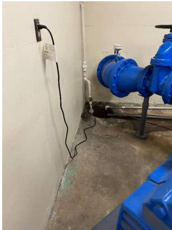
(West-26) Intake Pipeline
