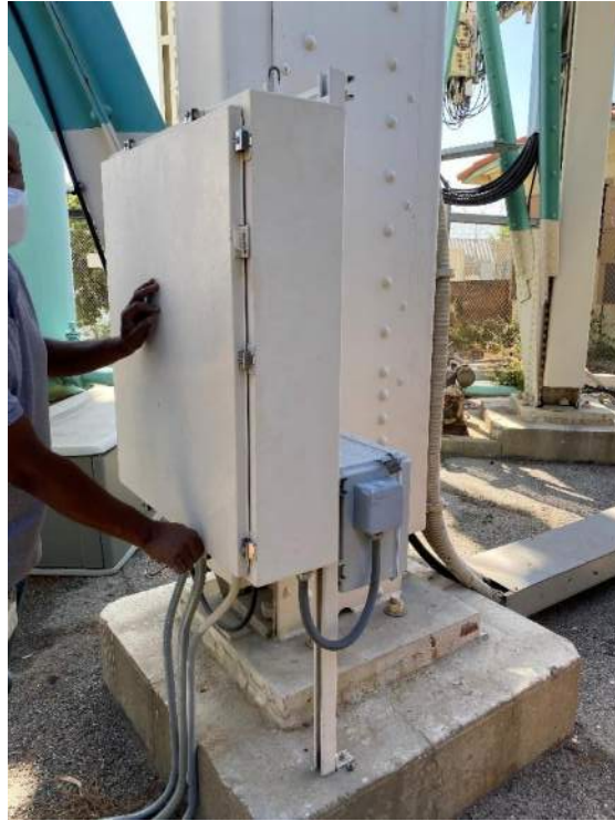
(Bil-15) Electrical Equipment at Tank Site
