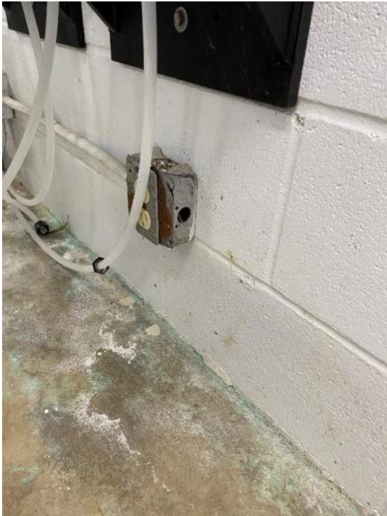
(Kol-21) Temporary Chemical Dosing Tubing
