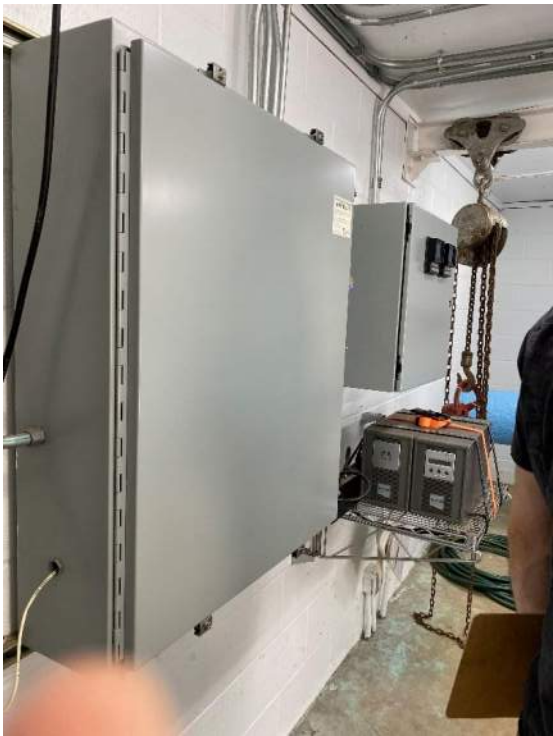
(Kol-18) Electrical Panel Inside Metering Building
