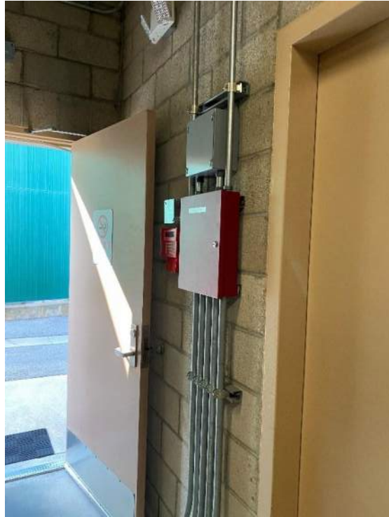
(Grand-27) Electrical Equipment – Inside Pump Room
