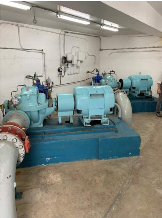
(Ind-2) Pumps and Motors
