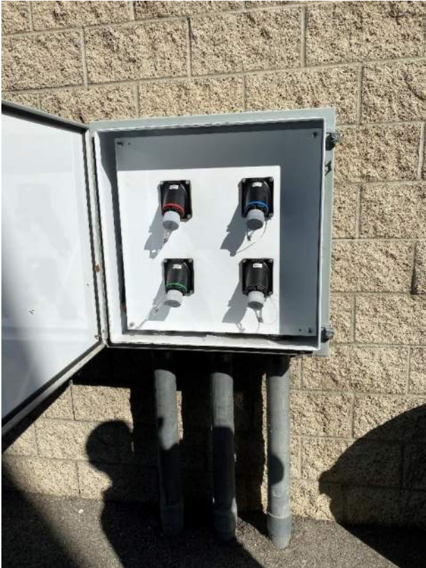
(Grand-21) Generac Hookup Panel
