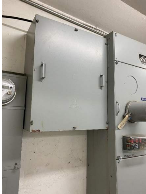
(Ind-7) Electrical Panel
