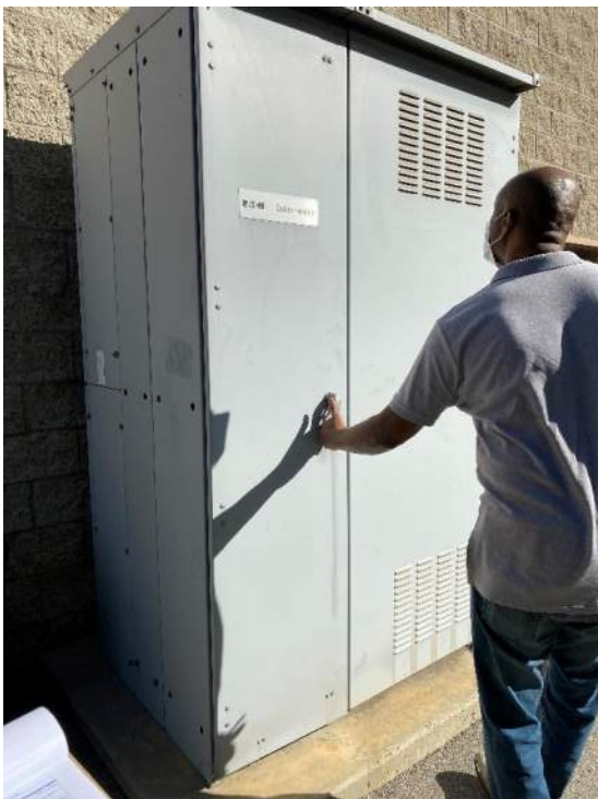
(Grand-18) Electrical Box Outside of Pump Room
