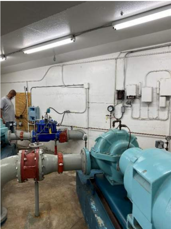
(Ind-10) Pump and Motor
