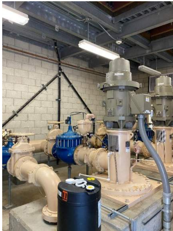
(Grand-28) Pumps and Motors
