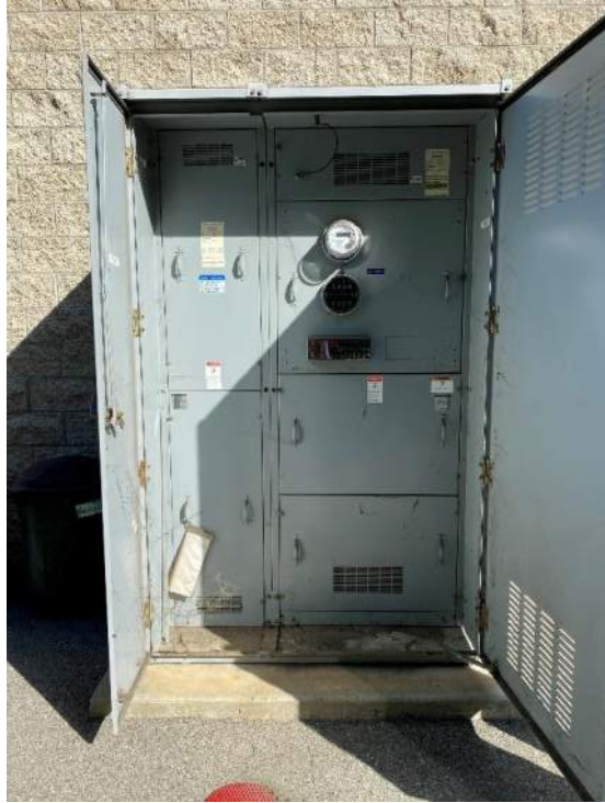
(Grand-19) Inside of Electrical Panel
