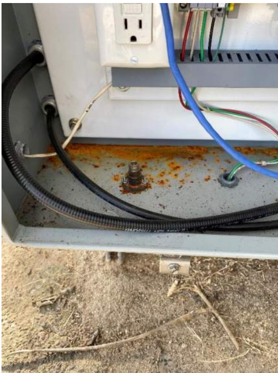
(Ray-16) Inside of Electrical Box
