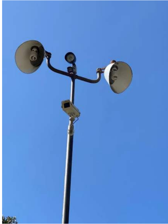
(West-17) Site Lighting and Surveillance Camera Outside Pump Room
