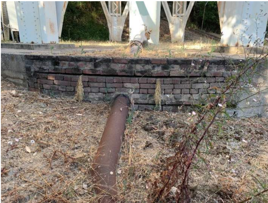
(Ray-12) INLET/OUTLET PIPE
