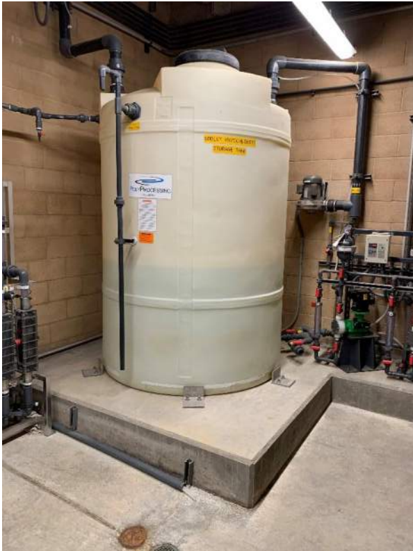
(Gar-7) Hypochlorite Tank in Chemical Room
