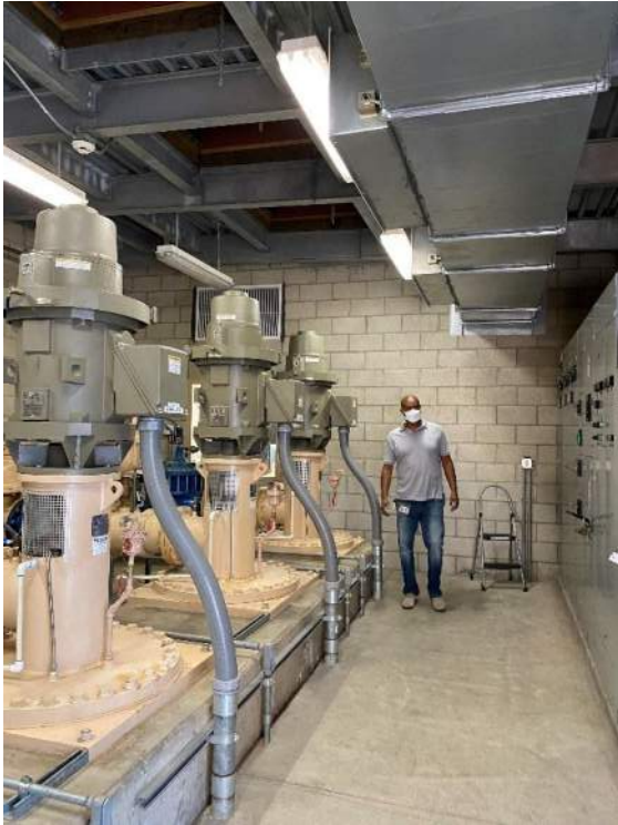
(Grand-25) Pump Motors
