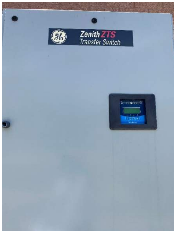
(Wil-18) Electrical Panel Outside of Pump Room
