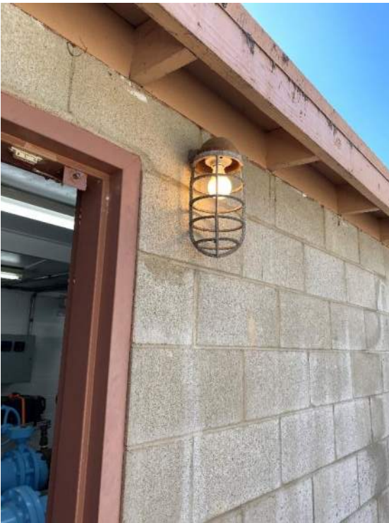
(Kol-10) Light Outside of Metering Building
