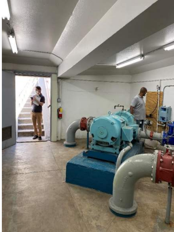
(Ind-11) Inside Pump Room
