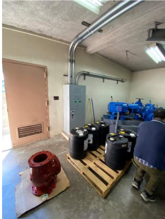
(West-25) Spare Check Valve Inside Pump Room
