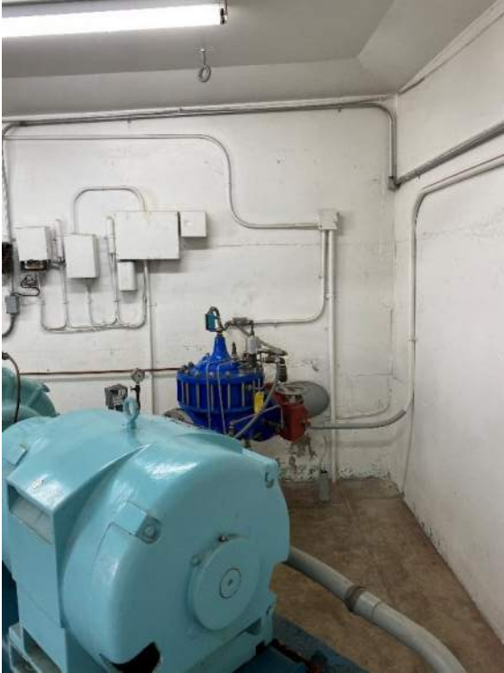
(Ind-9) Pump Motor
