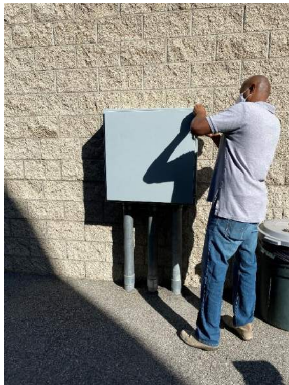
(Grand-20) Outside of Generac Hookup Panel
