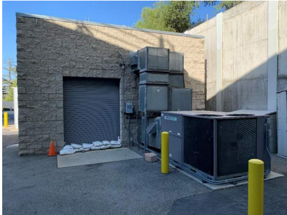
(Grand-8) Side of Pump Room
