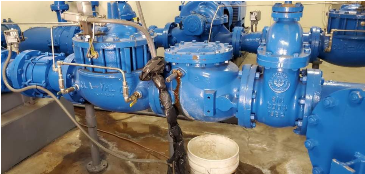
(West-15) Pumps, Motors, and Valve Assemblies Inside Pump Room
