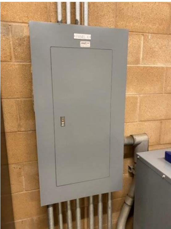
(Gar-12) Electrical Panel Outside Pump Room
