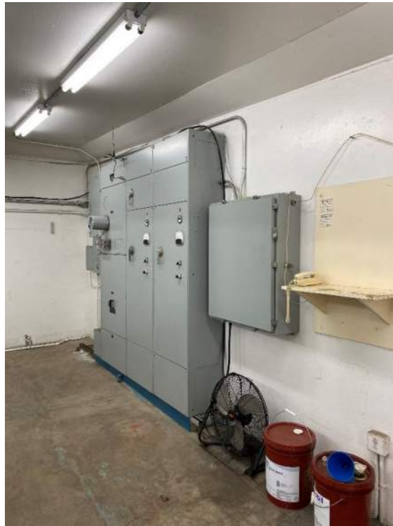
(Ind-8) Electrical Panel
