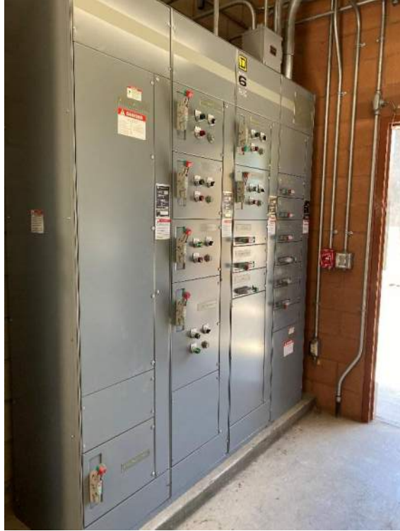
(Wil-13) Electrical Panel Inside Pump Room
