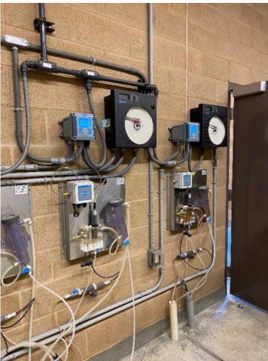
(Gar-20) Chemical Monitoring Equipment Inside Chemical Room
