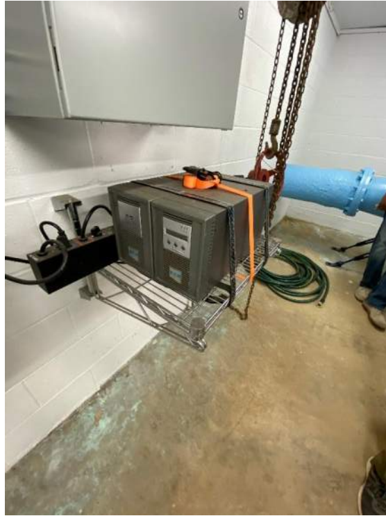
(Kol-15) Battery System Inside Metering Building
