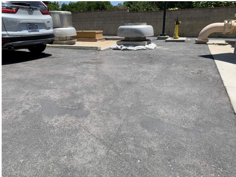
(Wil-6) Vent for Underground Well 2
