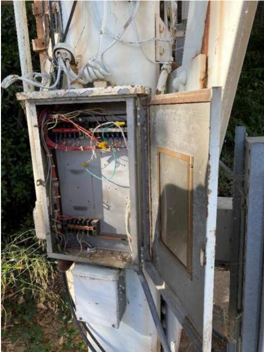
(Ray-19) Inside of Electrical Box
