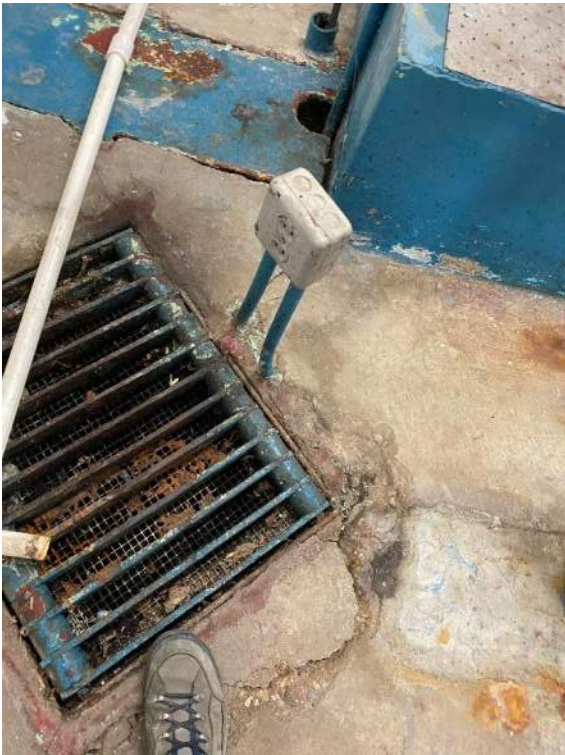
(Ind-14) Pump room Drain
