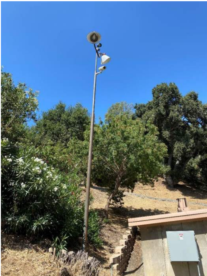
(West-16) Site Lighting and Surveillance Camera Outside Pump Room
