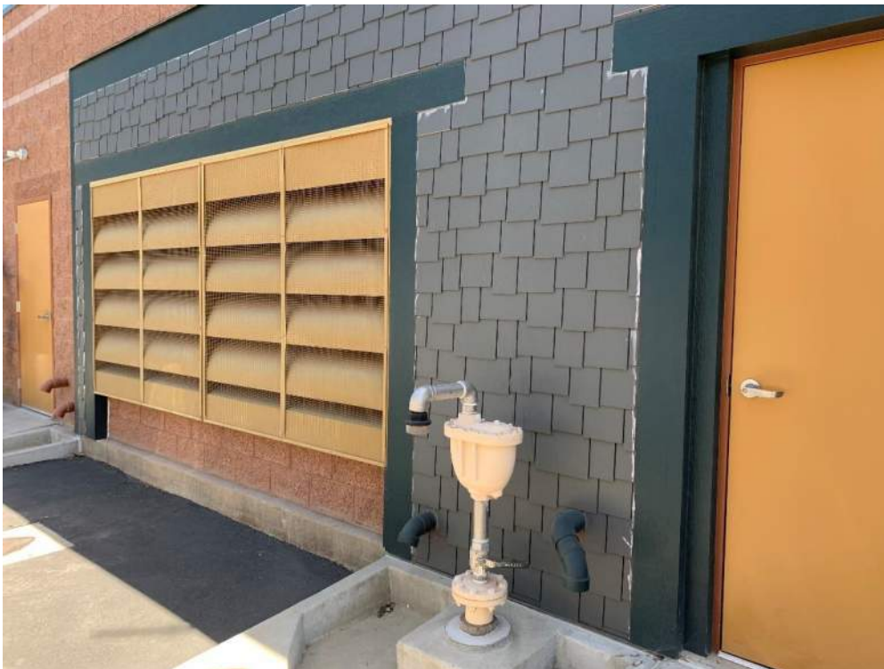
(Wil-4) Vacuum Valve Outside of Pump Room
