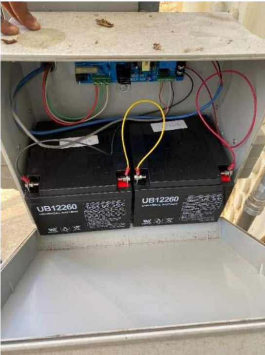
(Ray-20) 12-V Battery System
