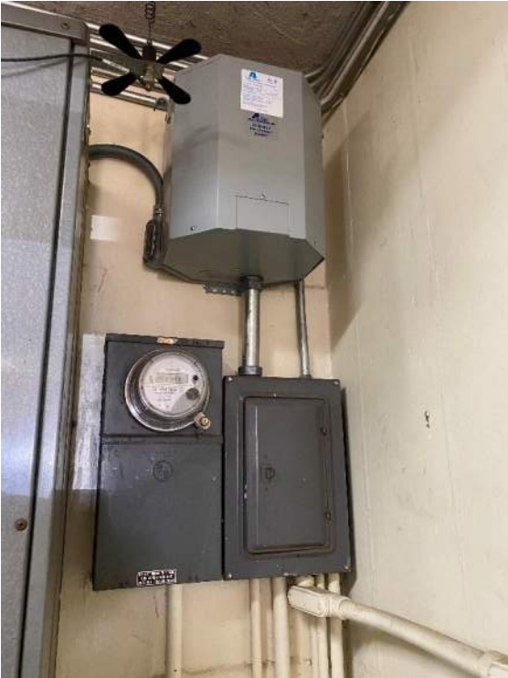
(West-23) Electrical Equipment Inside Pump Room
