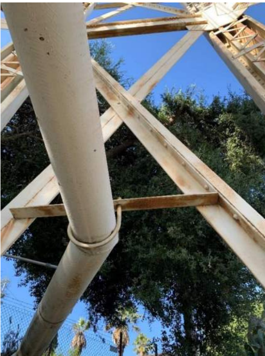
(Ray-8) Inlet/Outlet Pipe
