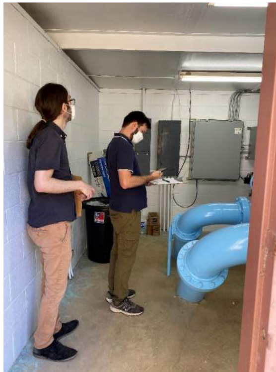
(Kol-16) Inlet Headers Inside Metering Building
