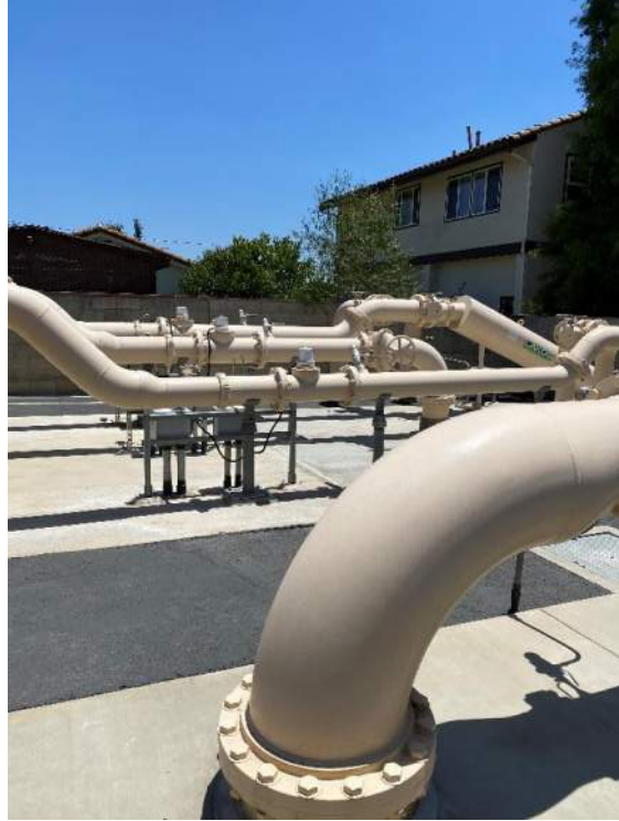
(Wil-21) Yard Piping
