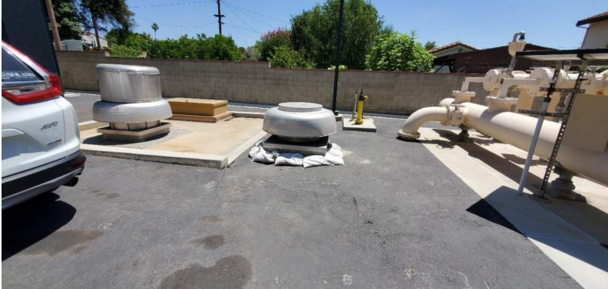
(Wil-11) Vent Above Well 2
