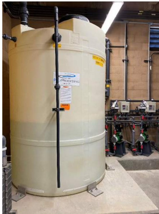
(Gar-18) Hypochlorite Tank Inside Chemical Room
