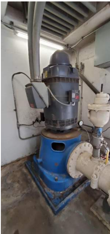
(Wil-8) Well 2 Pump and Motor
