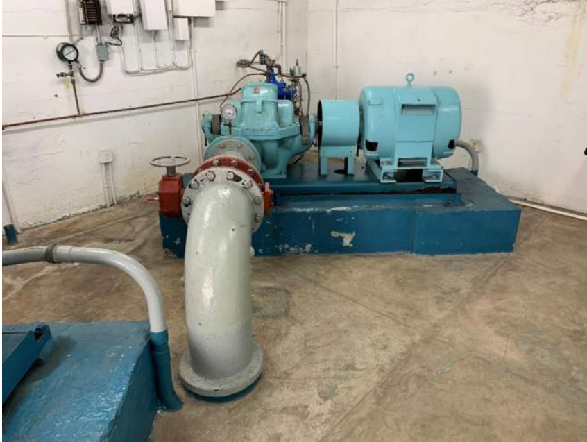
(Ind-5) Pumps and Motors
