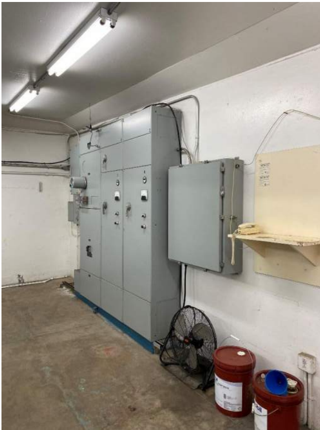
(Ind-6) Electrical Panel
