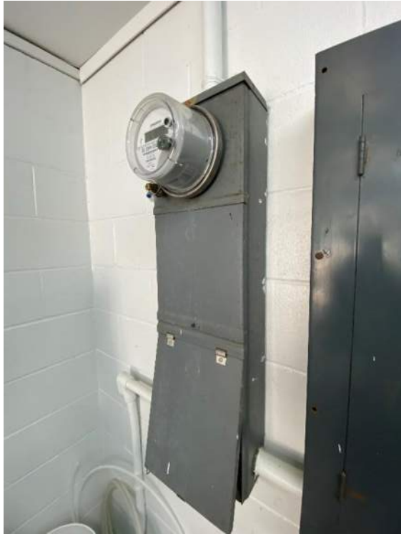
(Kol-11) Electrical Panel Inside Metering Building
