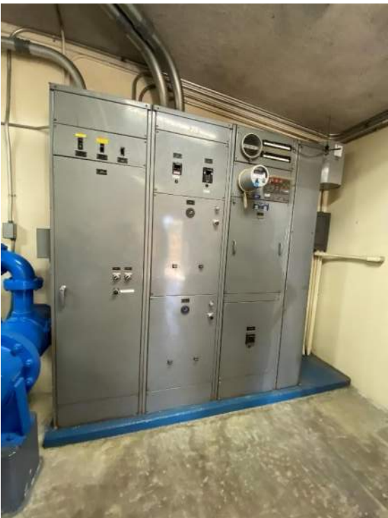
(West-20) Electrical Panel Inside Pump Room
