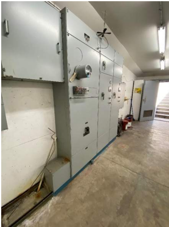
(Ind-12) Electrical Panel
