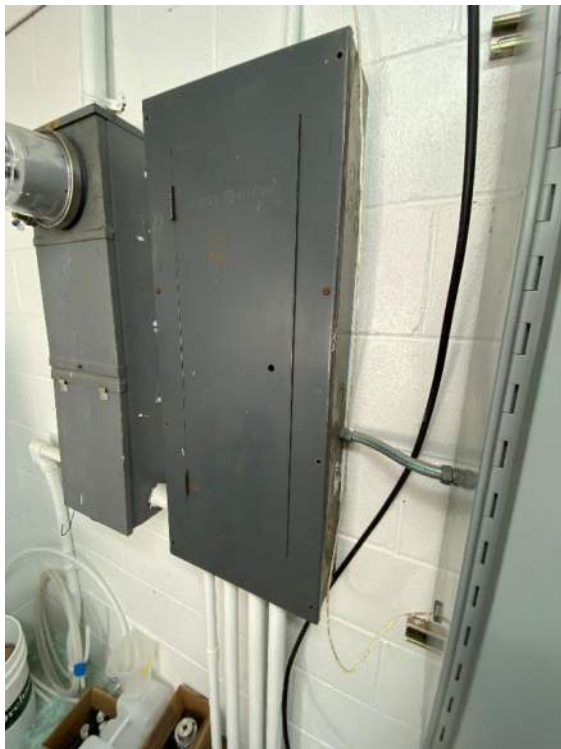
(Kol-12) Electrical Panel Inside Metering Building
