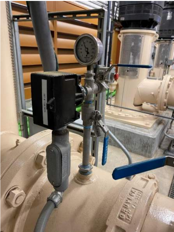
(Wil-20) Pump Monitoring Equipment
