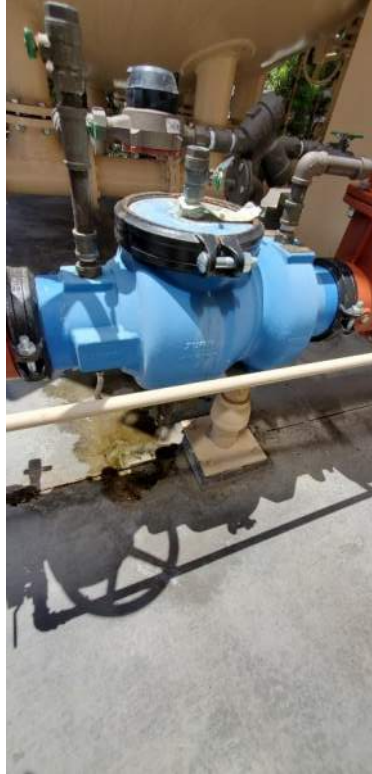
(Wil-9) Valve in GAC System
