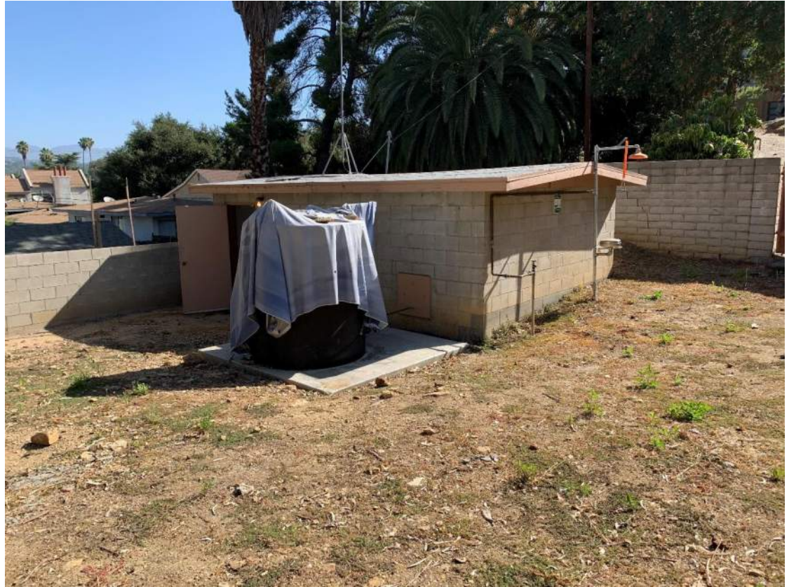
(Kol-7) Temporary Chemical Dosing Tank – Outside of Metering Building
