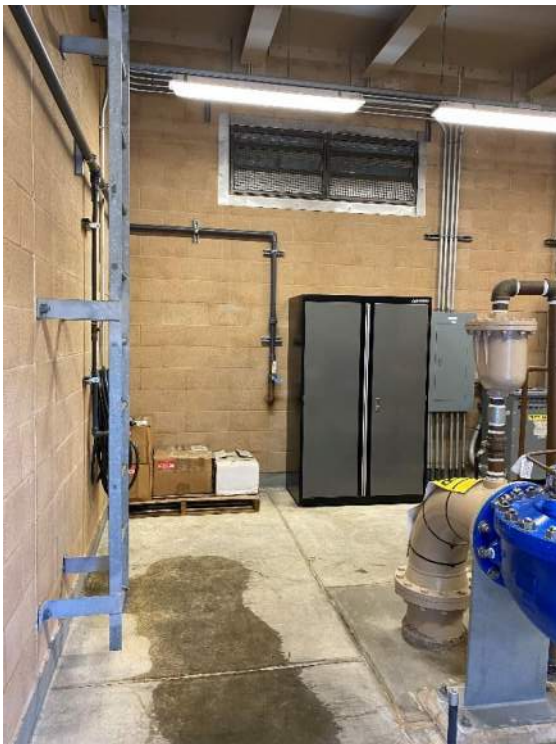
(Gar-16) Inside of Pump Room
