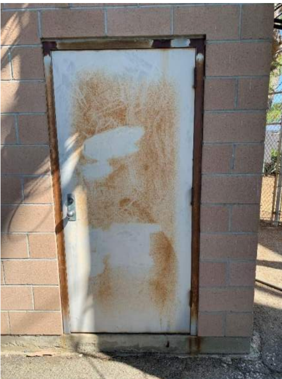
(Bil-6) Electrical Building at Tank Site
