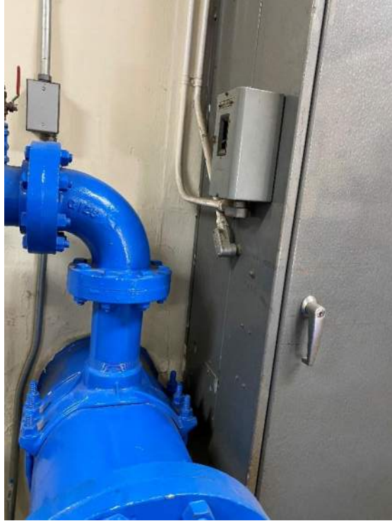
(West-21) Discharge Pipeline
