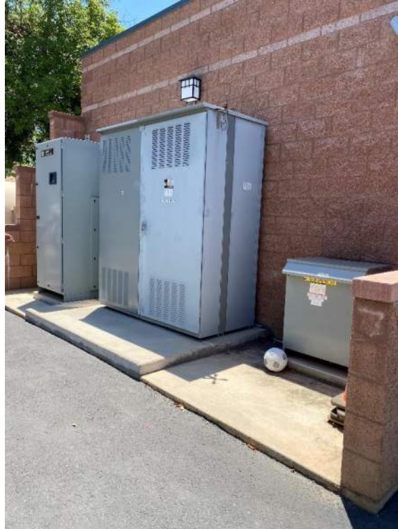
(Wil-17) Electrical Panel Outside of Pump Room
