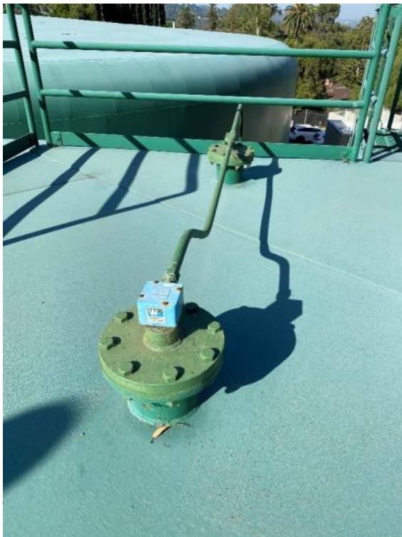
(Grand-30) Level Sensor on Reservoir 1
