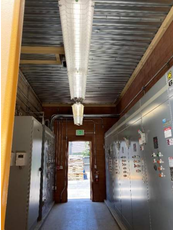
(Wil-15) Electrical Panel Inside Pump Room
