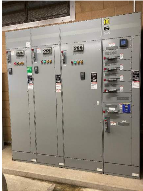
(Gar-13) Pump Controls Inside Pump Room
