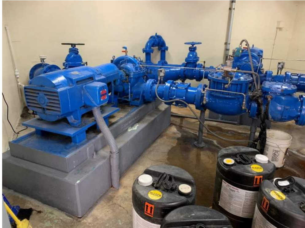
(West-13) Pumps, Motors, Valve Assemblies, and Temporary Chemicals Inside Pump Room
