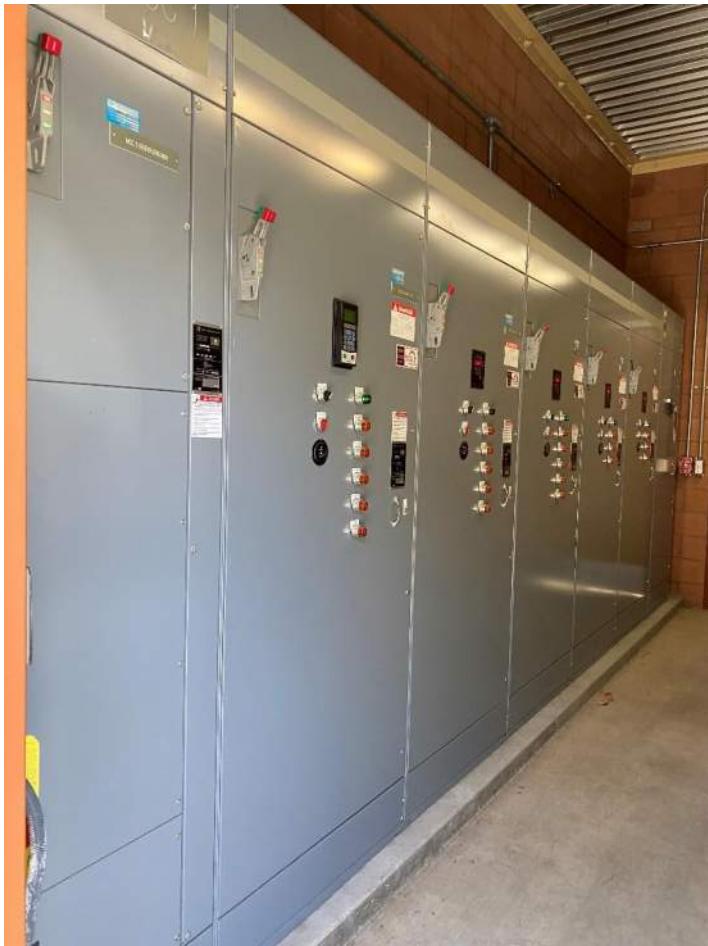
(Wil-12) Electrical Panel Inside Pump Room
