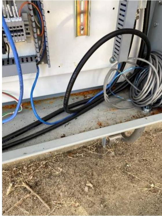
(Ray-17) Inside of Electrical Box
