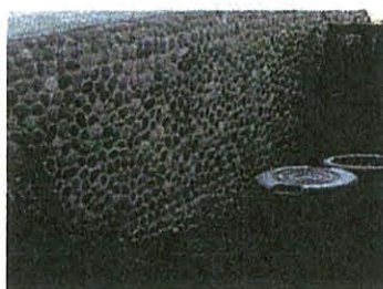
Re Use of later Stucco
