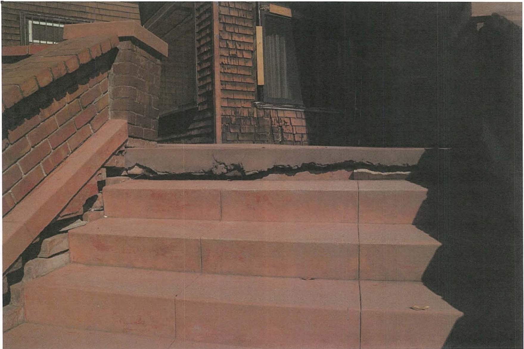
Figure 34 West stairs, detail of gap between stairs, west patio, and brick railing.
