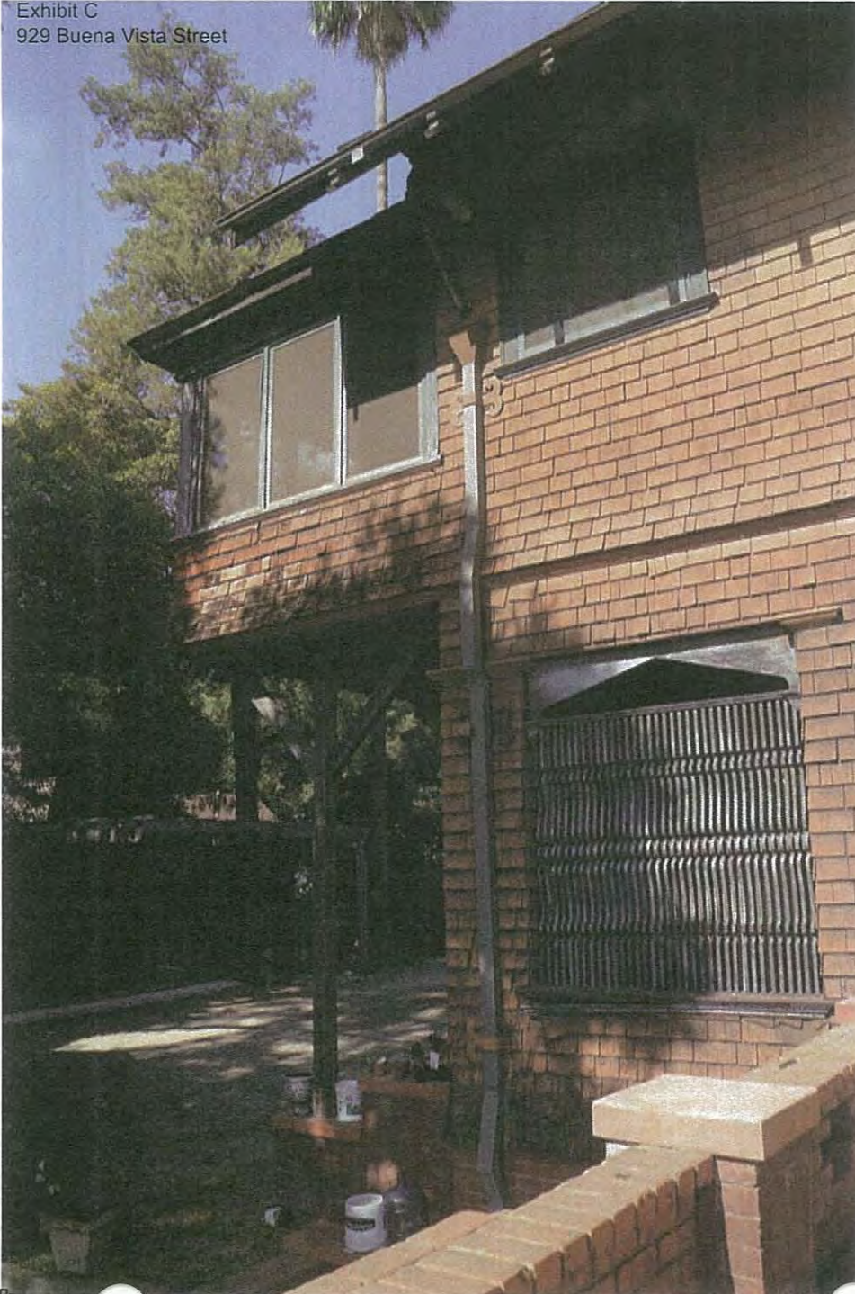
Figure 37 West elevation, detail of secondary entrance and second-story sleeping porch. View from west patio.
