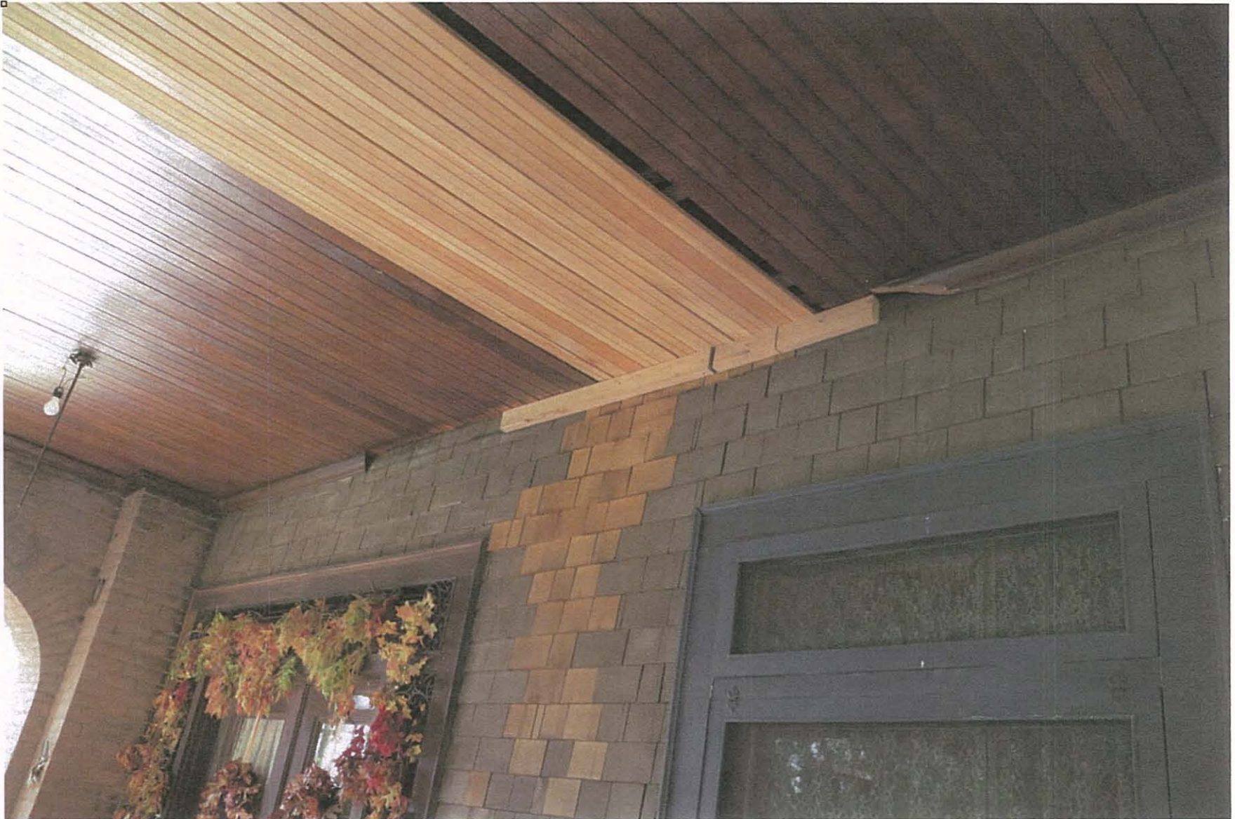
Figure 12 Torrance-Childs Residence, primary entrance. Replaced wood shingles and ceiling planks. Northeast perspective.
