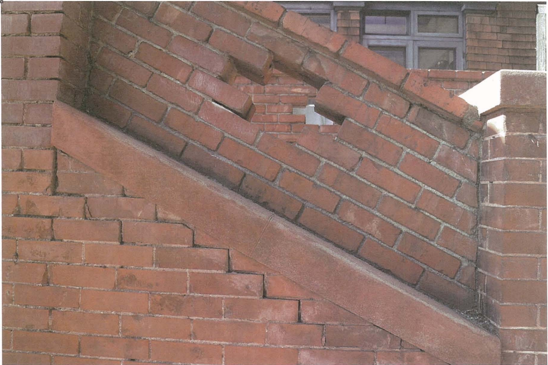
Figure 24 South stairs, detail of cracks and material failure. East perspective.
