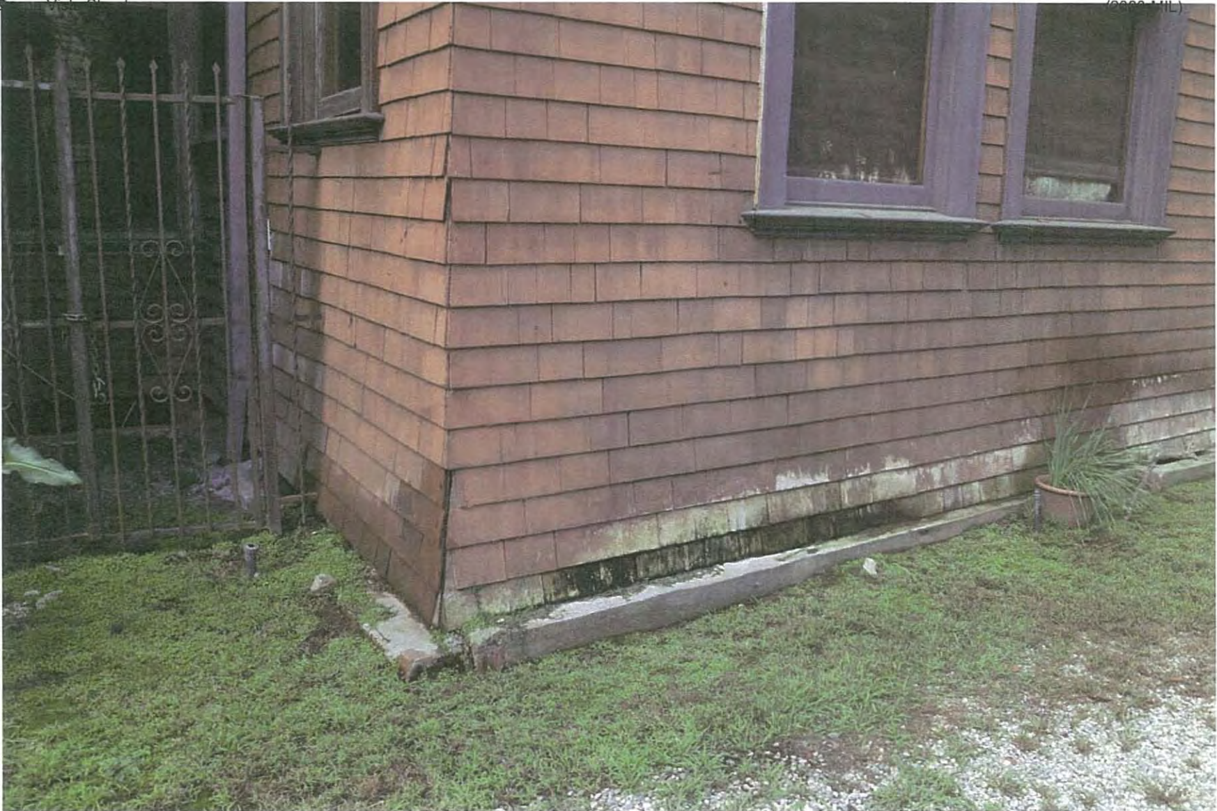
Figure 7 Torrance-Childs Residence. Water damage/mold on exterior shingles and foundation. Northeast perspective.
