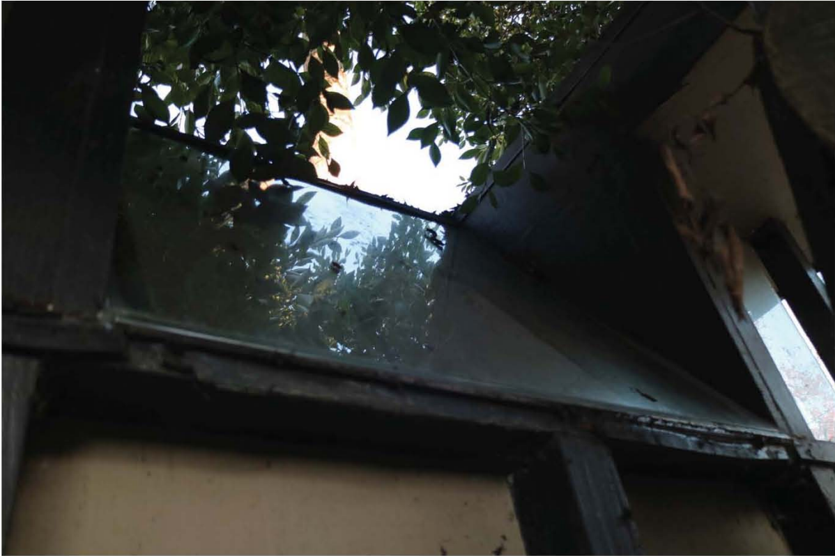
Figure 10. Smith Residence Studio, roof features and segments in need of water proofing, repairs and rehabilitation
