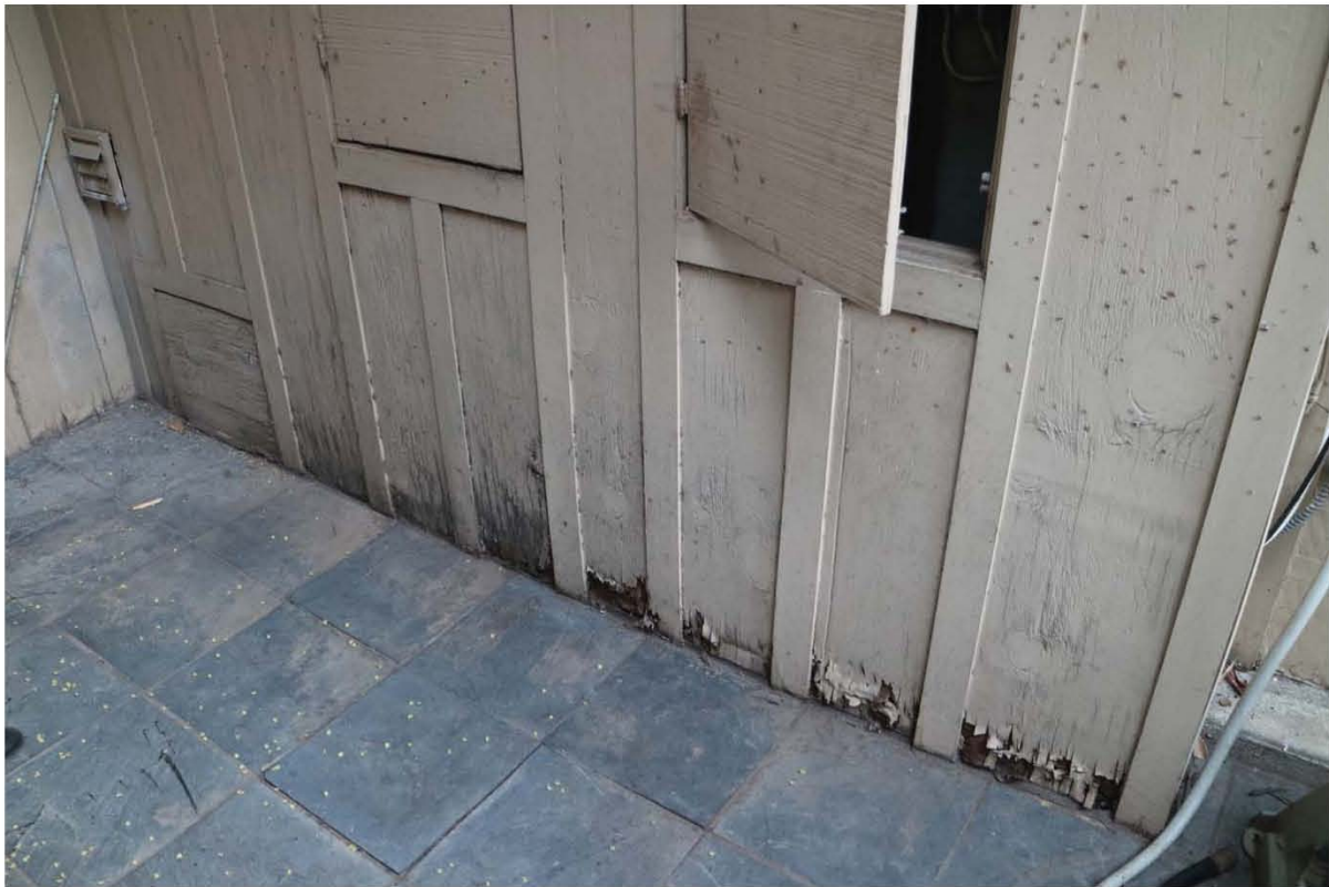
Figure 11. Smith Residence, wood elements and features in need of repairs and rehabilitation
