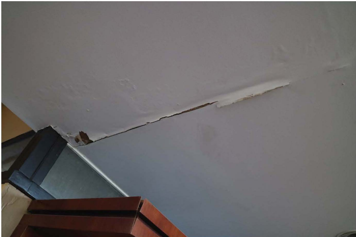
Figure 6. Smith Residence, areas of interior ceiling with water penetration, Living Room (top and bottom)
