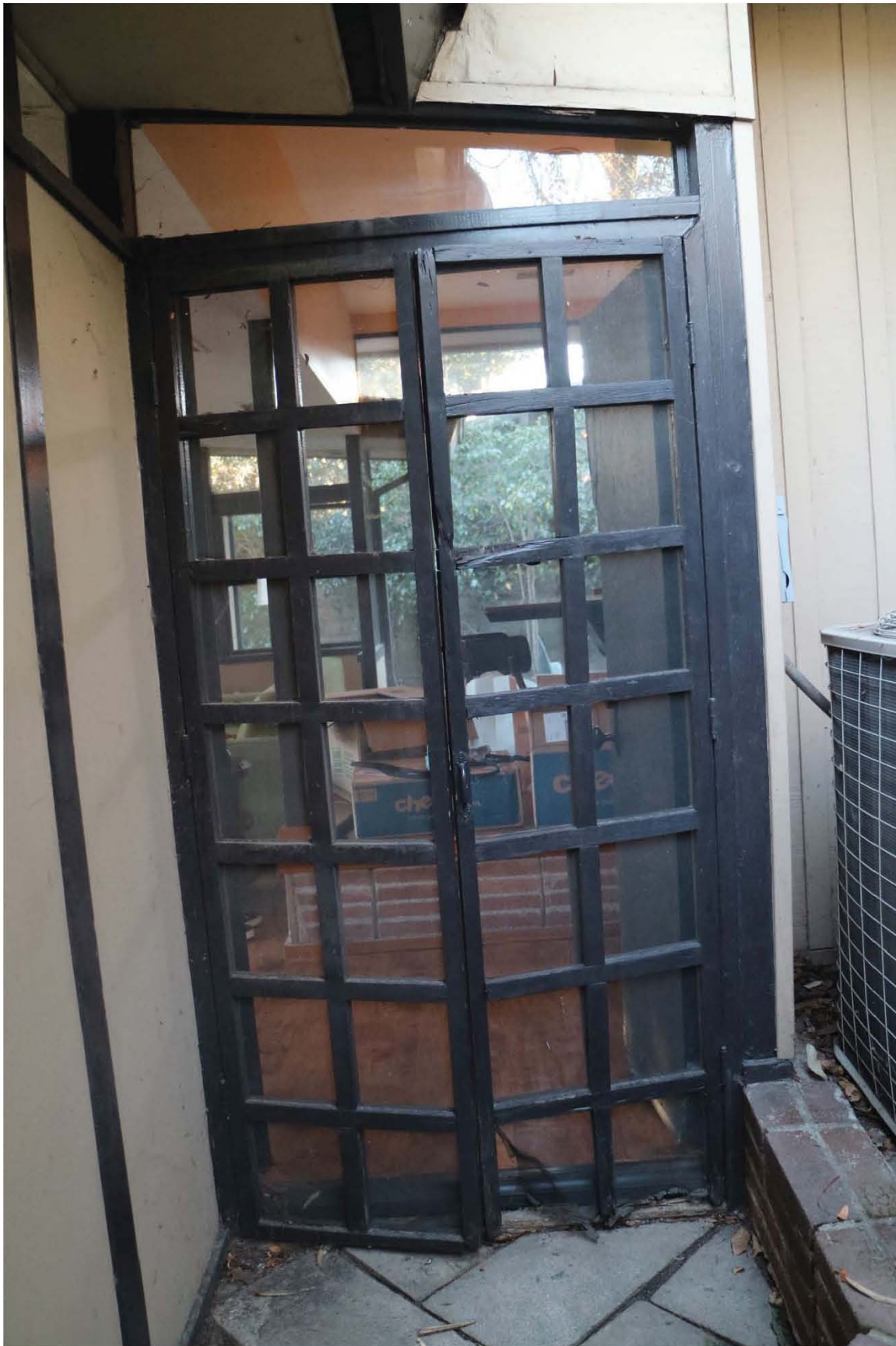
Figure 13. Smith Residence, wood elements and features in need of repairs and rehabilitation; north elevation entrance door and wood screen
