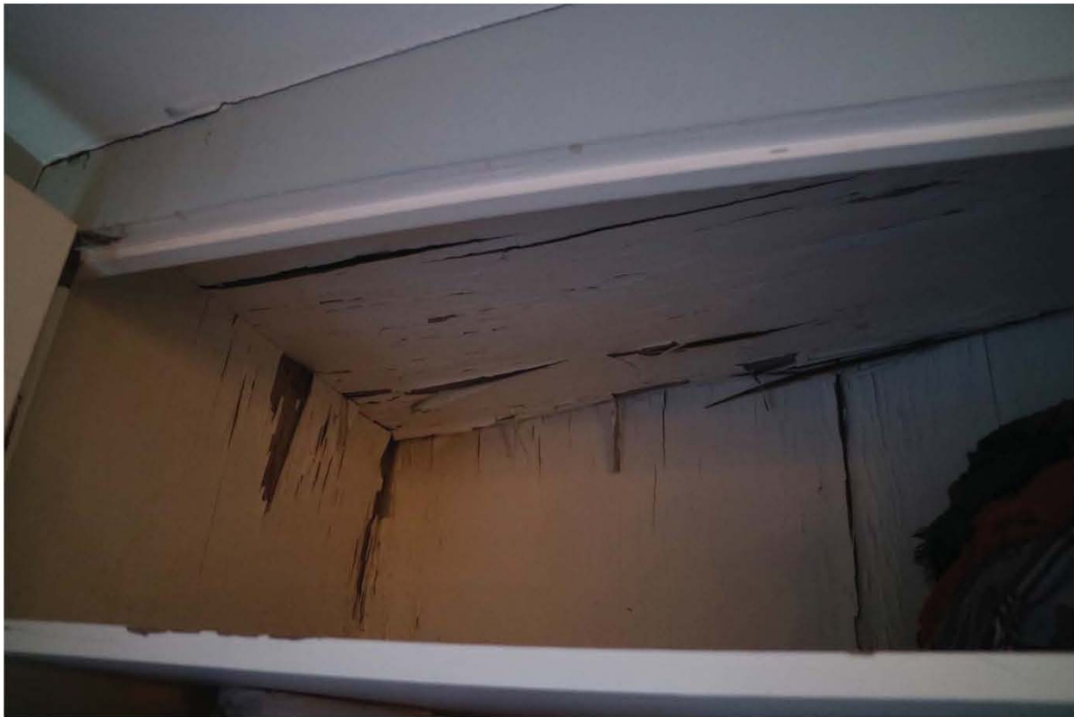
Figure 7. Smith Residence, areas of interior with water penetration, bedroom closet (top) and secondary entrance, south elevation (bottom)
