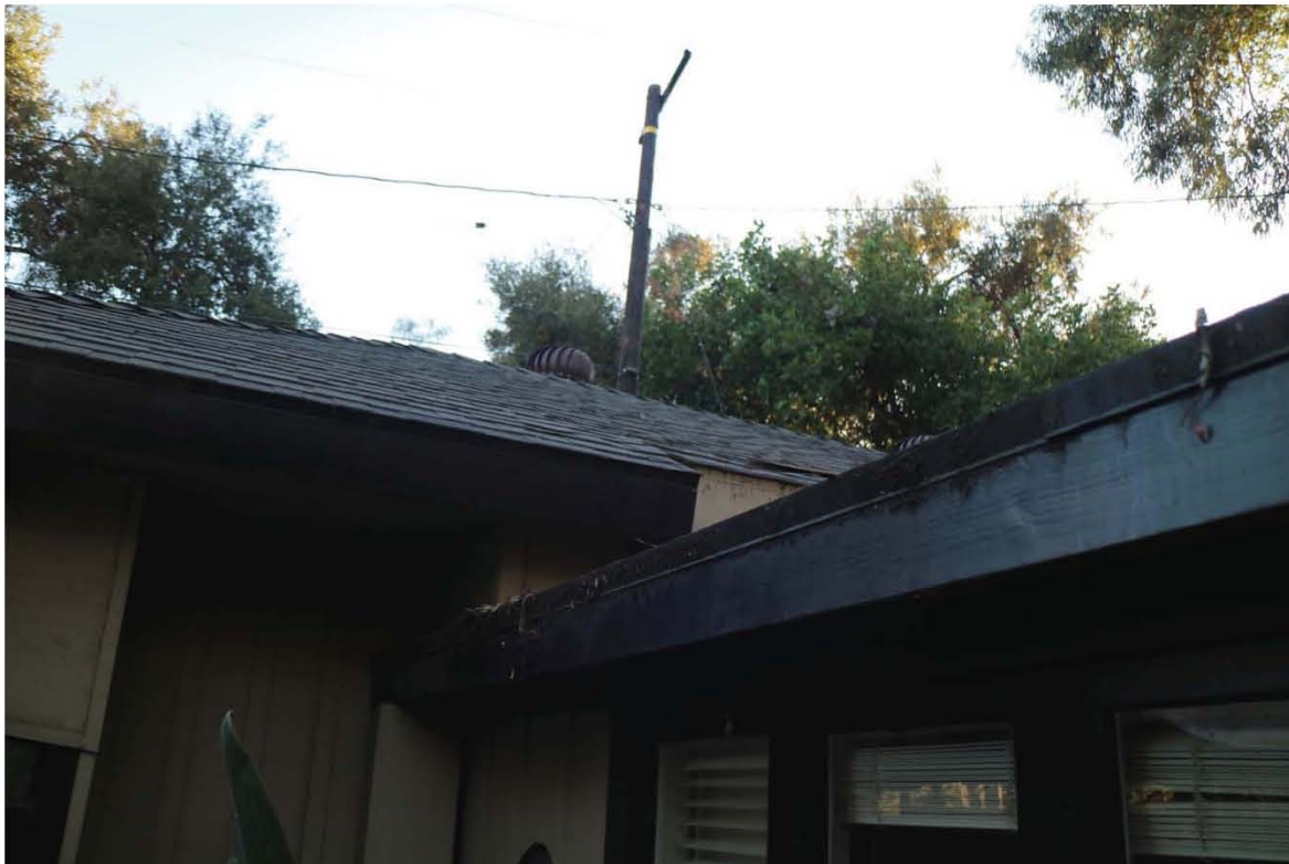
Figure 5. Smith Residence, detail of exterior roof juncture (top) and area of interior ceiling with water penetration, Living Room (bottom)
