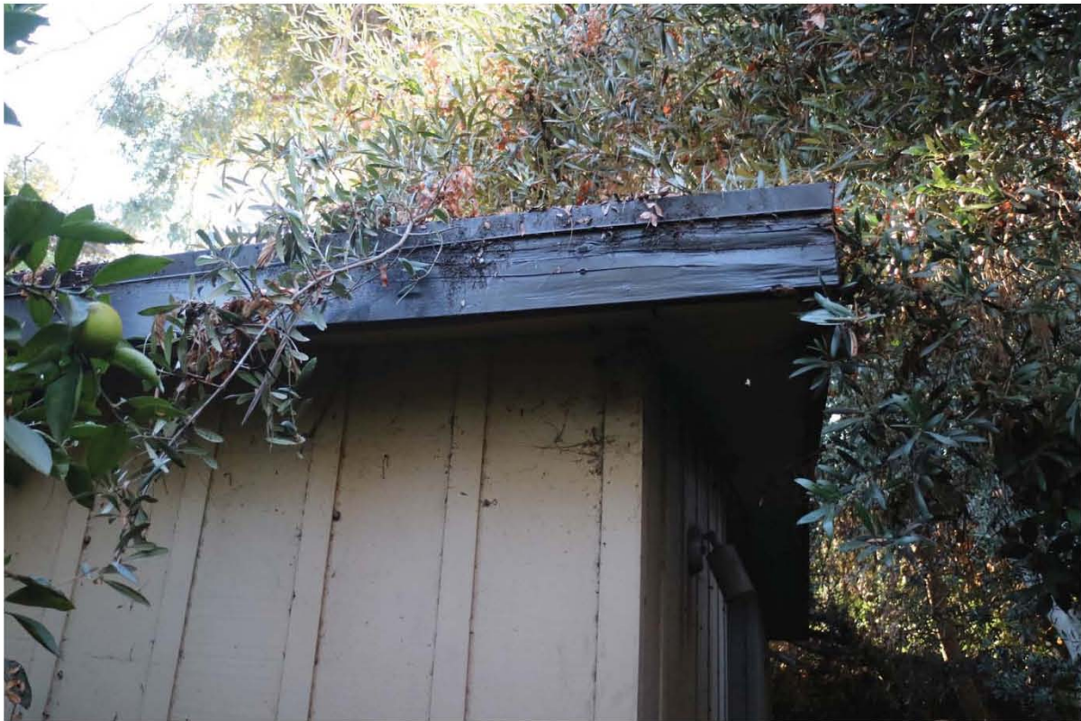
Figure 9. Smith Residence, roof features and segments in need of water proofing, repairs and rehabilitation
