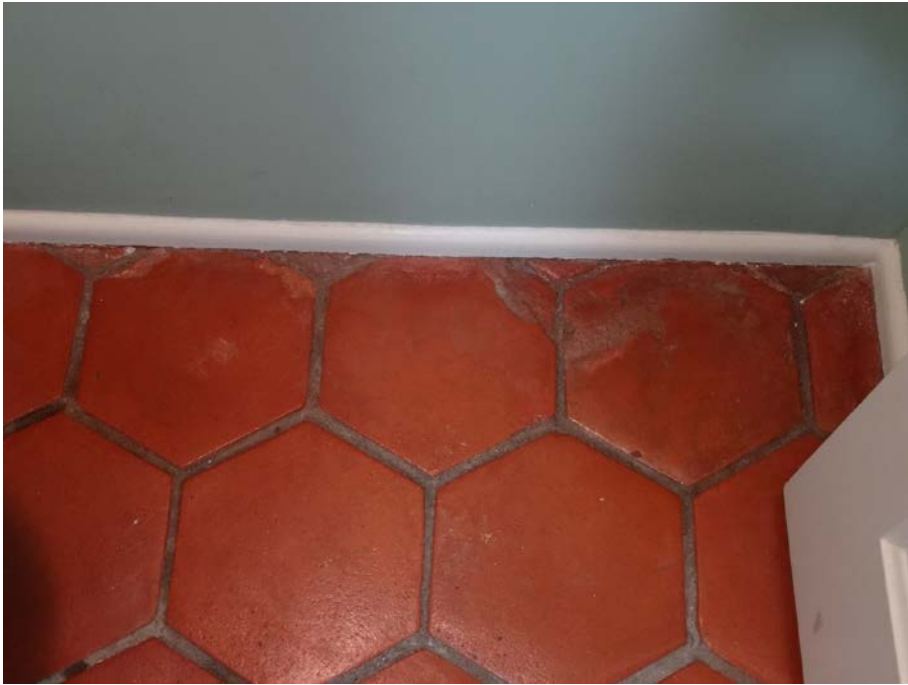
Terracotta floor tiles to be repaired
