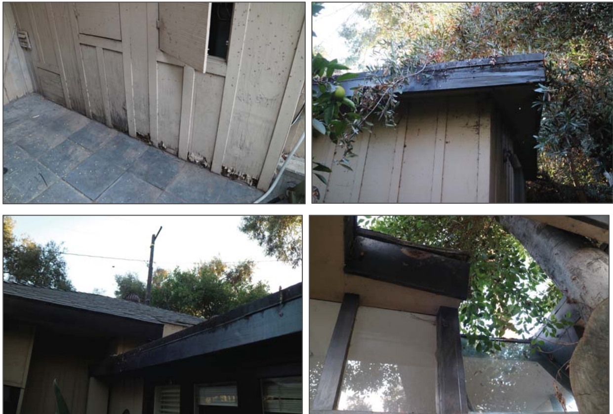
Figure 1. Overview of wood elements and features in need of repair/replacement
