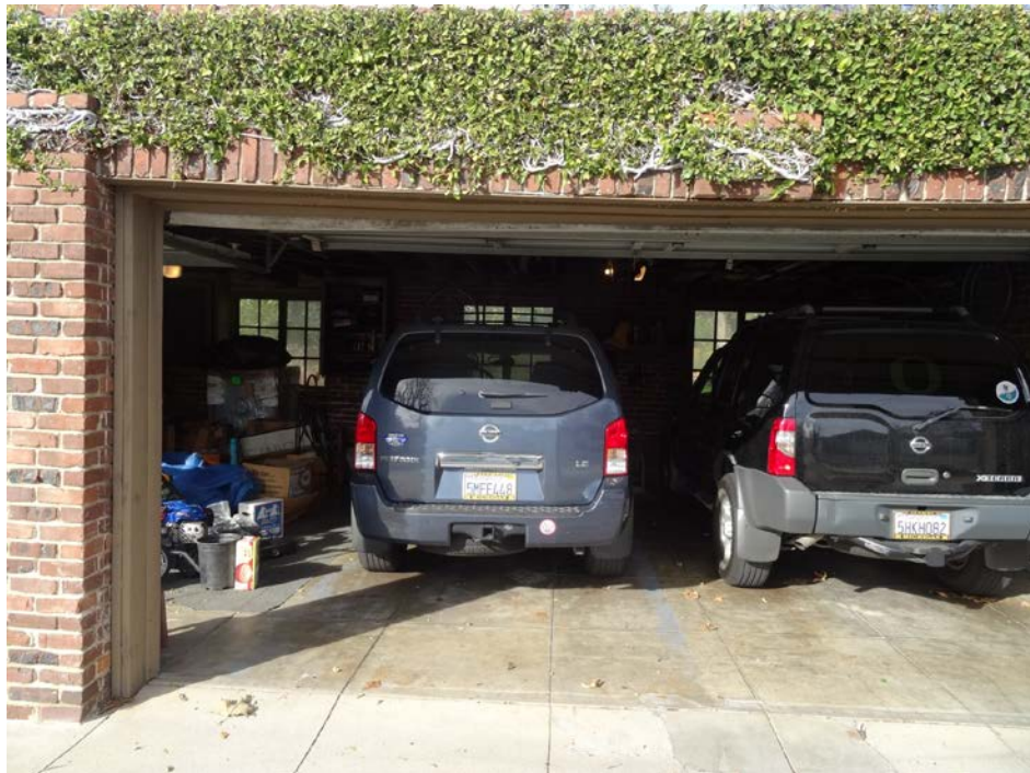
Garage opening beam to be reinforced
