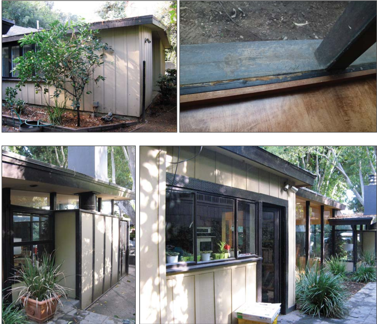
Figure 2. Overview of areas in need of repainting and refinishing following repairs
