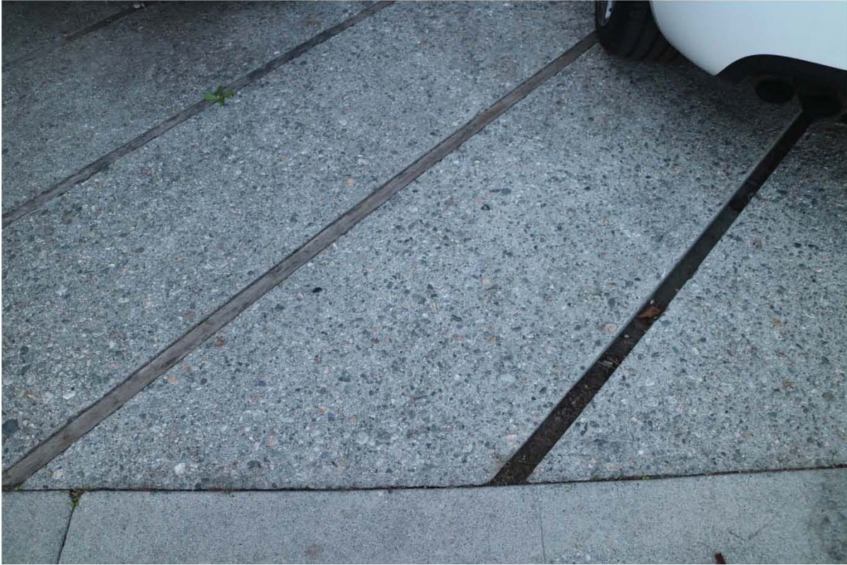
Figure 14. Smith Residence, character-defining hardscaping in need of repairs
