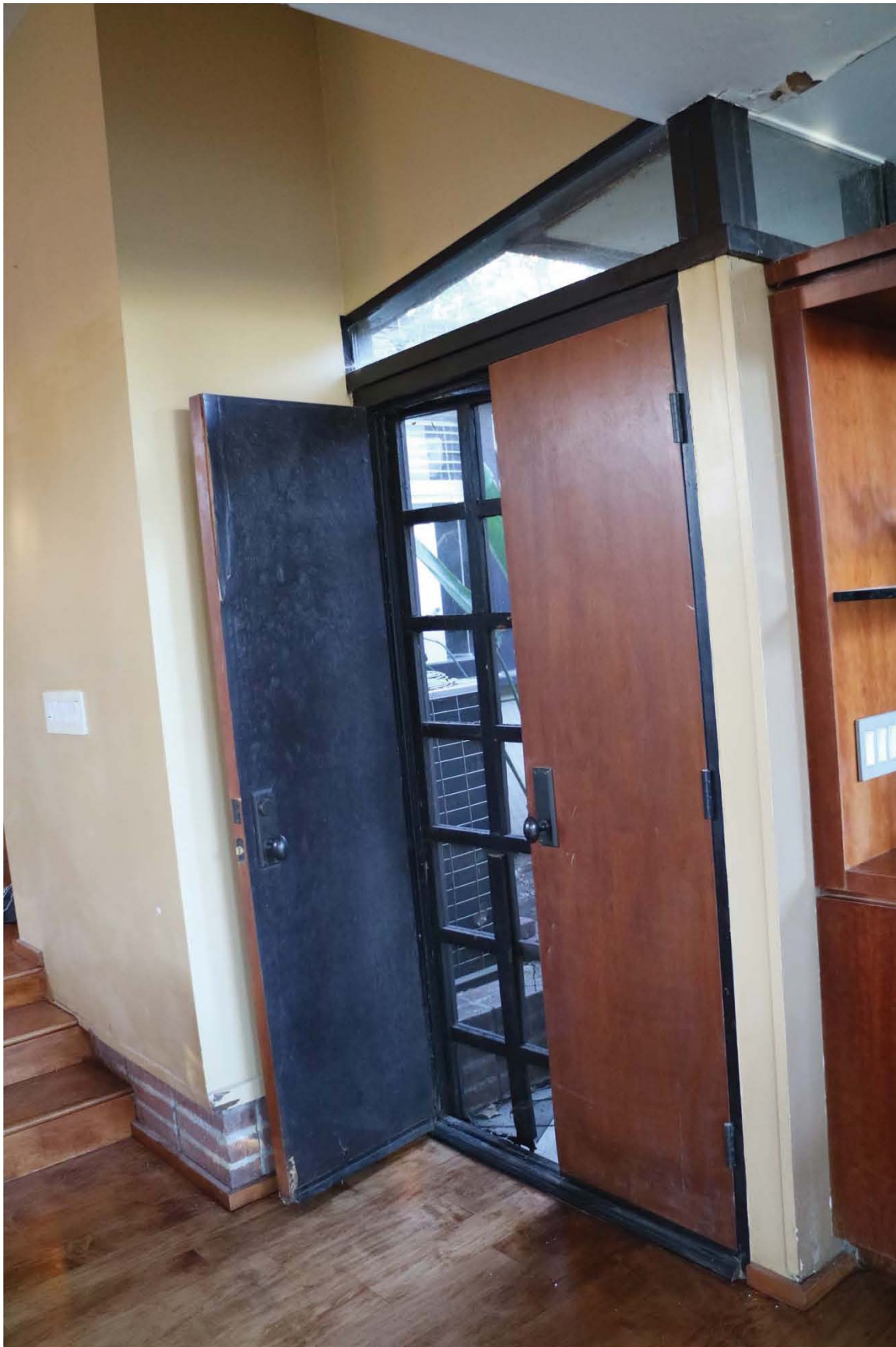
Figure 12. Smith Residence, wood elements and features in need of repairs and rehabilitation; north elevation entrance door and wood screen
