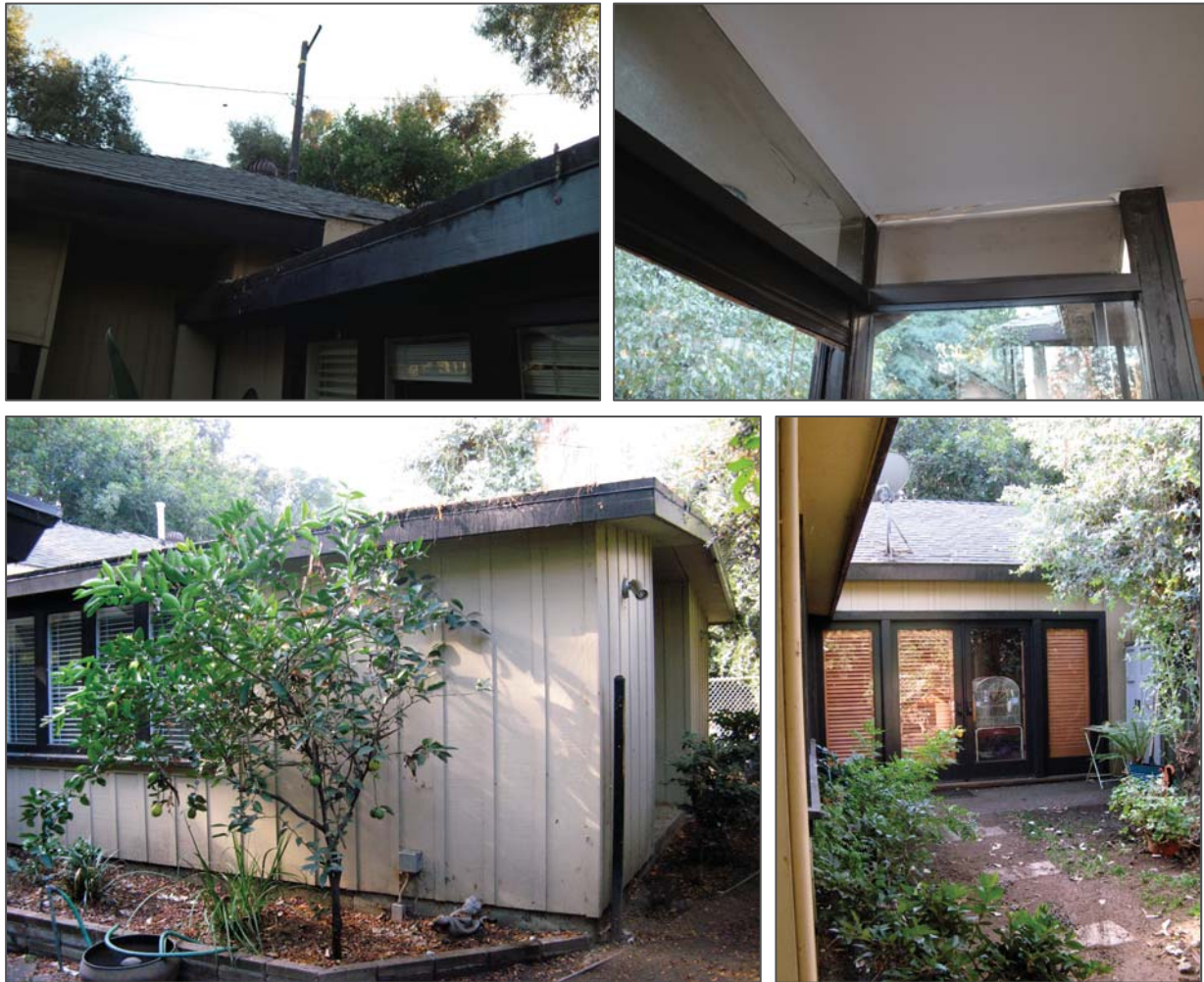
Figure 1: Overview of issues and areas in need of repair and waterproofing
