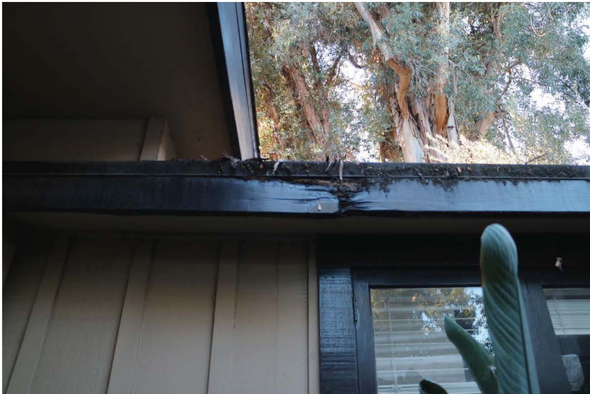
Figure 8. Smith Residence, roof features and segments in need of water proofing, repairs and rehabilitation
