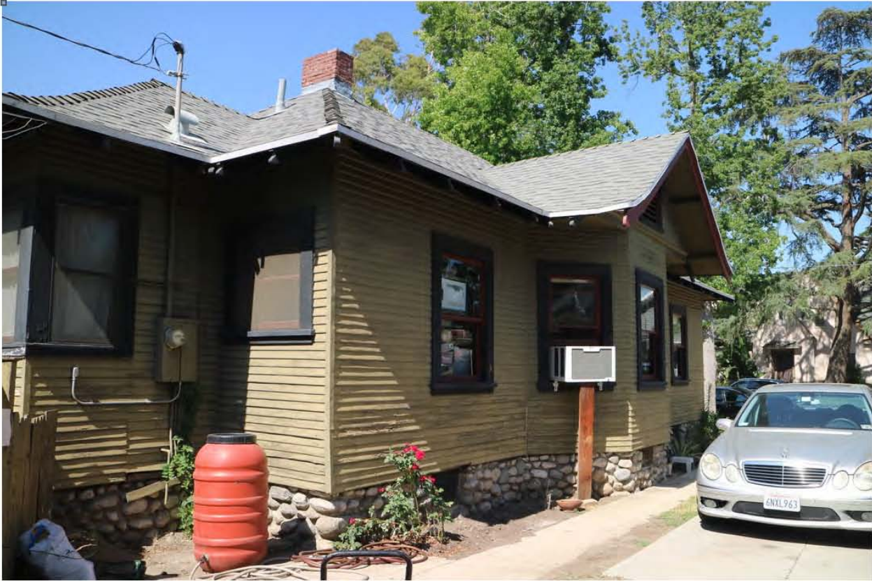
Figure 5. Original wood-frame windows; many are inoperable, all need repainting and re-weather sealing
