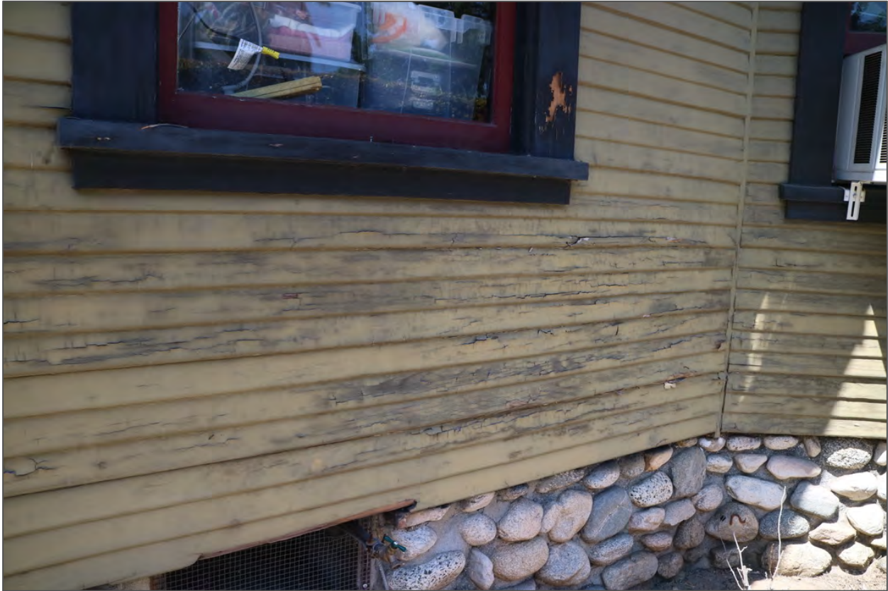
Detail, horizontal wood-siding, areas in need of repair and repainting, south elevation
