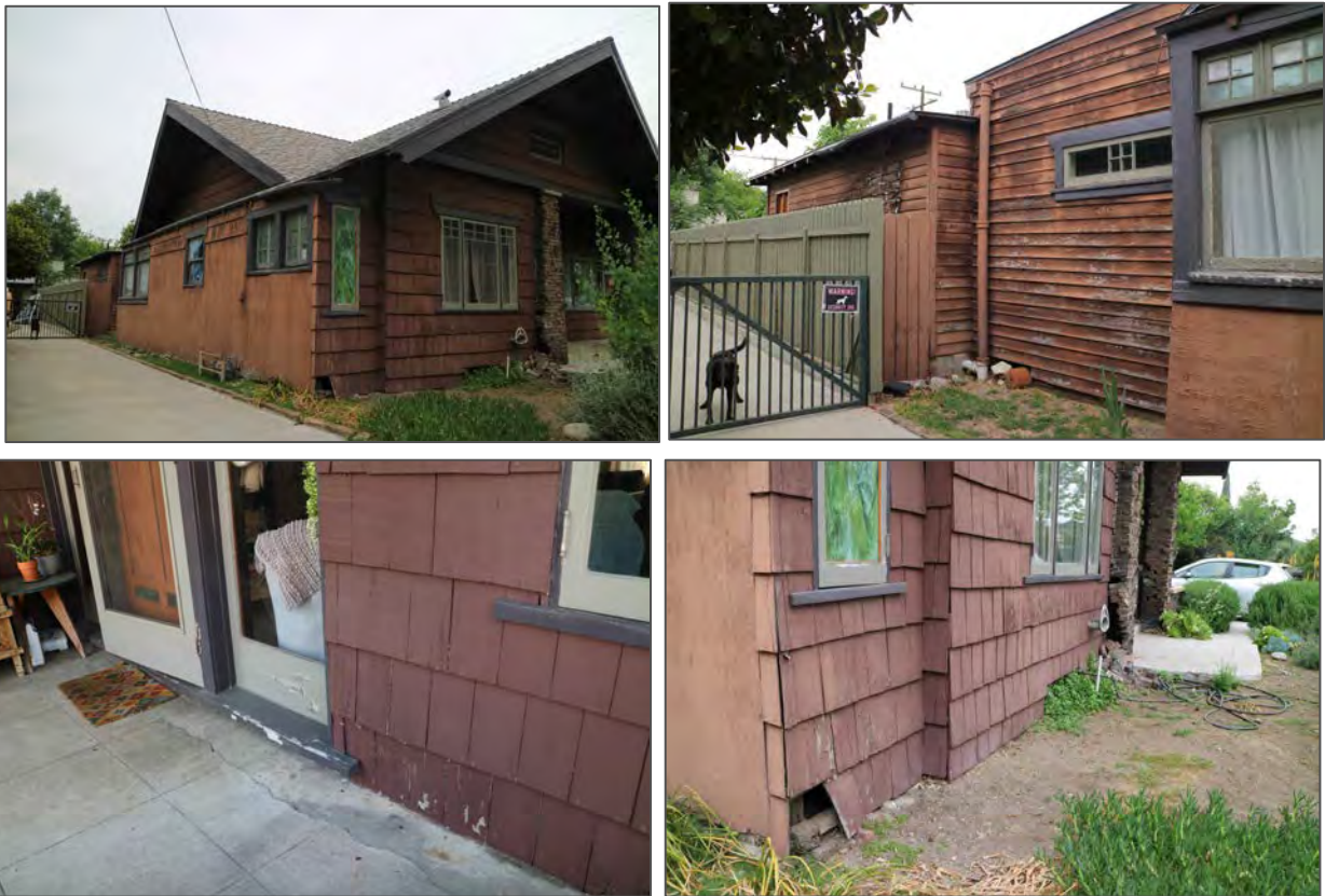
Figure 2. Overview of wood shingles in need of repair/replacement and repainting
