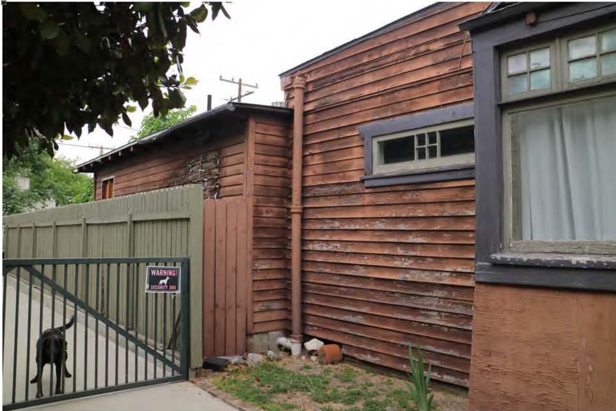
Figure 9. Overview of wood shingles in need of repair/replacement and repainting
