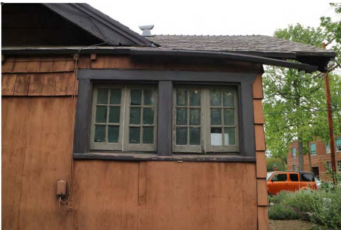
Figure 10. South elevation windows in need of repairs/in-kind replacement
