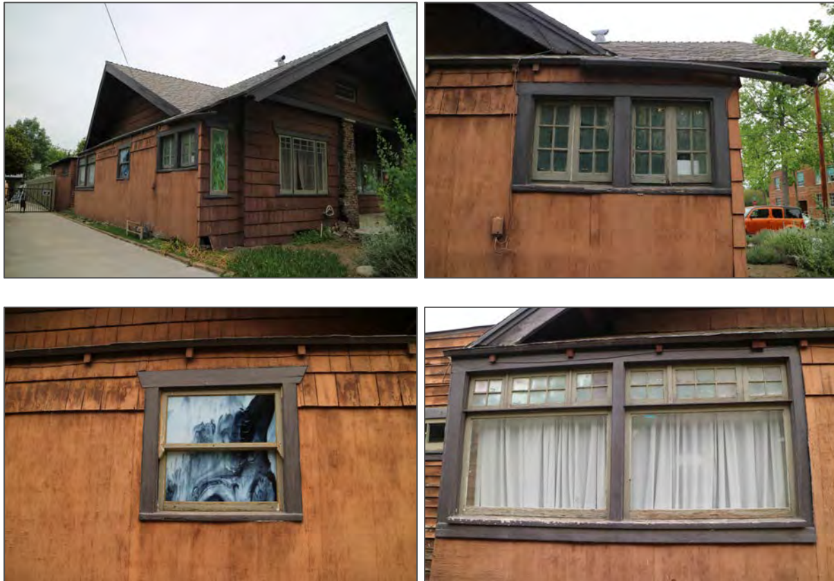
Figure 3. South elevation windows in need of repairs/in-kind replacement
