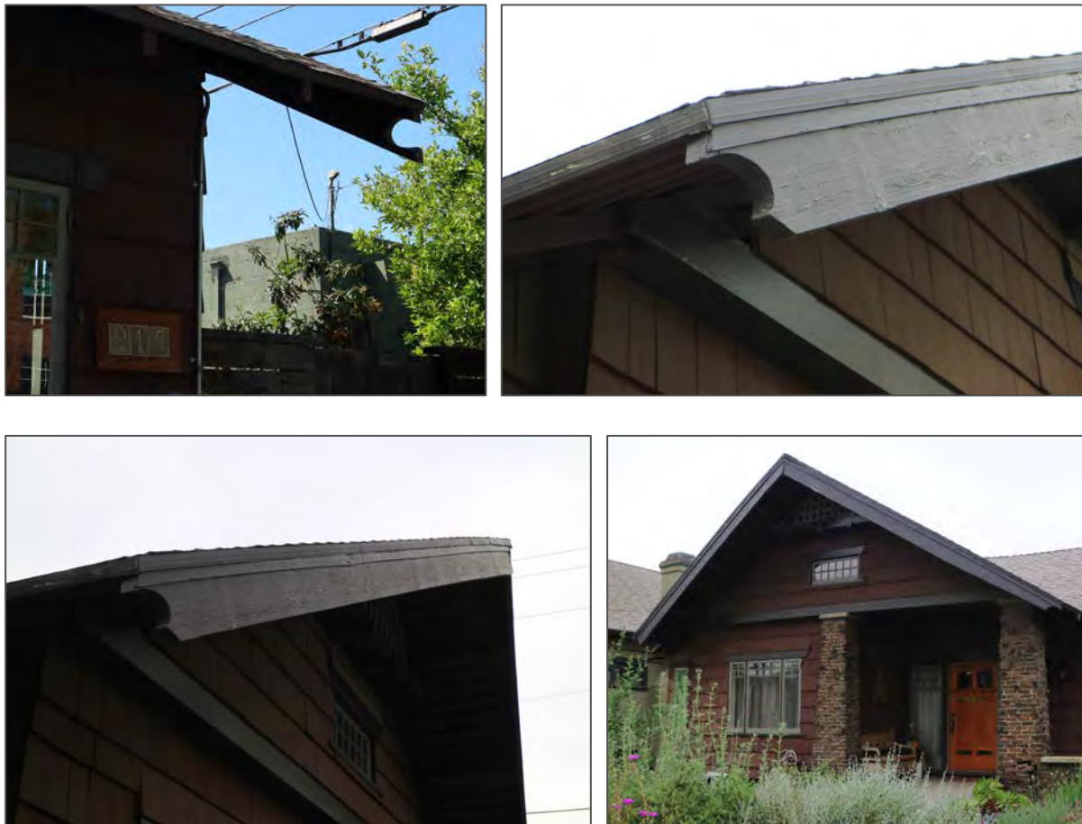
Figure 4. Roof features – bargeboard and decorative rafter tail to be re-created and repaired
