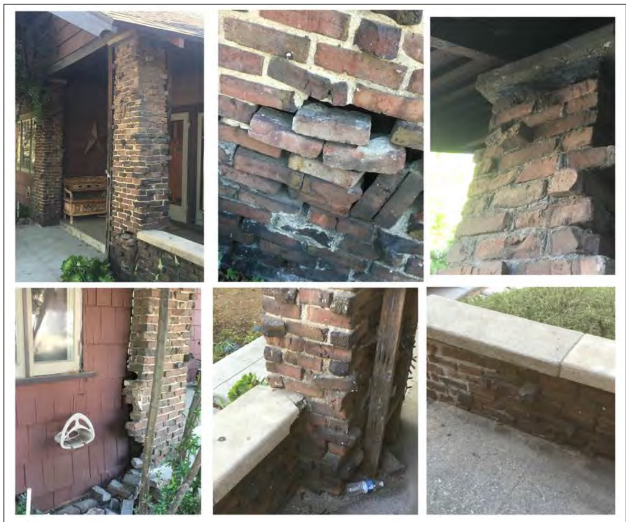
Figure 1: Overview of issues, clinker brick porch features
