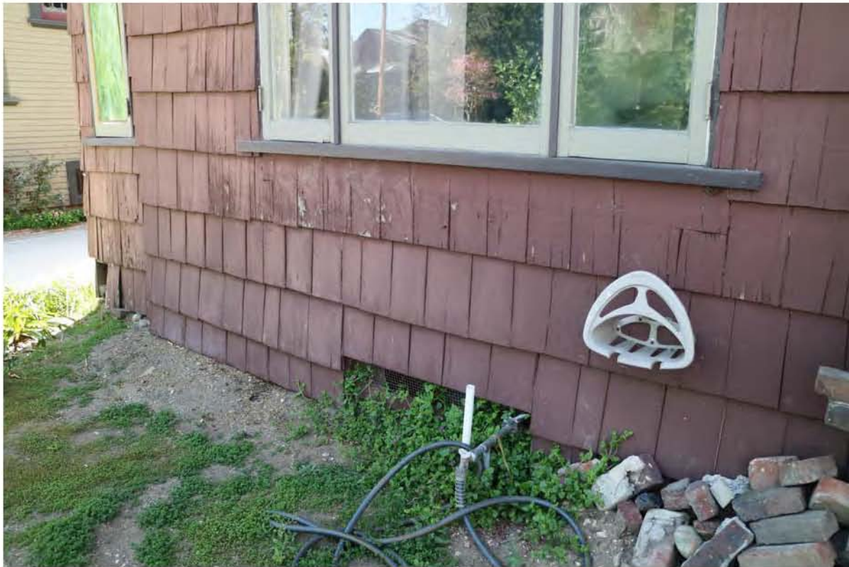
Figure 8. Overview of wood shingles in need of repair/replacement and repainting
