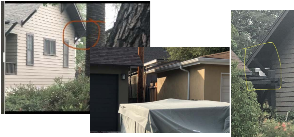
Figure 1: Photos of Unpermitted Patio Cover From Street
