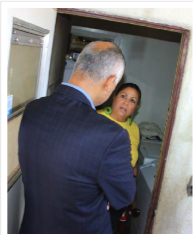
Cracked doors and leaky plumbing- Resident Carlene Ward shows Hernandez her cracked doors and walls and the substandard plumbing that Caltrans will not let her fix. Photos by Randy Economy.
