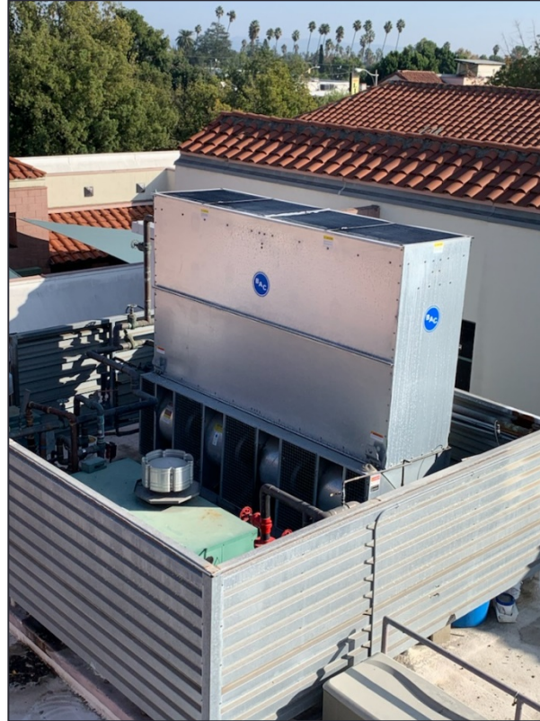
City Hall HVAC System
