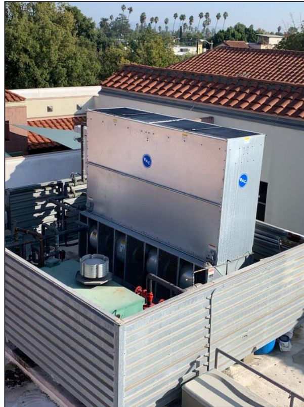
City Hall HVAC System
