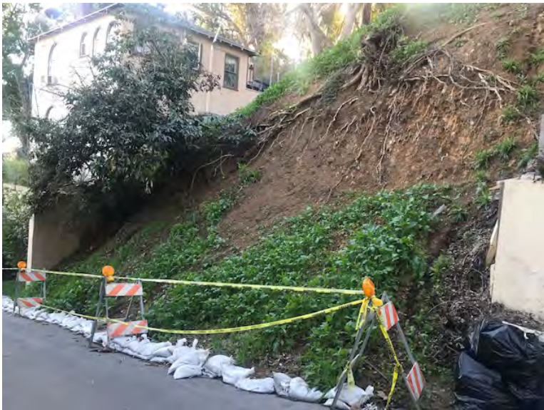
3 lost parking spaces due to unstable hillside. Bonita and Oneonta Drs. are restricted to parking on one-side only.
