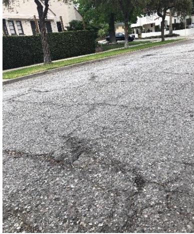
Description: Sever thermal cracking and surface unravelling at Forest Ave.
