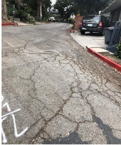
Description: Severe Aligator Cracking at Alta Vista Avenue
