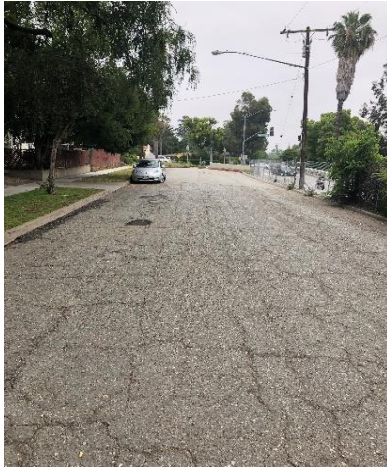
Description: Block cracking and surface unravelling at Sterling Place
