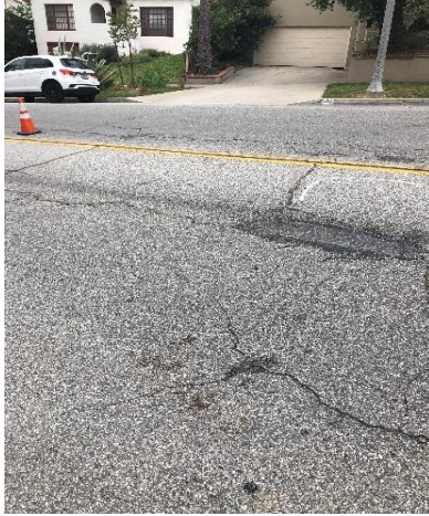
Description: Block Cracking and Thermal Cracking at Monterey Road
