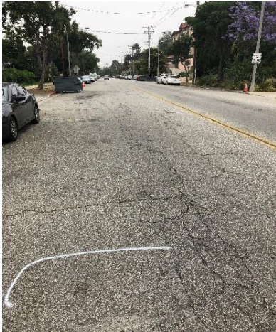
Description: Alligator Cracking on the wheelpath at Monterey Road
