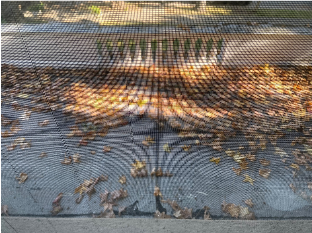
Damaged roof of the porch
