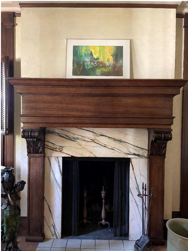
One of three fireplaces to be repaired
