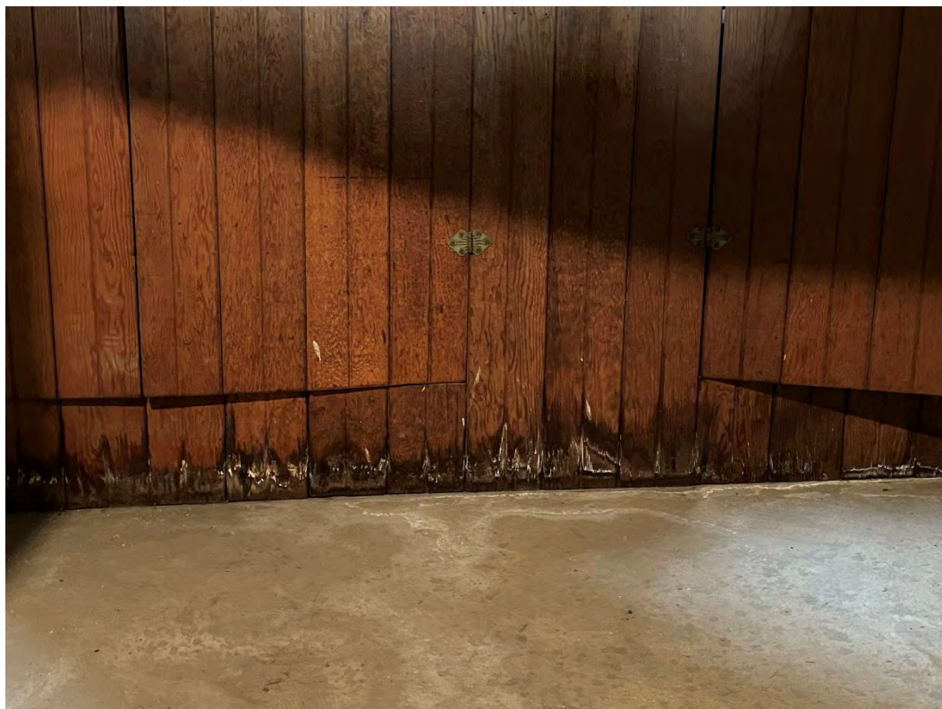
Evidence of drainage issues in the basement
