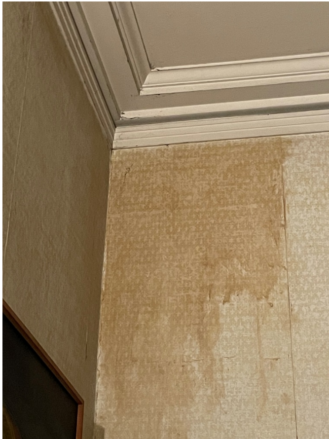
Evidence of roof leaks on the second floor
