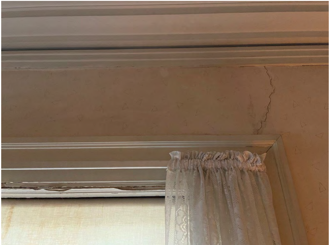
Interior cracks demonstrating structural damage
