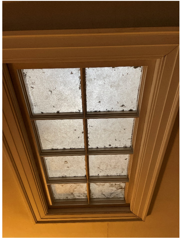
Staircase skylight to be repaired
