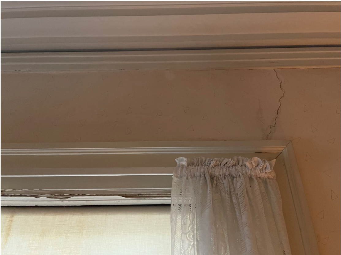
Interior cracks demonstrating structural damage
