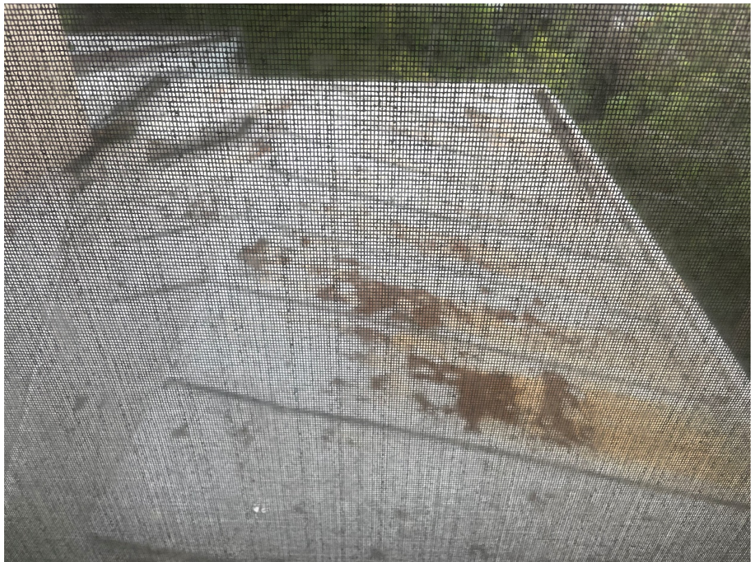
Damaged roof of the sun parlor
