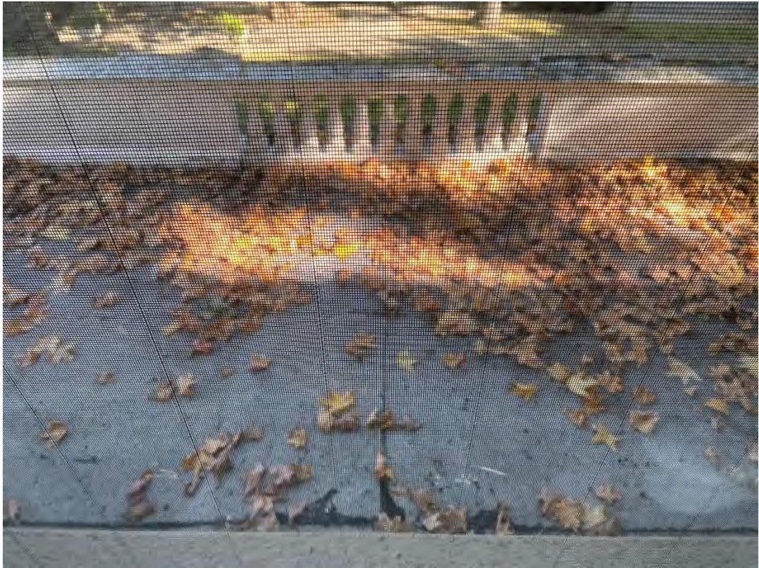
Damaged roof of the porch
