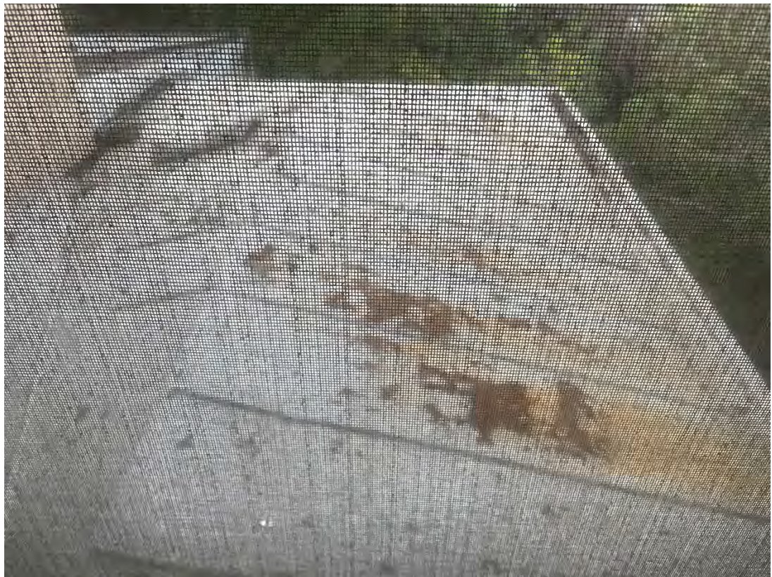
Damaged roof of the sun parlor
