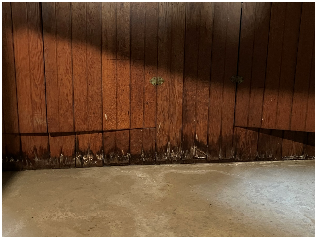
Evidence of drainage issues in the basement
