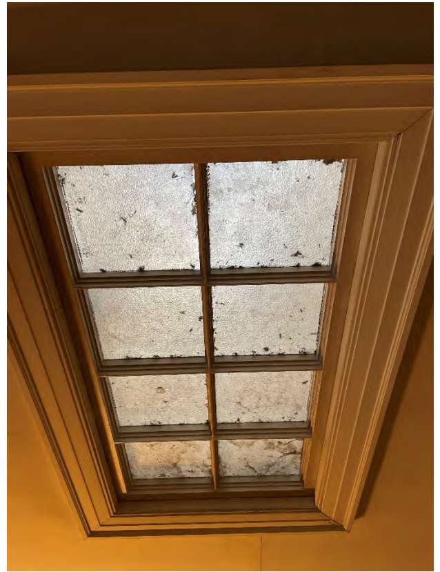
Staircase skylight to be repaired
