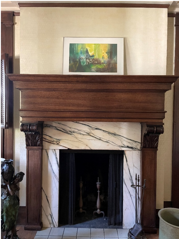
One of three fireplaces to be repaired
