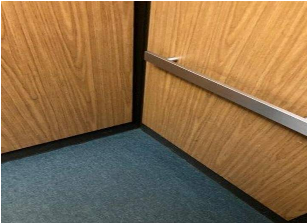
104 - Non-compliant elevator cab interior handrail.
