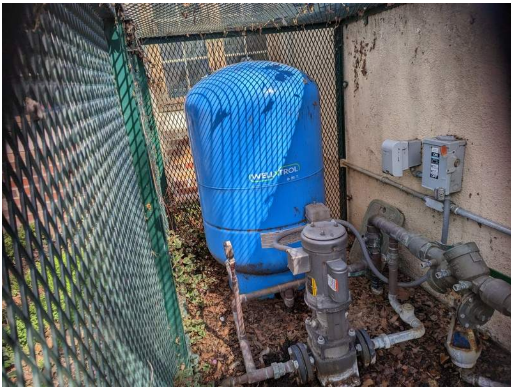
78 - Water pressure booster pump and pressure tank.
