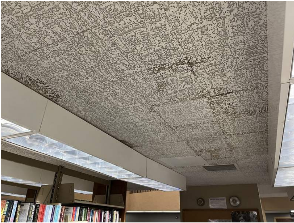
56 - Water damage on the acoustical ceiling in the Reading Room.
