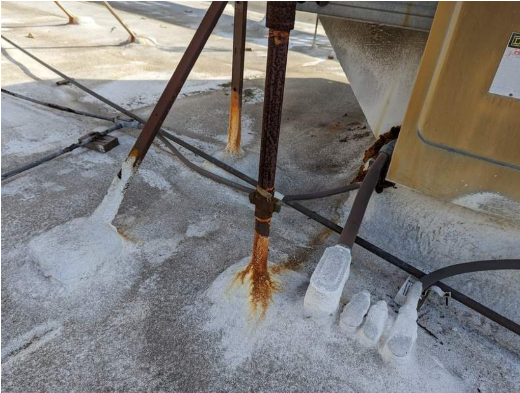
75 - Corroded natural gas piping at the roof.
