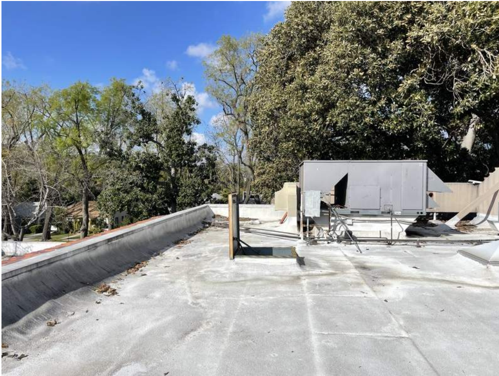
27 - Low-slope roof with multi-ply, built-up roofing and SPF overlay coated with elastomeric protection coating.
