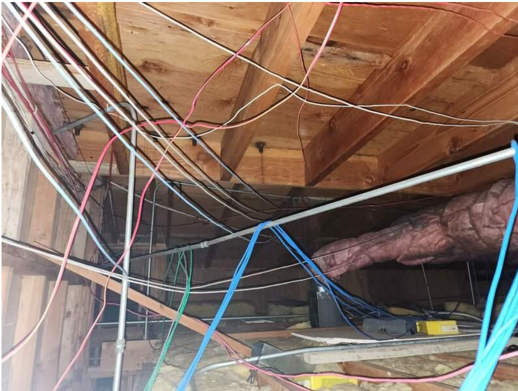
25 - Sawn lumber joists and plywood sheathing at roof framing of the 1982 renovation.
