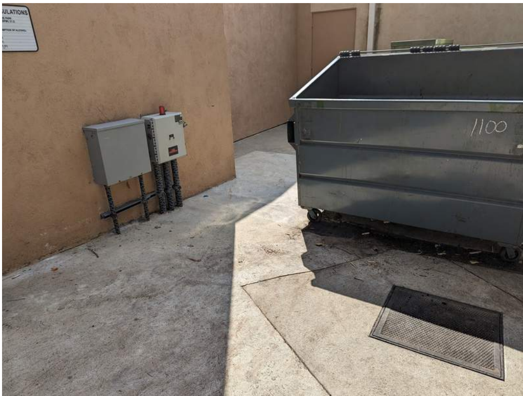
80 - Sump pump inlet grate and controller at the service yard.
