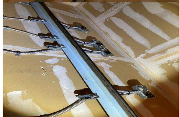
Top of hoistway and hoistway switches
