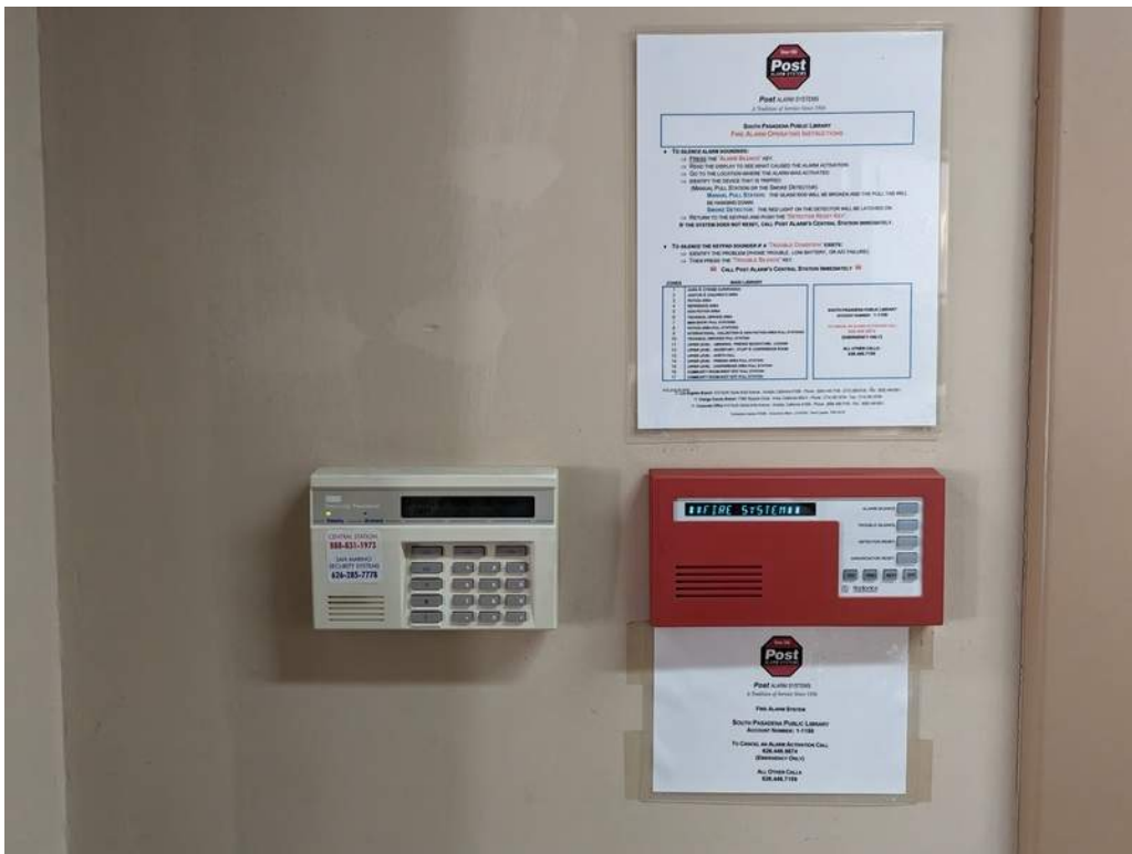
106 - Security panel and fire alarm annunciator panel.
