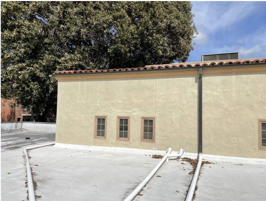
30 - Gutter and downspout at the pitched roof eave. Note PVC drain pipes provided without sleepers.
