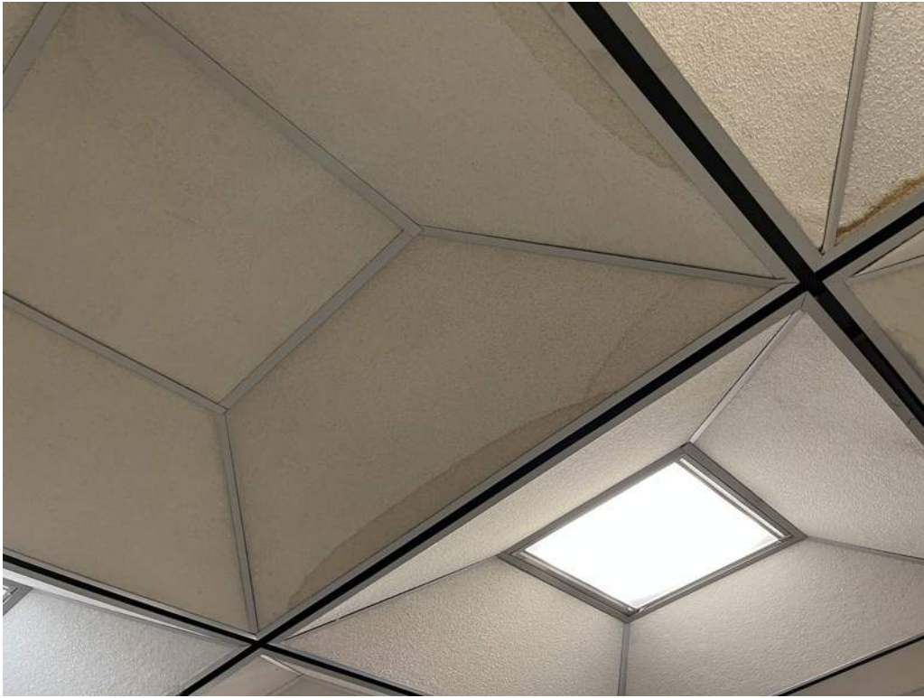
53 - Water damage at the Children's Reading Room acoustical ceiling.
