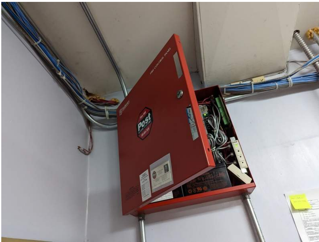
86 - Fire alarm control panel in the server room.
