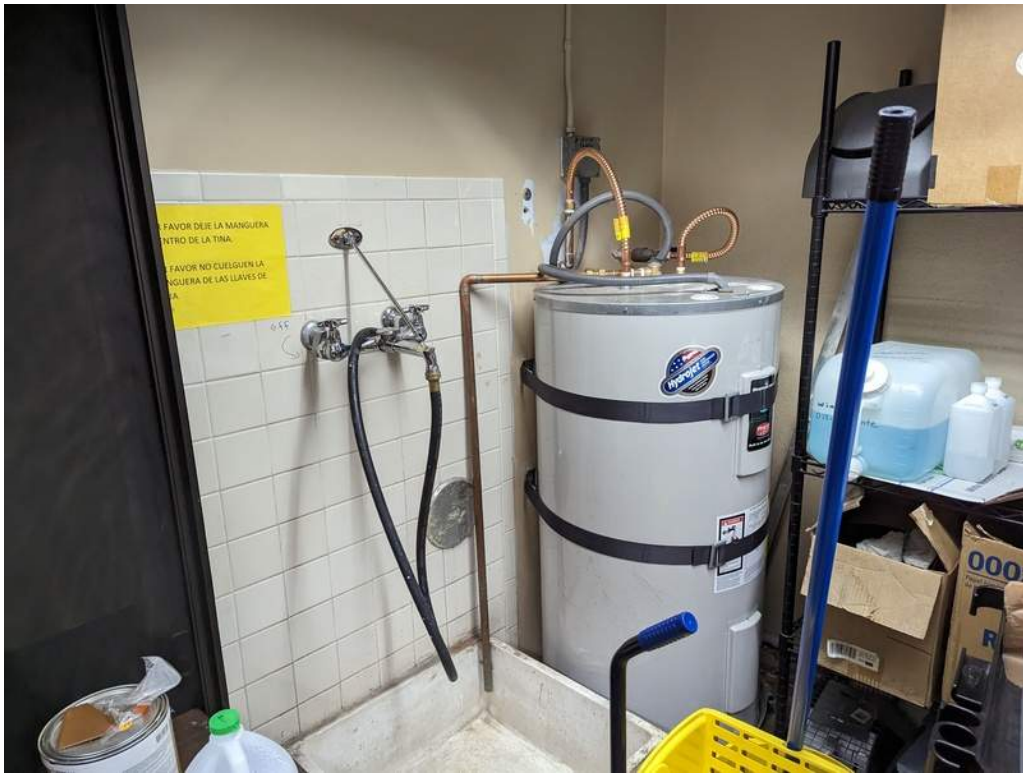
79 - Electric water heater in the janitor's closet.
