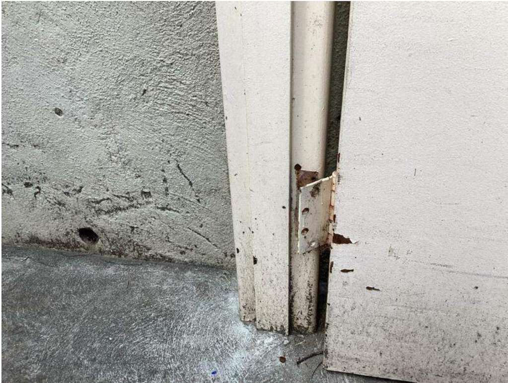
17 - Broken hinge at the service yard gate.
