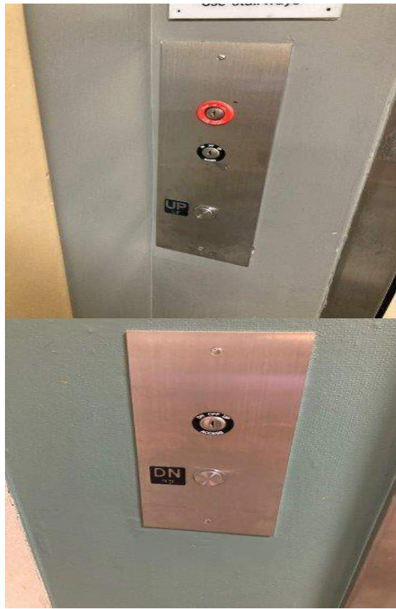
Elevator hall fixtures (2013)
