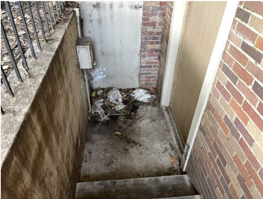
2 - Surface drain at the egress stairwell with debris build-up.
