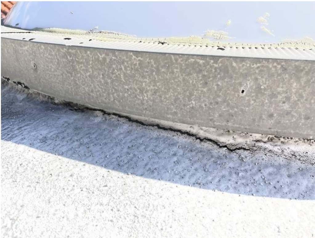
45 - Cracked sealant at the circular dome skylight.
