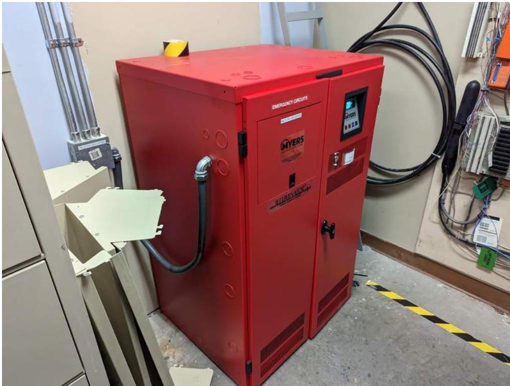
85 - Emergency power supply system in the server room.
