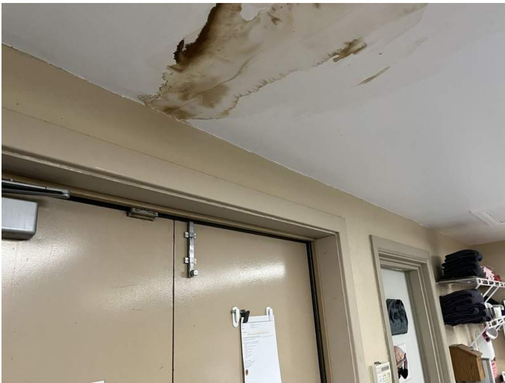
62 - Water damage at the staff area ceiling.
