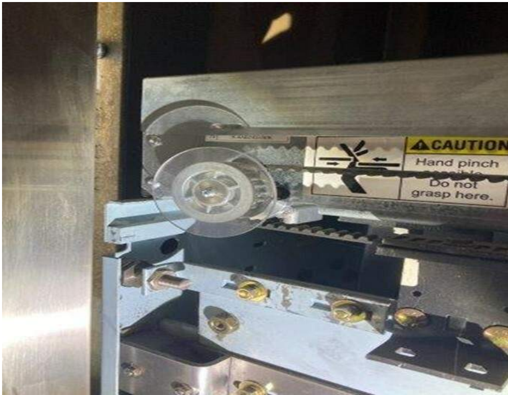
91 - Otis AT 400 linear car door operator (2013).
