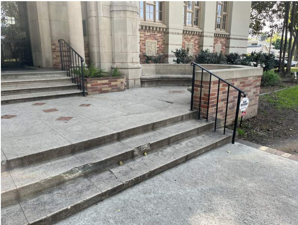
99 - Handrails with non-compliant handrail extensions at the entrance to the Community Room.
