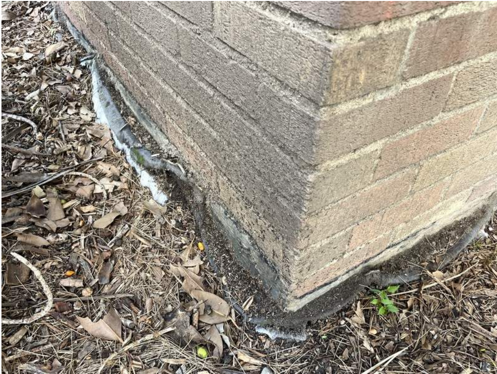
37 - The visible edge of the below-grade waterproofing is deteriorated and not provided with termination bar and counter flashing.
