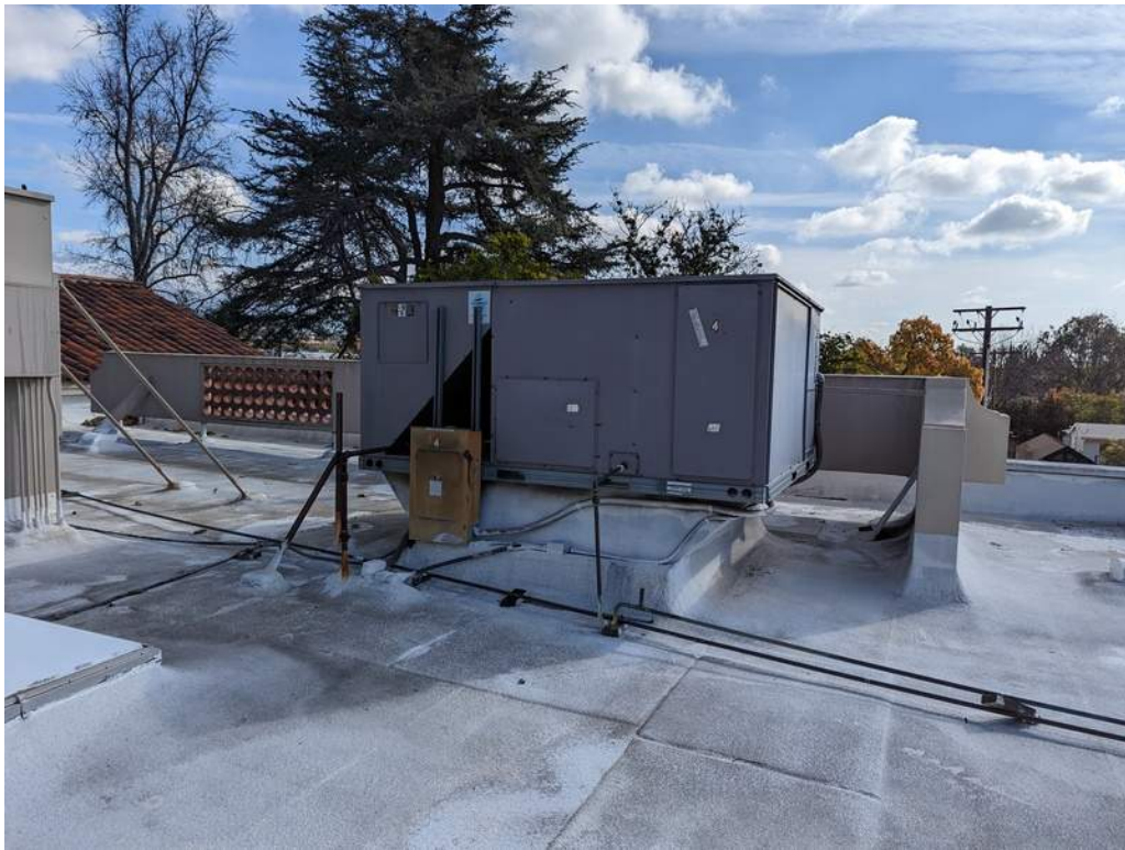
70 - Rooftop packaged unit with electrical disconnect, condensate drain, and natural gas piping.
