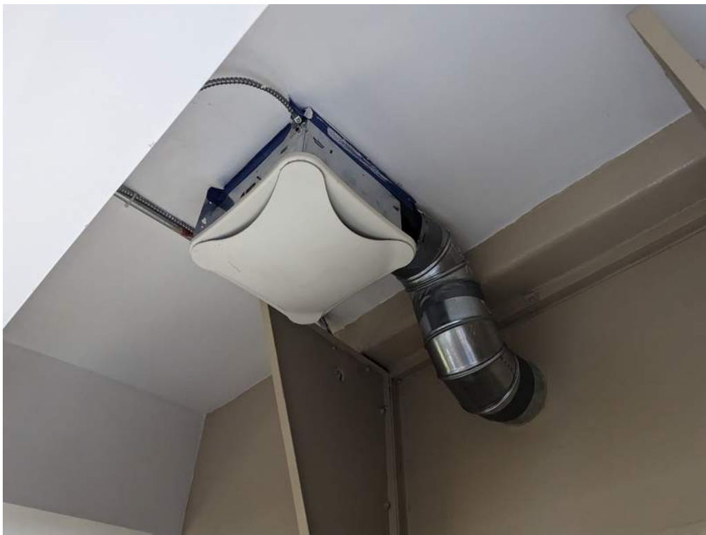
72 - Ceiling-mounted exhaust fan in the janitor's closet.
