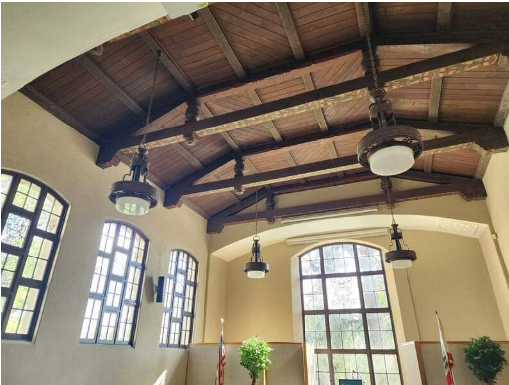
23 - Wood trusses and original sheathing at the roof framing of the Community Room.
