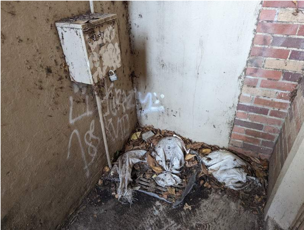
81 - Sump pump inlet at west stair landing with debris covering inlet.
