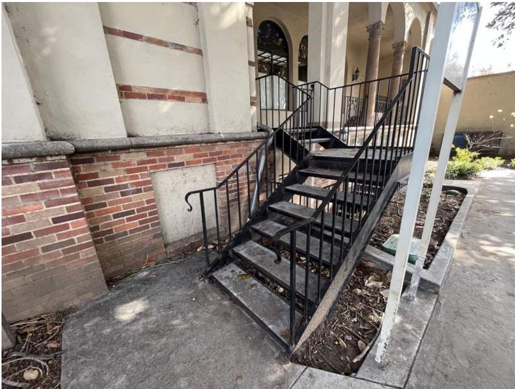
95 - Exterior egress stair with missing handrail extension and open treads.
