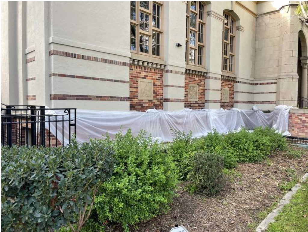
36 - Northeast corner of building with temporary plastic sheeting to reduce water infiltration into the basement.
