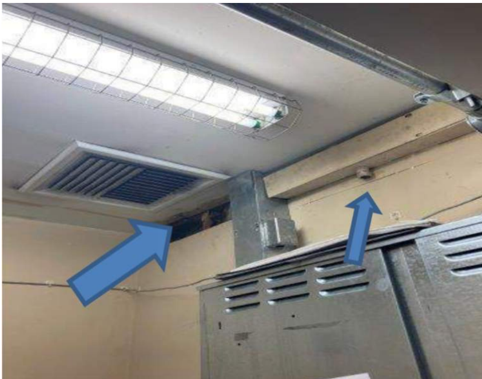
92 - Wall openings in the elevator machine room.
