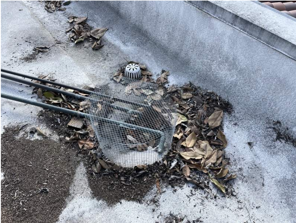
33 - Internal low-slope roof drain and overflow. Debris build-up noted.
