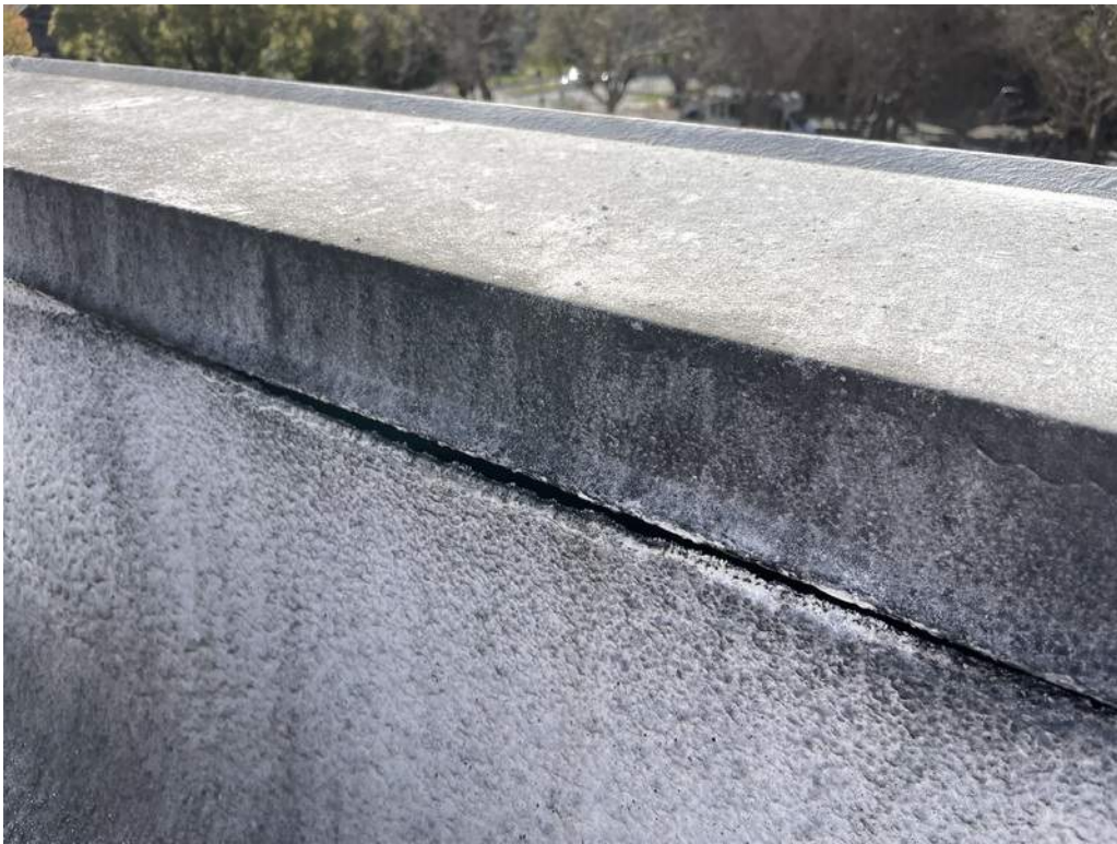
32 - The roofing termination at the parapet is separating providing a possible path for moisture intrusion.
