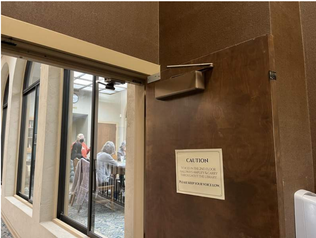
61 - Damaged door closer at the upper level.
