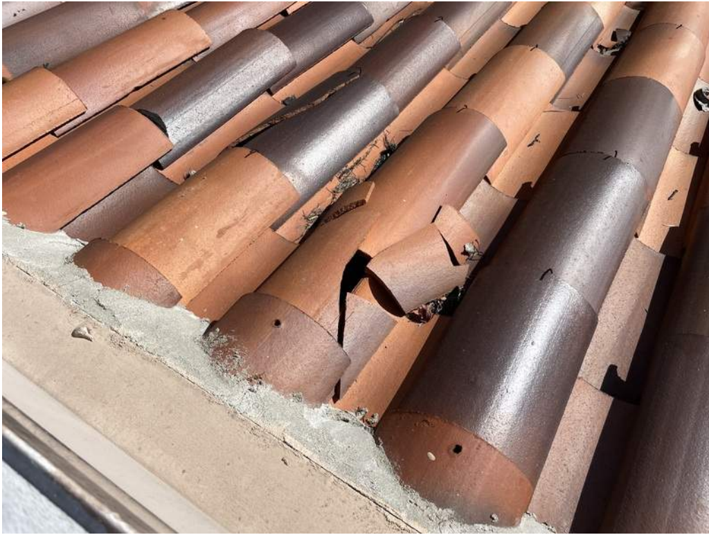
35 - Damaged clay tiles.
