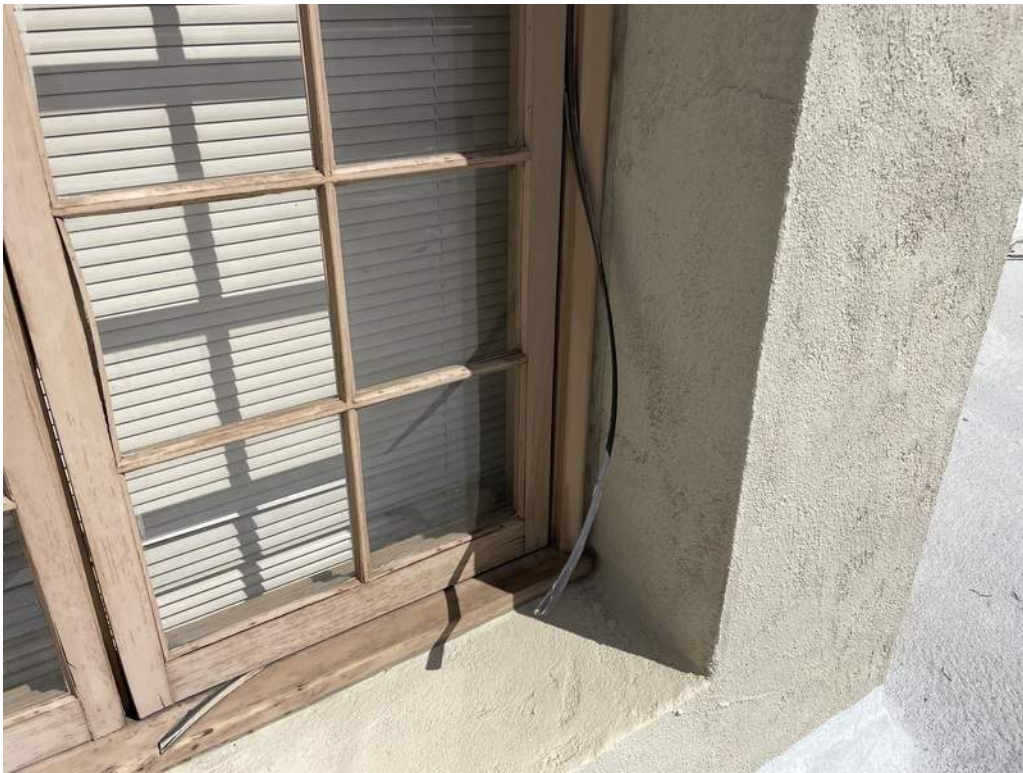
44 - Deteriorated and warped window with failed gaskets and paint.
