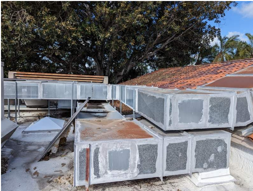
74 - Air ducts mounted on the roof. Ponding water on the top of deformed ducts noted.
