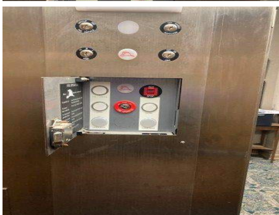
Car operating panel (2013)
