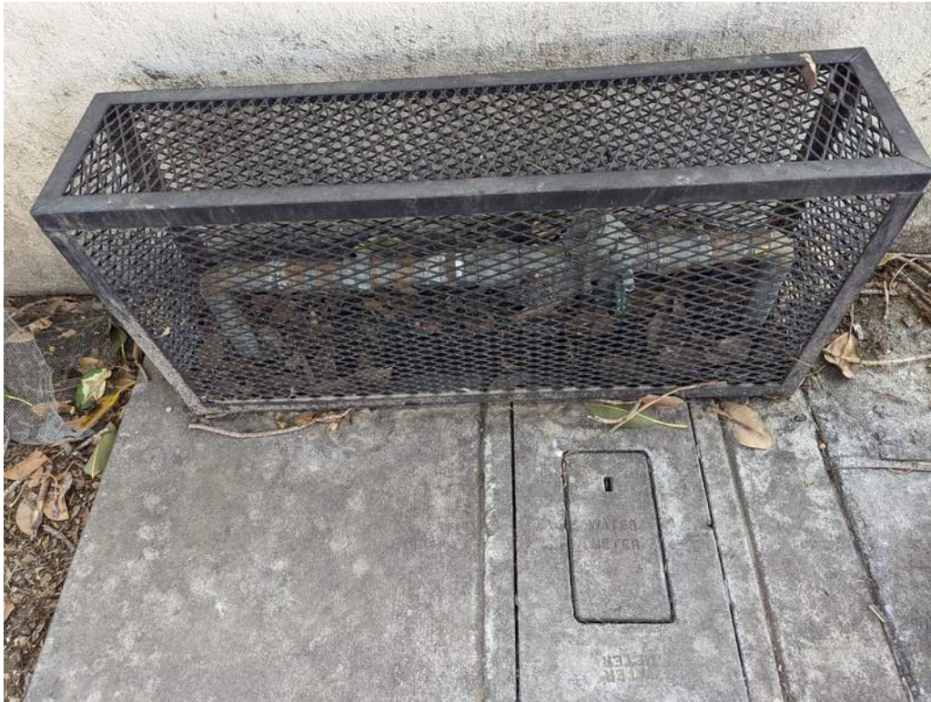
77 - Backflow prevention device and water meter.
