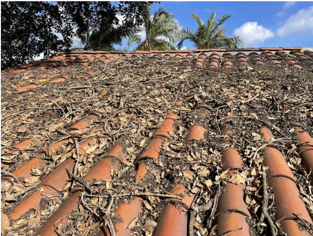
34 - Debris build-up on the clay tile roof.
