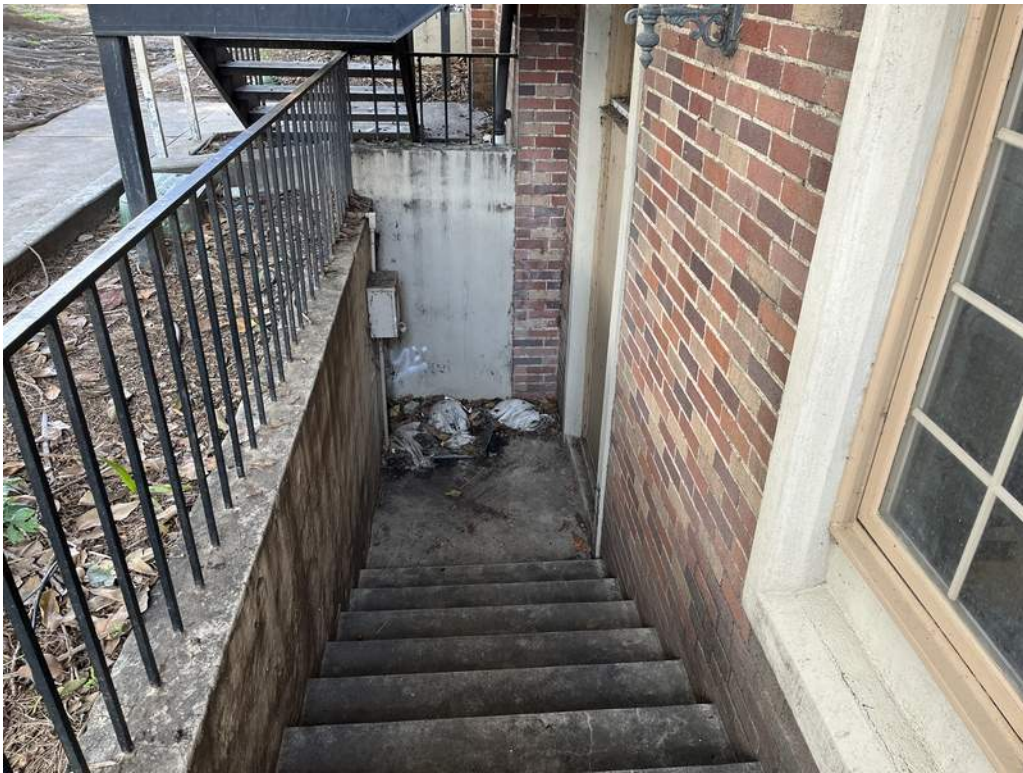
96 - Exterior egress stair with missing handrails.
