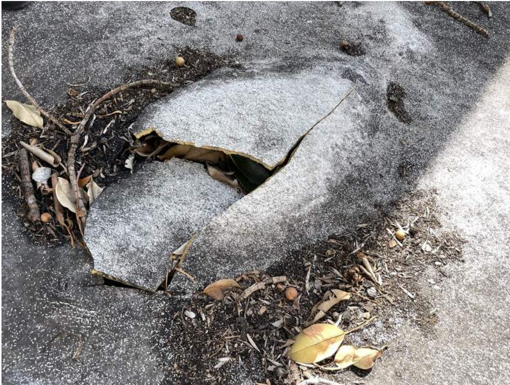
31 - Large ruptured blister in the spray foam roofing membrane.
