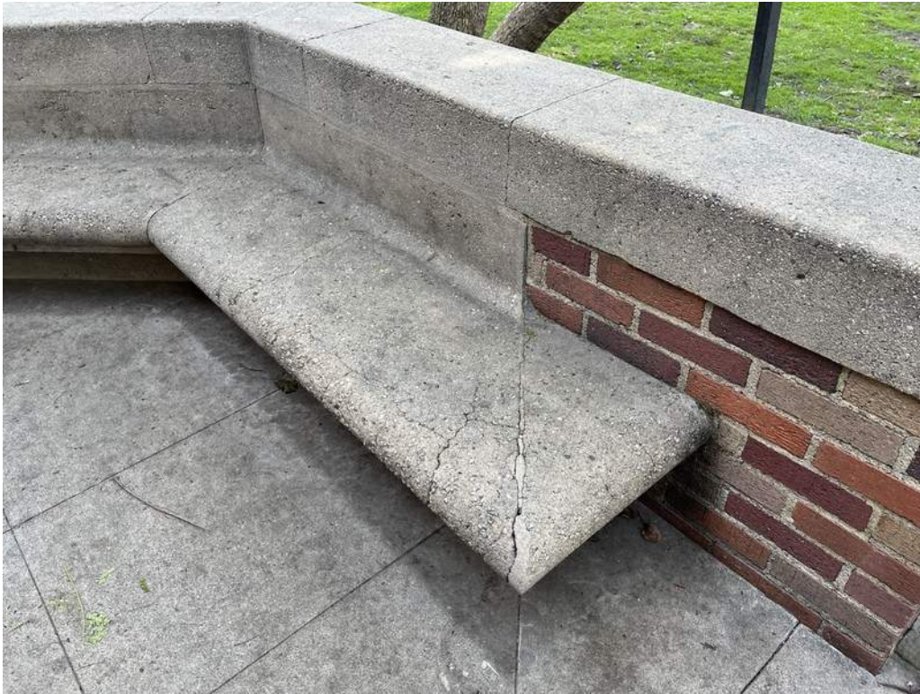
21 - Cracked concrete bench at the Community Room entrance.
