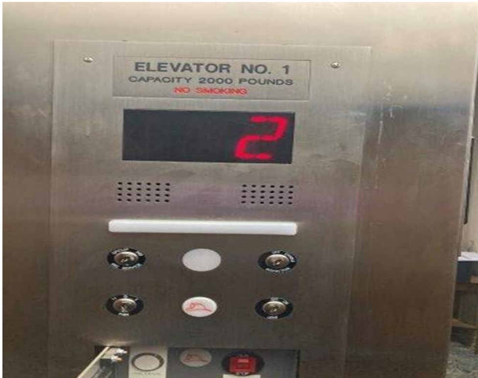
89 - Car operating panel (2013).
