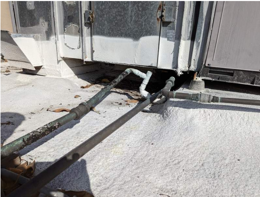
76 - Condensate drain askew and not draining properly.
