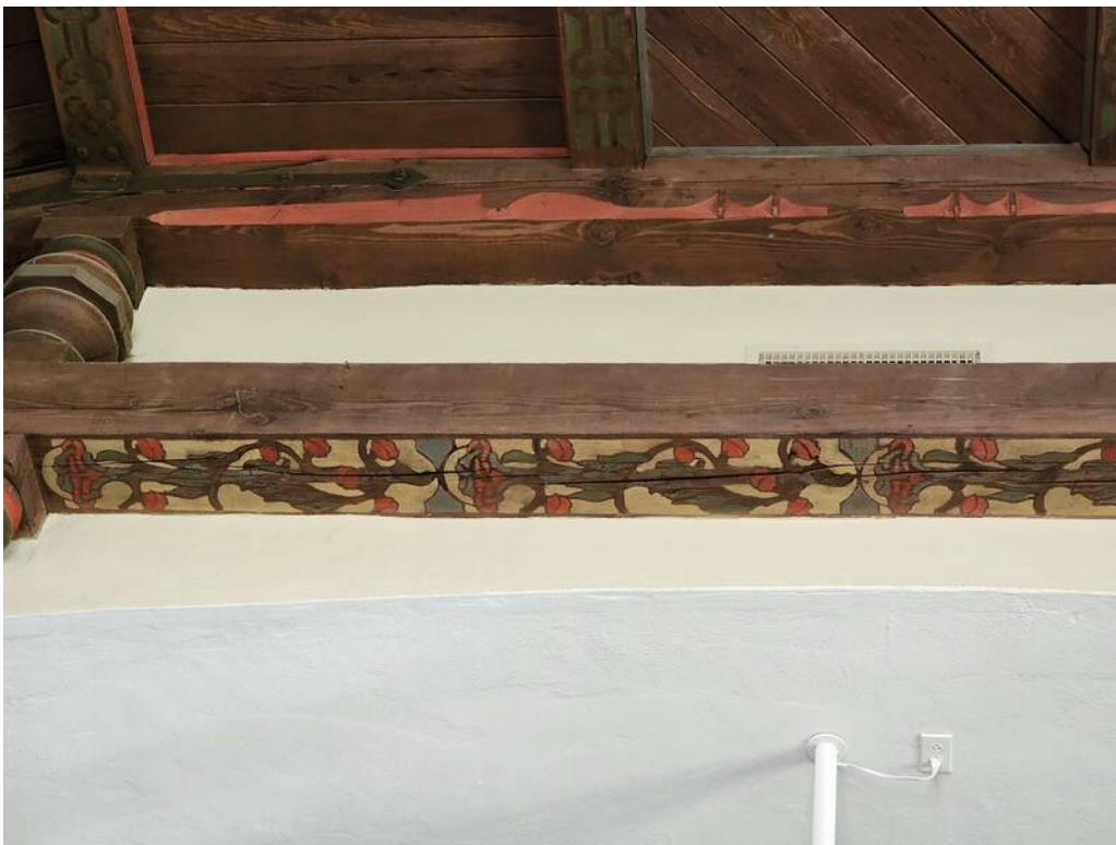
26 - Splits at bottom chords of the Community Room trusses.
