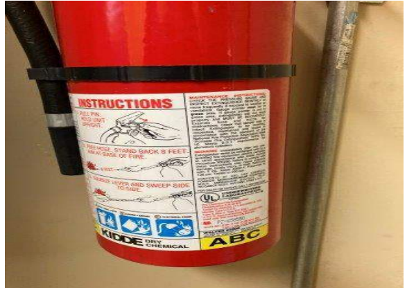
Elevator machine room ABC fire extinguisher
