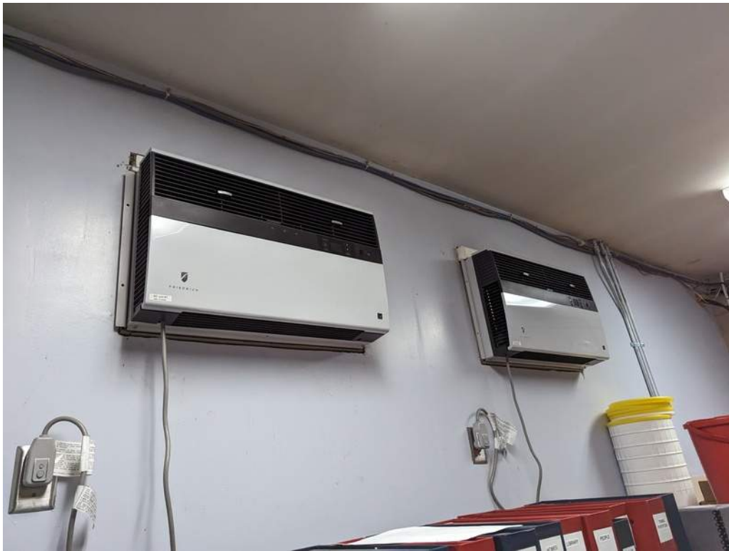
71 - Wall-mounted through-wall AC units in the server room.
