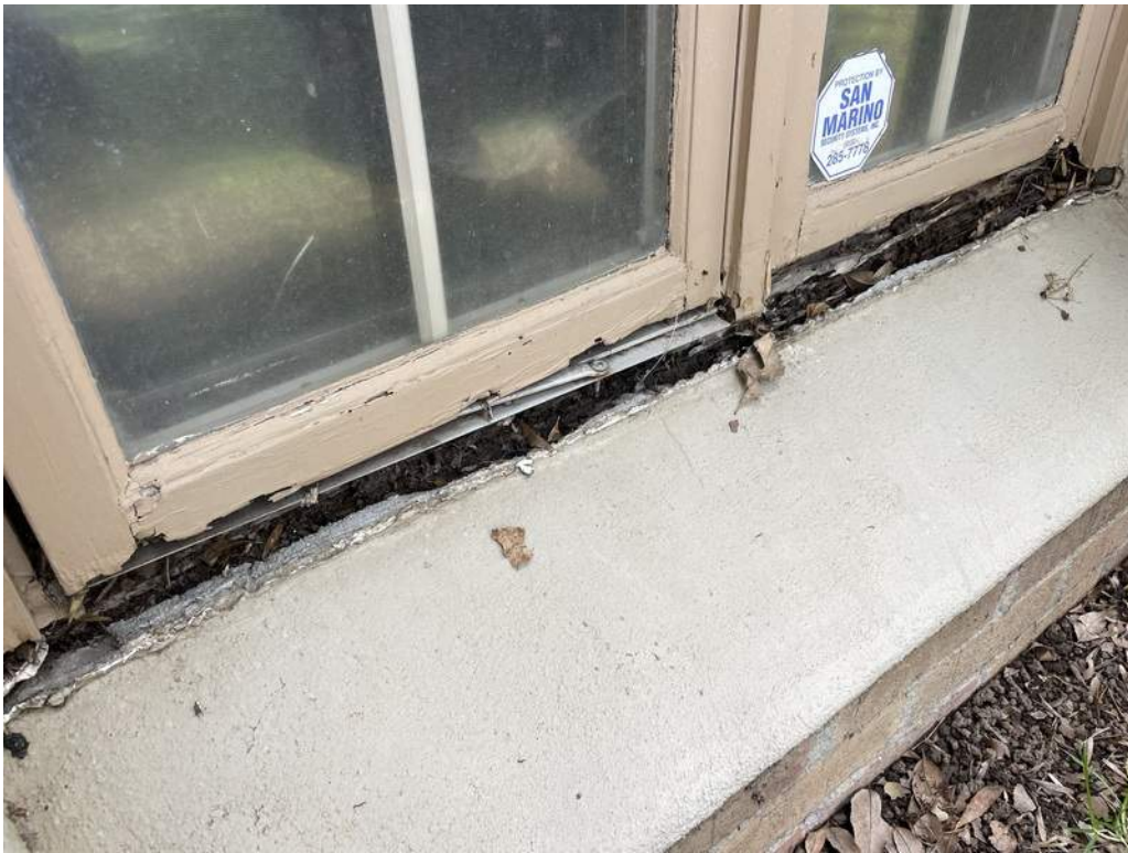
39 - Rotted and deteriorated window sill.
