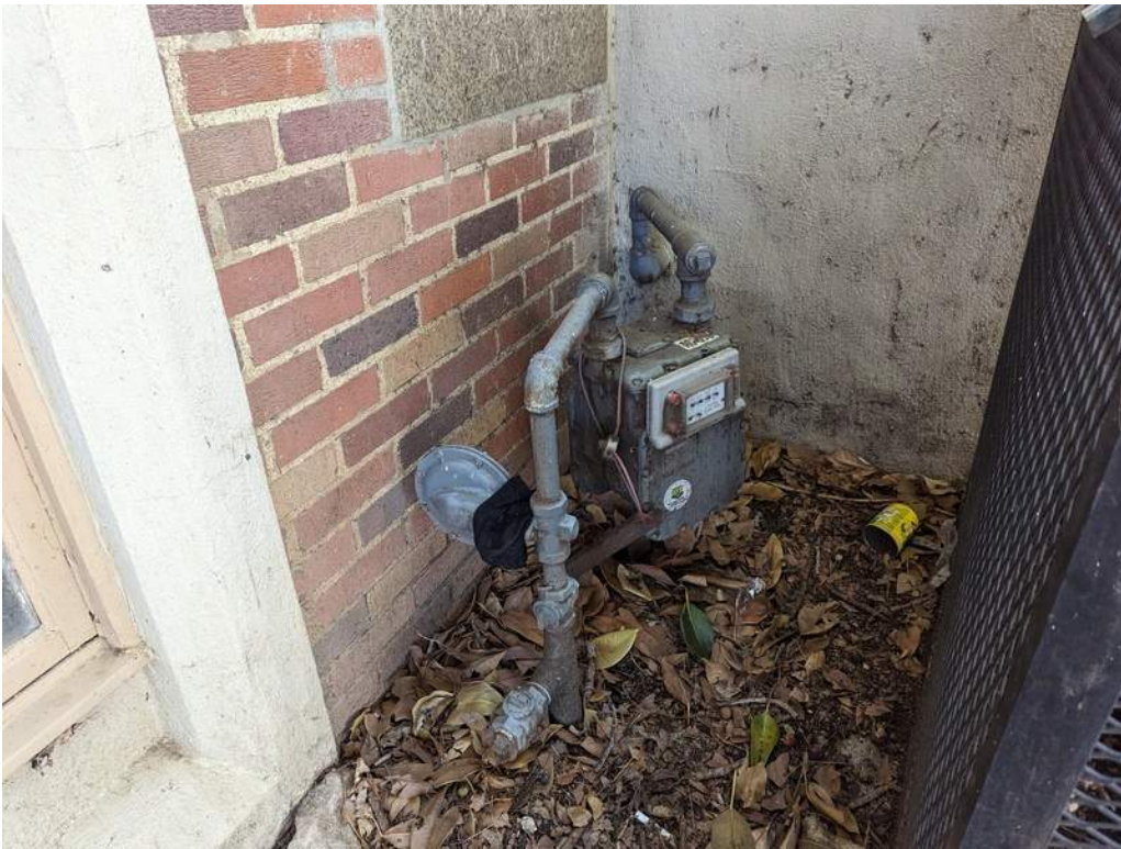
82 - Natural gas service with no seismic shut-off valve.
