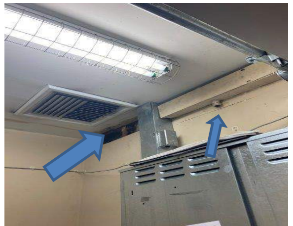
Elevator machine room HVAC. Note hole in drywall and abandon electrical fitting.
