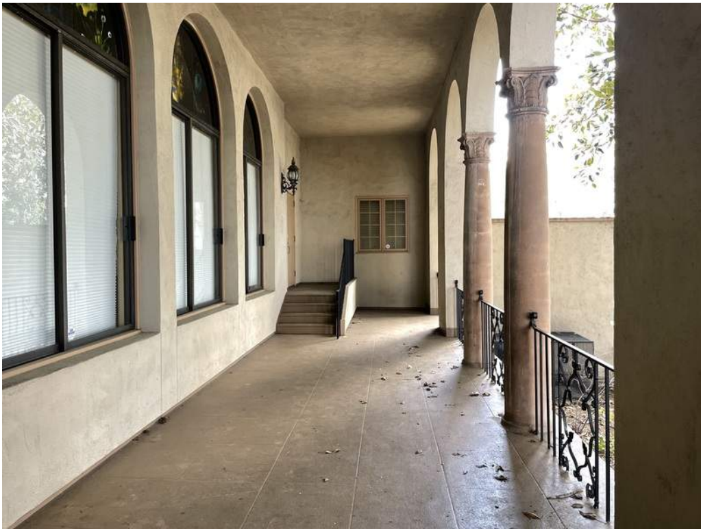
48 - Exterior balcony with fluid-applied waterproof traffic coating, dark anodized aluminum windows, cast stone columns, painted metal guardrail, and exterior cement plaster soffit.
