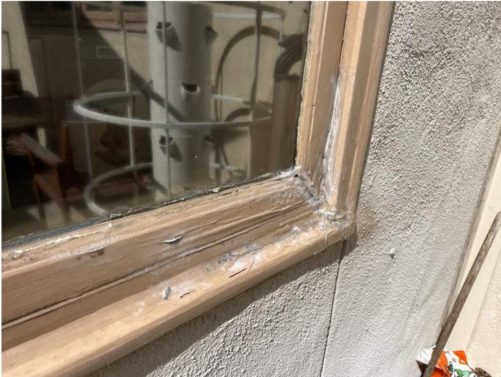
43 - Evidence of wood rot at the window frame; the material is soft and brittle. Film-forming sealer temporary repair noted.
