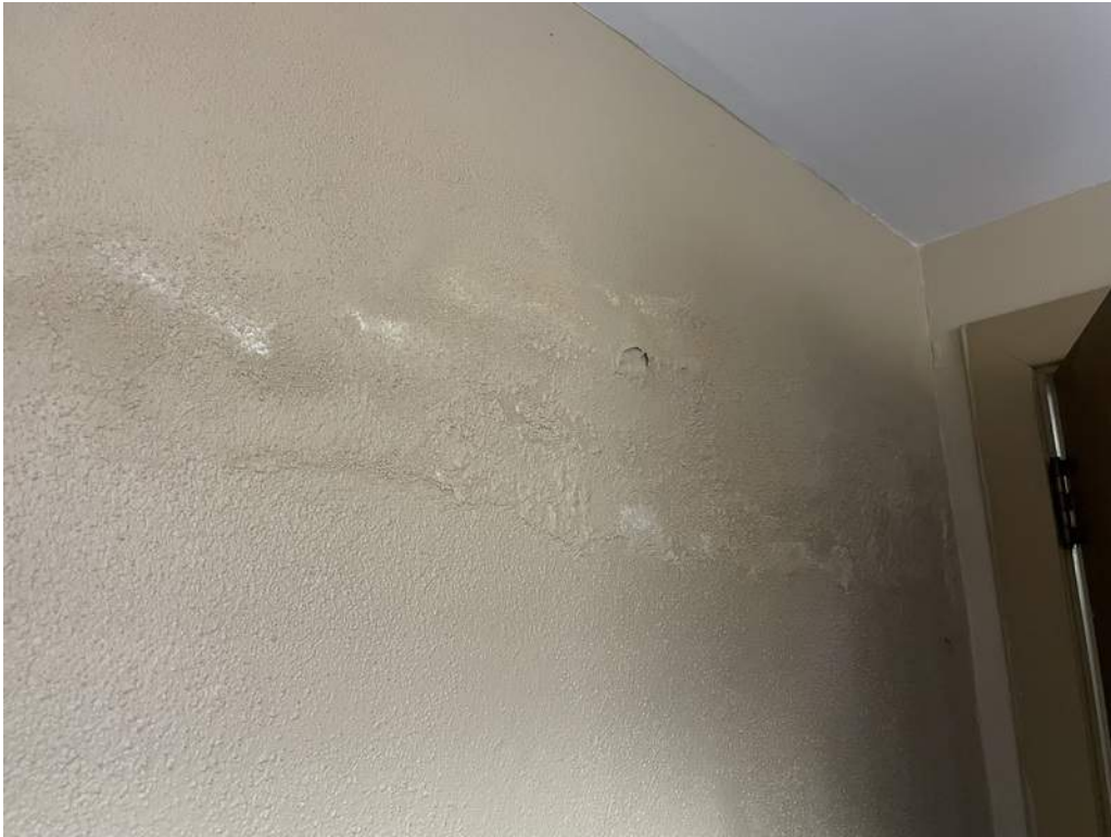
69 - Blistering paint and efflorescence observed in the staff work room.
