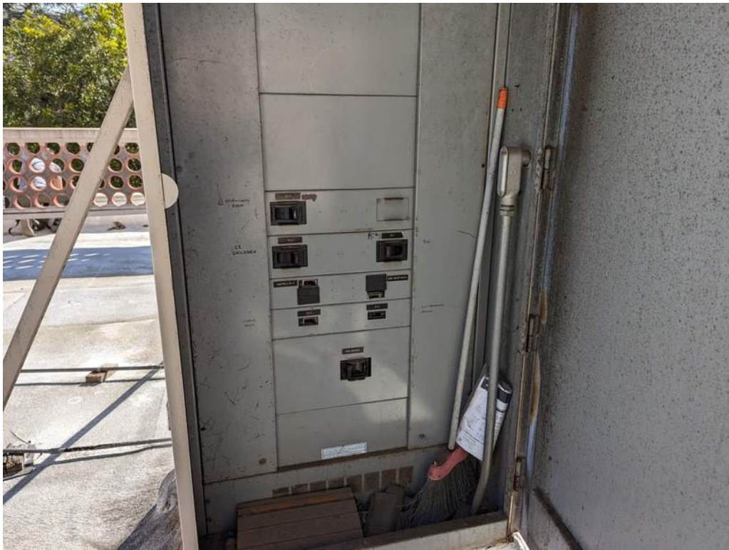
83 - Electrical panel in enclosure at the roof.
