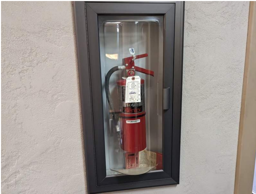
87 - Fire extinguisher in a recessed cabinet.
